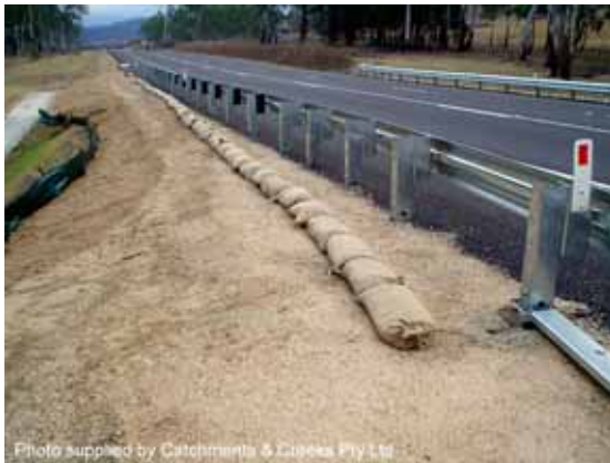
Photo 1 – Flow diversion berm used to minimise road runoff flowing down a steep, unstable section of the embankment
