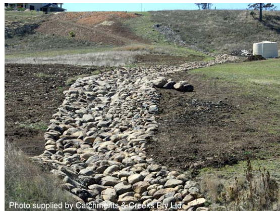
Photo 14 – Rock-lined catch drain
