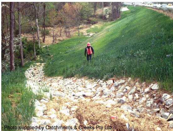
Photo 13 – Rock lined catch drain
