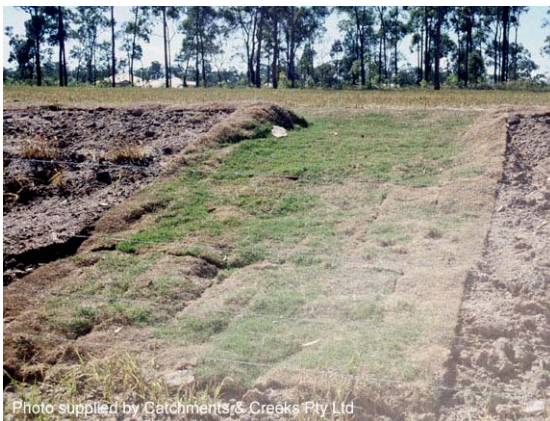
Photo 11 – Grass-lined chute (showing incorrect placement of turf)
