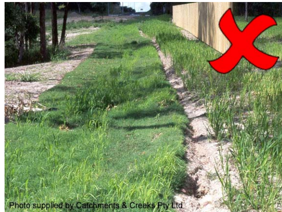
Photo 14 – Undesirable rilling along edge of turf caused by lateral inflows
