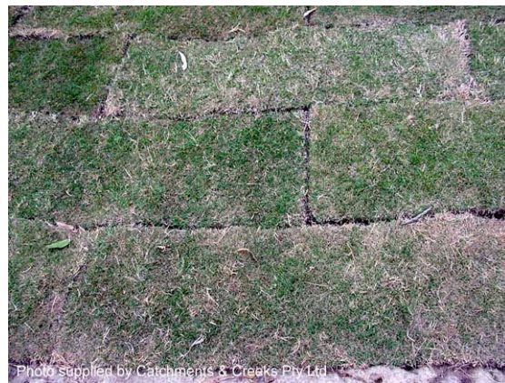
Photo 12 – Correct placement of turf (flow is from top of photo to bottom)
