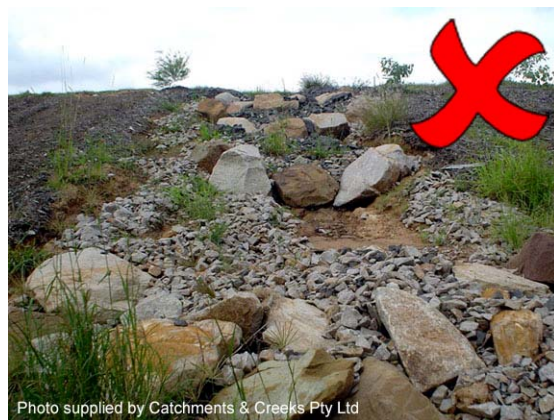
Photo 24 – Placement of a few large, anchor rocks down a steep slope will not help stabilise adjacent, under-sized rocks, and will likely cause flow diversion
