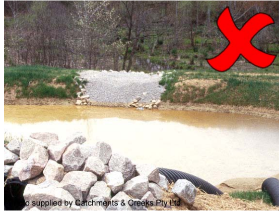
Photo 20 – Rock-lined spillway with poorly defined crest profile
