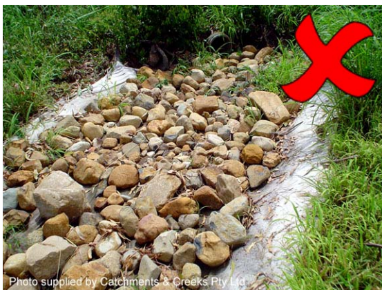
Photo 23 – Rounded rock can be significantly less stable than angular, fractured rock, especially when placed on steep slopes
