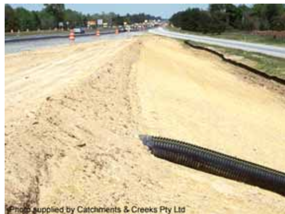
Photo 9 – Earth flow diversion bank used to direct runoff towards the Slope Drain
