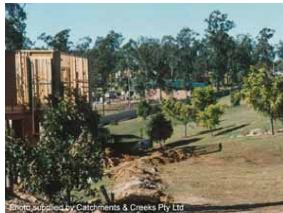
Photo 11 – Flow diversion bank up-slope of a building site – the bank also acts as a topsoil stockpile
