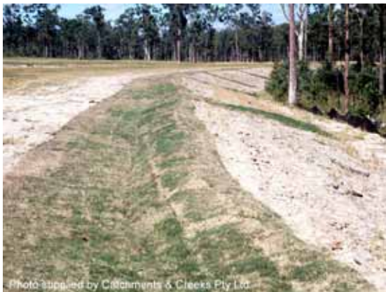
Photo 10 – Turf-lined flow diversion bank with grass-lined outlet chutes at regular intervals along the embankment
