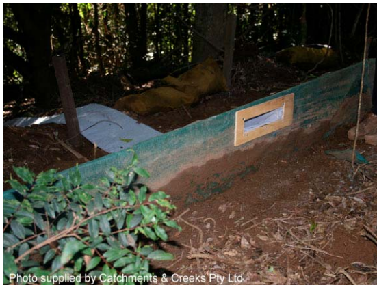
Photo 3 – Note filter tube inlet is raised above ground level to encourage ponding
