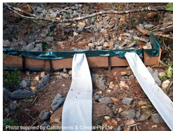
Photo 6 – Filter tube dam located at the base of a rock-lined chute
