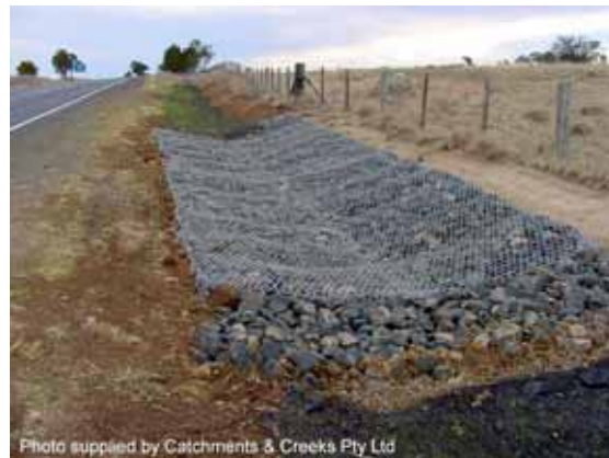
Photo 2 – Rock mattress-lined table drain (stormwater infiltration pit)
