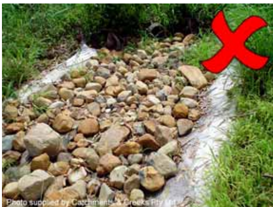
Photo 7 – Rounded rock can be significantly less stable than angular, fractured rock, especially when placed on steep slopes
