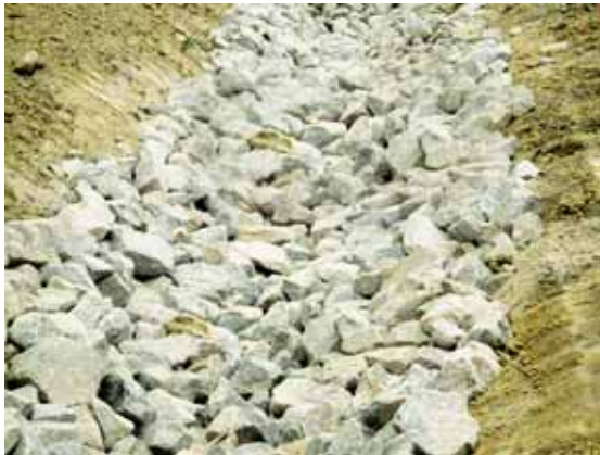
Photo 5 – Placement of the rock on the soil can result in erosion problems if significant lateral inflows occur
