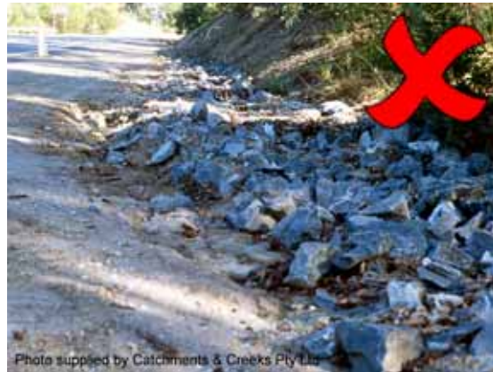
Photo 6 – In this example, placement of the rock has resulted in the rock-lined table drain being higher than the road shoulder
