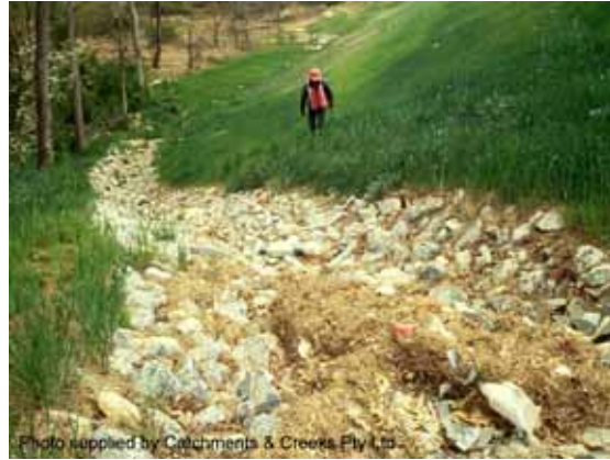
Photo 4 – Note how runoff from the adjacent batter is able to spill freely into the drain
