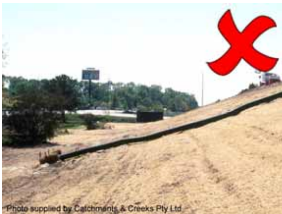
Photo 9 – Inappropriate flow release
