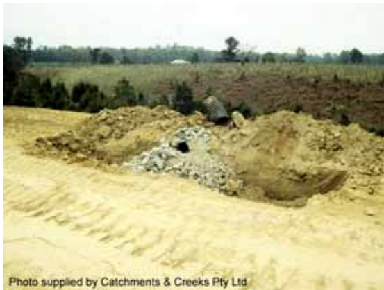
Photo 5 – Inlet sediment trap
