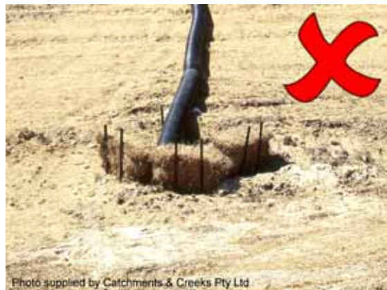
Photo 10 – Inappropriate flow release
