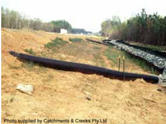
Photo 1 – Flexible, plastic slope drain
