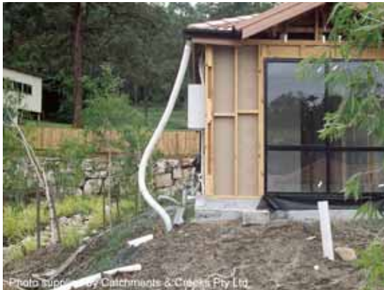
Photo 1 – Temporary downpipe (flexible pipe)
