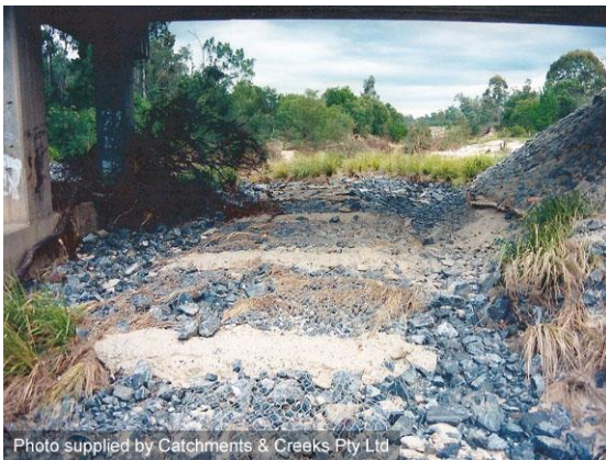
Debris on bridge pier, 1996
