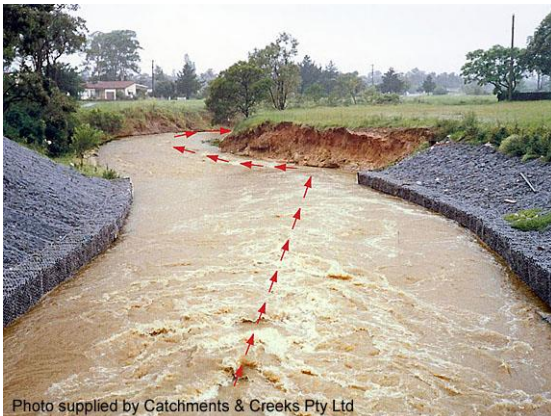
Flow jetting downstream of a culvert
