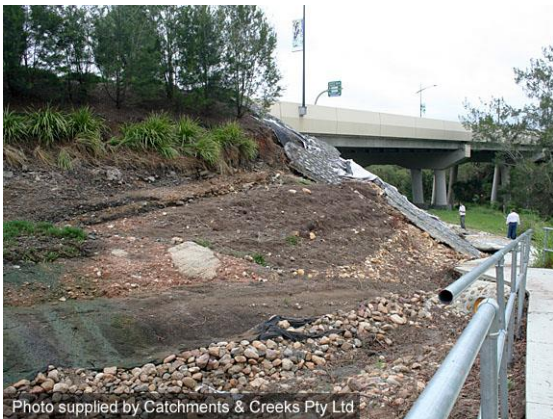
Flood damage upstream of bridge (Qld)
