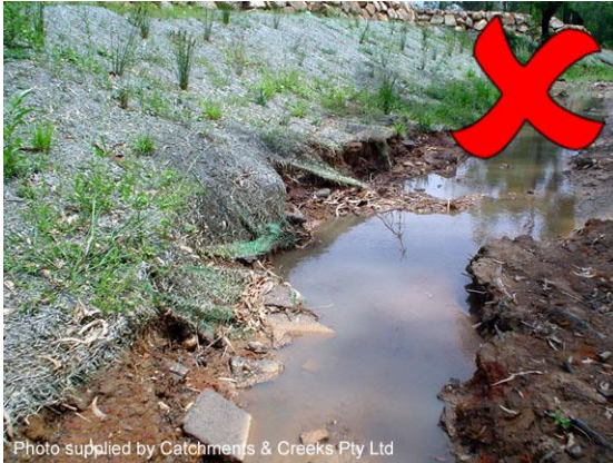
Erosion along toe of bank
