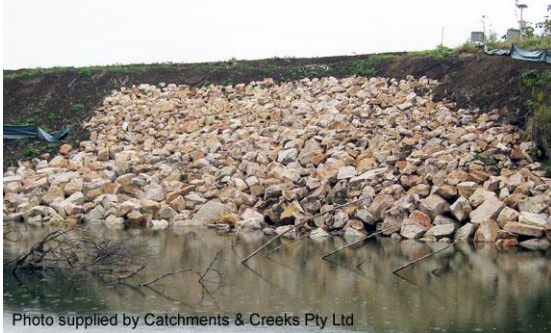
Poor aesthetics without vegetation cover
