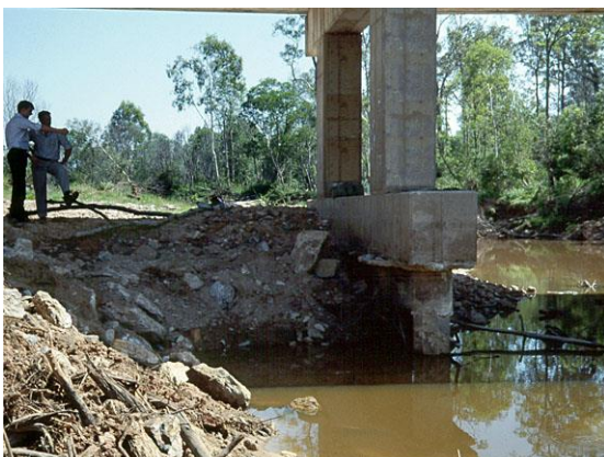
Local scour near a bridge pier (Qld)
