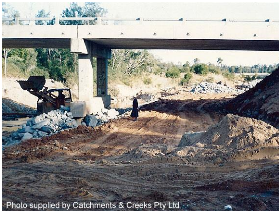
Vegetation cleared from under a bridge
