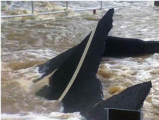
Pavement failure, Queensland, 2011
