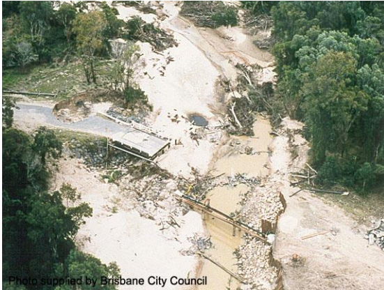
Bridge scour (Qld)
