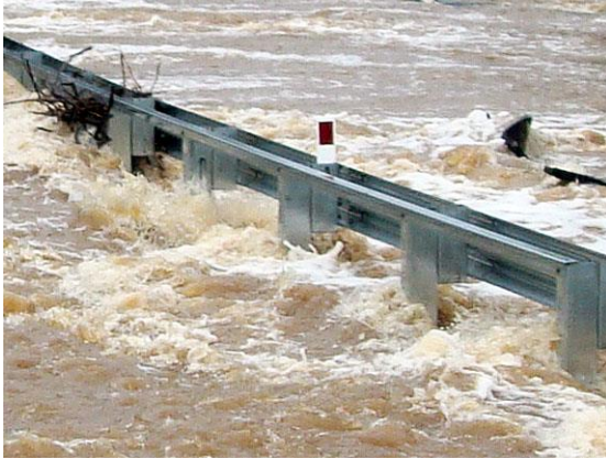
Floodwater passing under a guardrail
