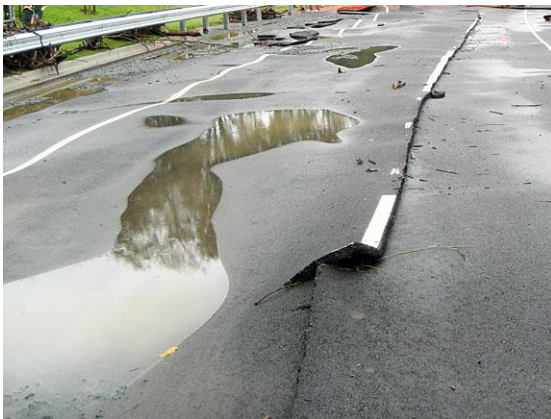
Pavement damage (Qld, 2010)
