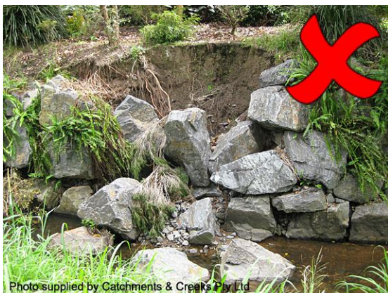
Failed boulder wall (Qld)
