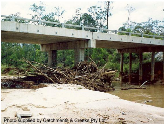
Debris raft trapped on a bridge pier
