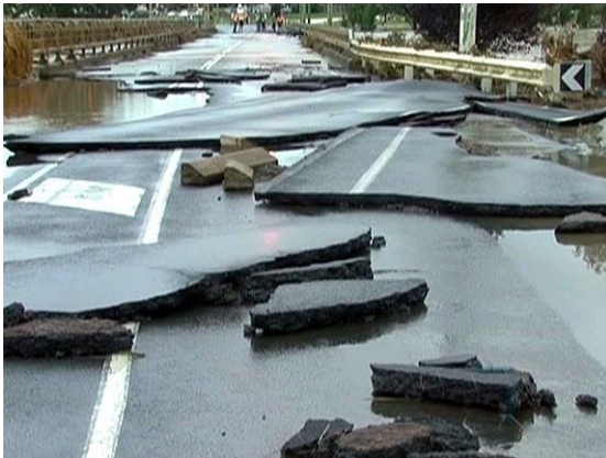
Road pavement lifted by floodwater
