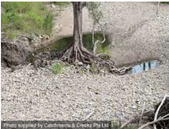
Scour pattern similar to a 'narrow' pier
