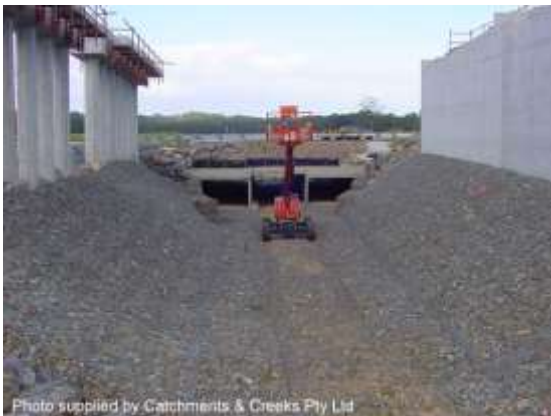
Non-vegetated rock mattresses (NSW)
