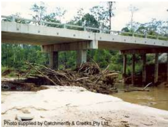
Debris raft trapped on a bridge pier
