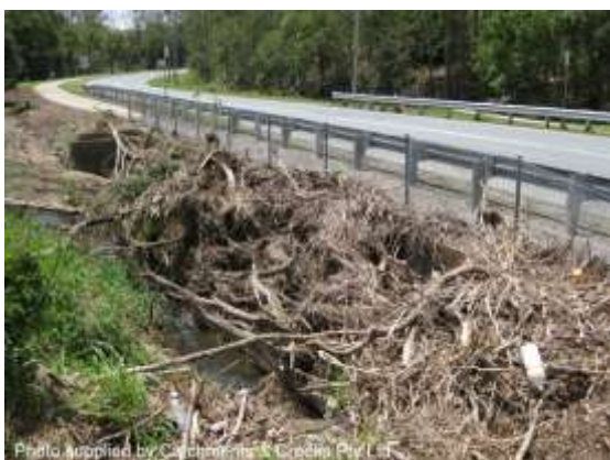
100% debris blockage of a road culvert
