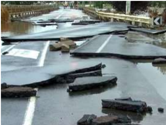
Road pavement lifted by floodwater
