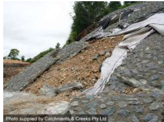
Same bridge post flood (2011)
