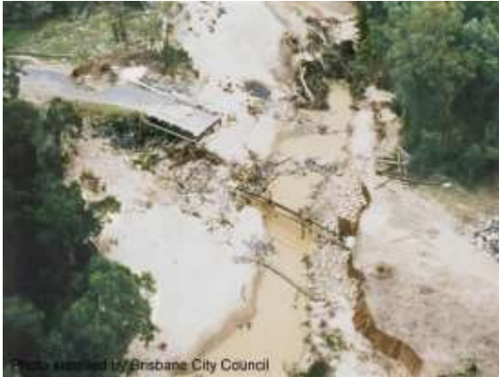
Flood damage to approach roads (Qld)
