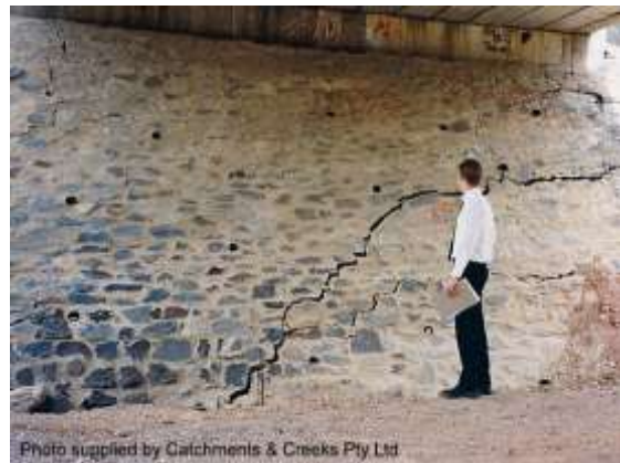
Damage to abutment stone pitching, 1991
