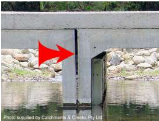
Open gap between culvert legs
