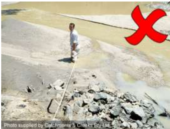
Weak sandy bed structure after a flood
