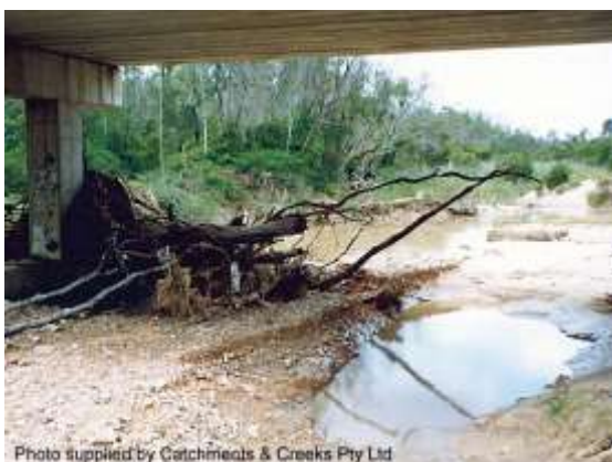
Scour hole formed by flood debris (Qld)
