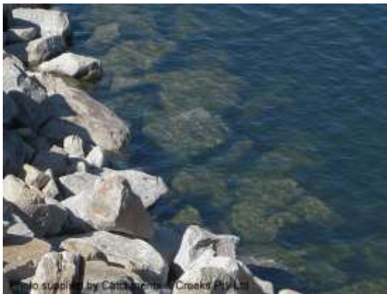
Open voids below permanent waterline
