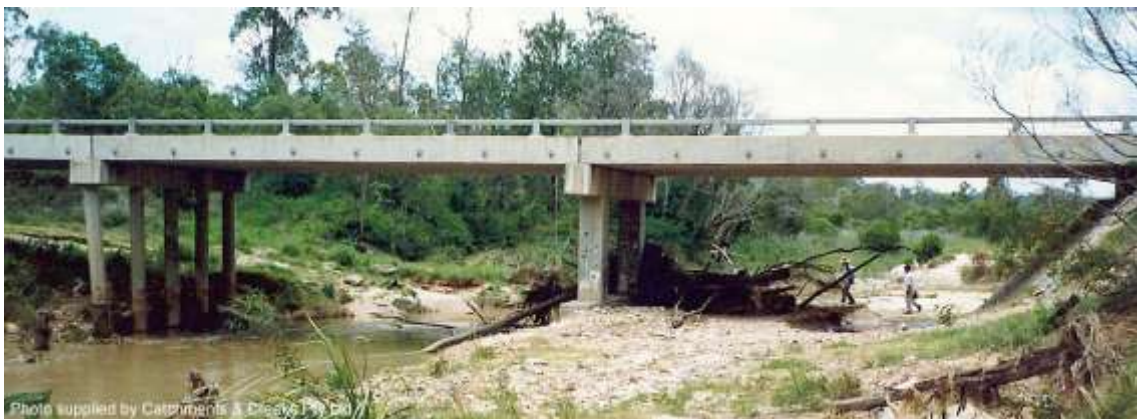
Post flood waterway scour, December 1991 (looking upstream)
