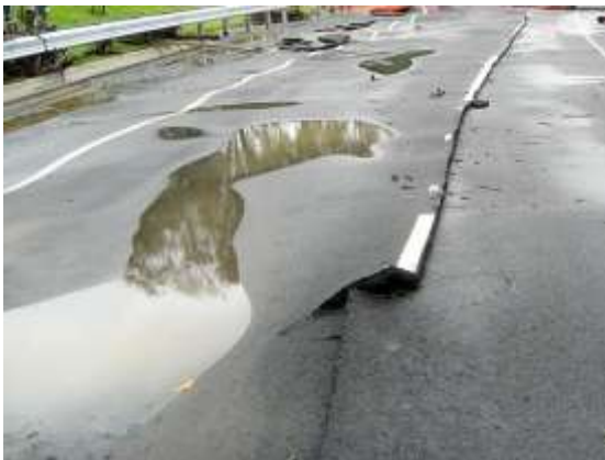
Pavement damage (Qld, 2010)
