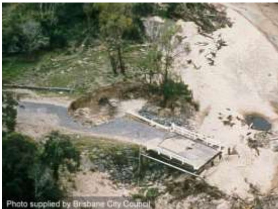
Flood damage to approach road
