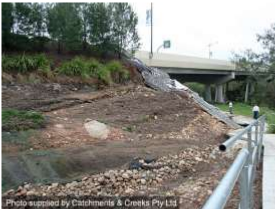
Flood damage upstream of bridge (Qld)
