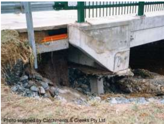
Flood damage to bridge abutment (Qld)
