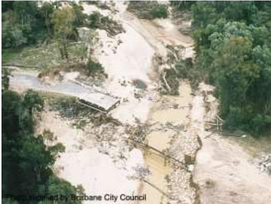
Bridge scour (Qld)
