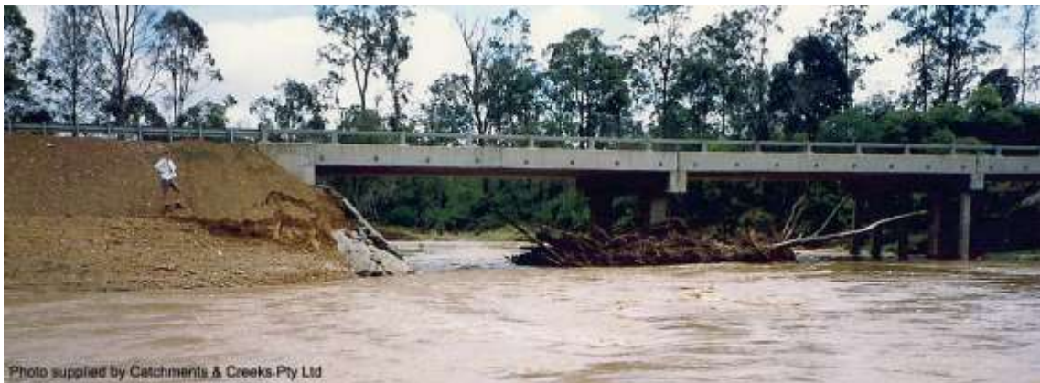
Debris raft captured by a bridge pier, 13 December 1991 (looking downstream)
