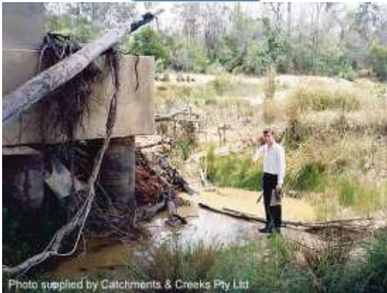
Degraded waterway channel (Qld)
