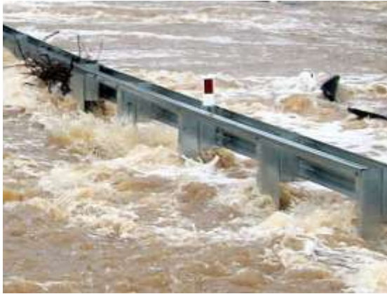
Floodwater passing under a guardrail
