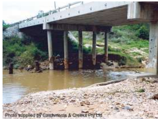
Post-1991 flood damage, east pier
