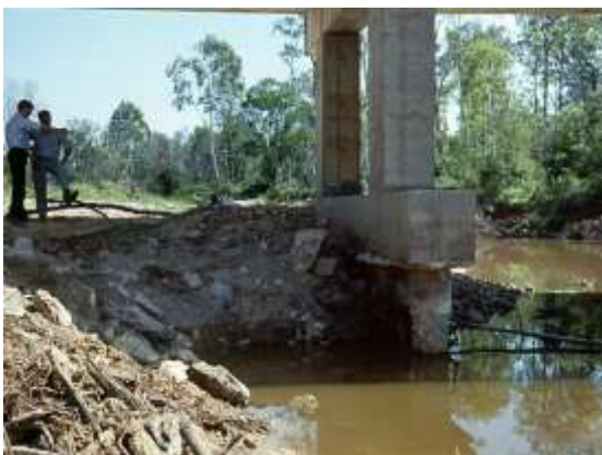
Local scour near a bridge pier (Qld)
