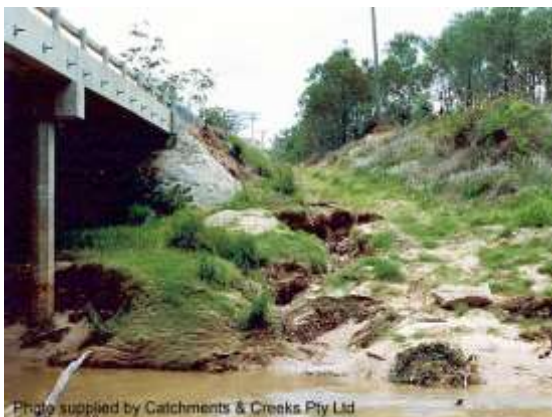
Diversion drain scour (1991)
