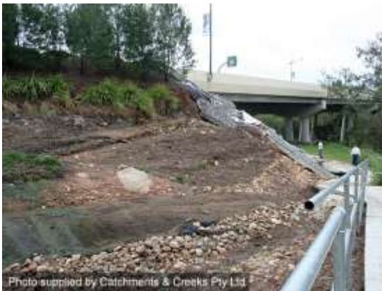
Flood damage to bridge abutment
