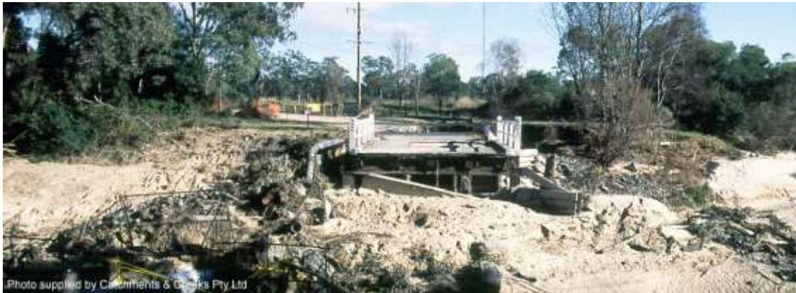
May 1996 flood damage (looking west)
