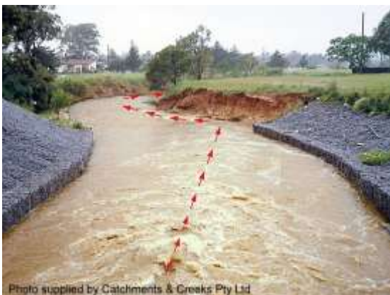
Flow jetting downstream of a culvert
