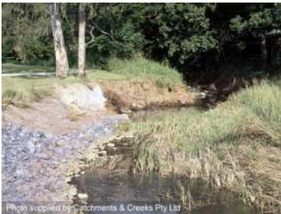
Bank erosion d/s of rock-stabilised bank
