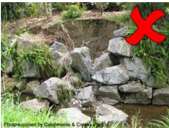
Failed boulder wall (Qld)
