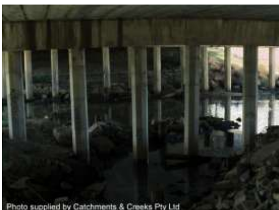
Poor light conditions under a bridge
