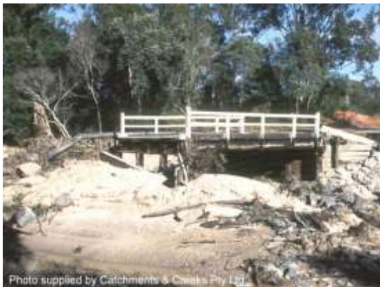
Timber bridge post May 1996 flood
