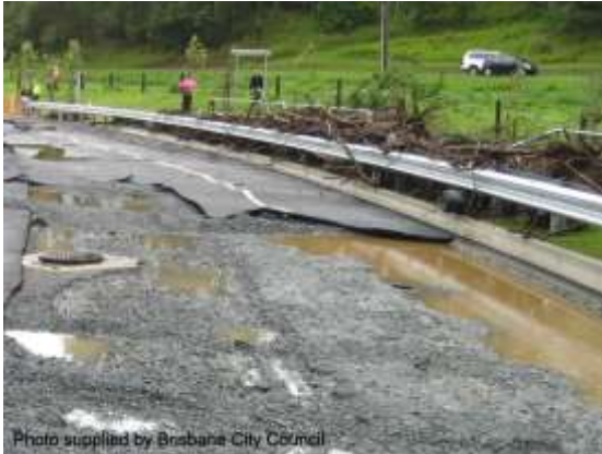
Pavement failure over a culvert
