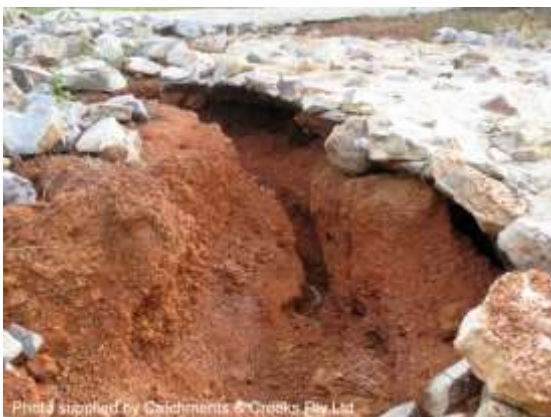
Failed stone pitching (NT)
