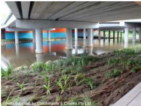
Adverse under-deck planting conditions
