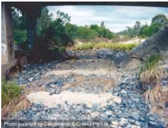
Debris on bridge pier, 1996
