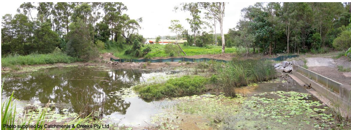
Photo supplied by Catchments & Creeks Pty Ltd Re-construction of creek bank, January 2011 (Kedron Brook in background)
