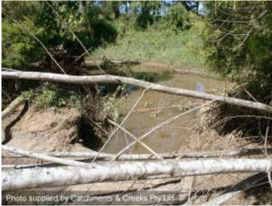
Post flood bank erosion (October, 2010)
