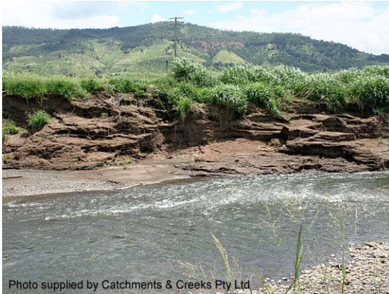
Soil scour caused by high velocity flows
