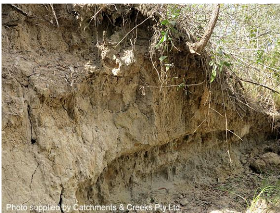
Bank undercutting (Qld)
