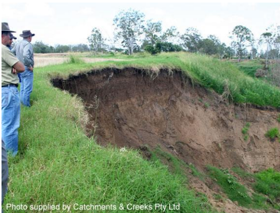
Bank slumping (Qld)
