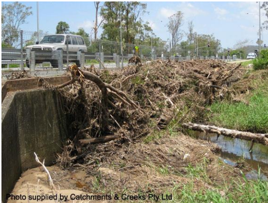
Debris blockage of a road culvert (Qld)
