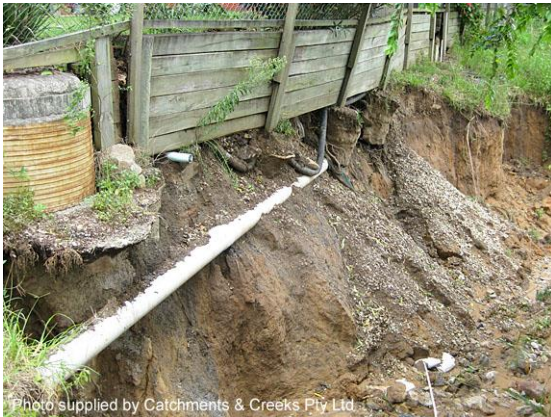
Urban creek erosion
