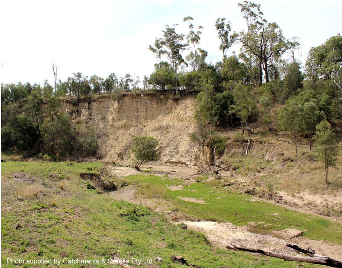
Bank undercutting on a channel bend adjacent a small bank slump, Miles, Queensland
