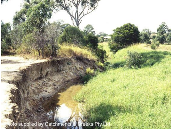
Photo supplied by Catchments & Creeks Pty Ltd Bank erosion (left) & sedimentation (right)
