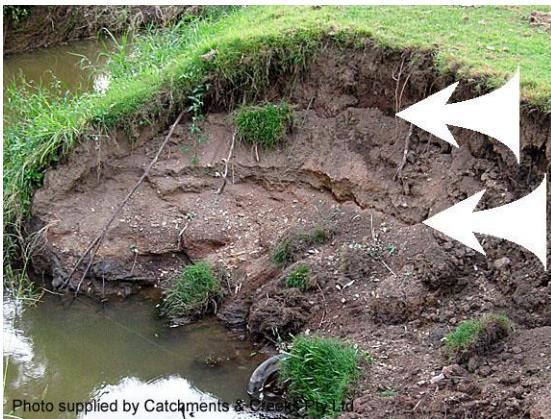
Bank slump (Qld)
