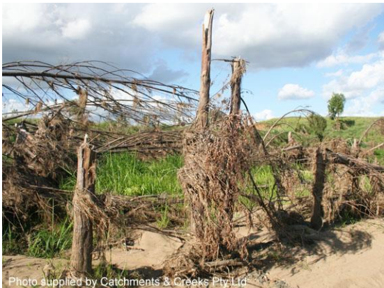
Flood damage to in-bank plants (Qld)
