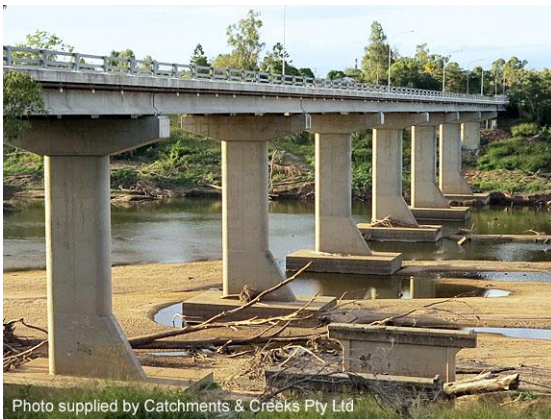
Localised bed scour around bridge piers
