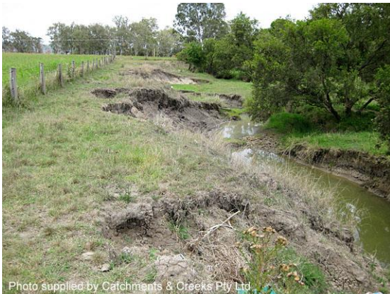
Lateral bank erosion (Qld)
