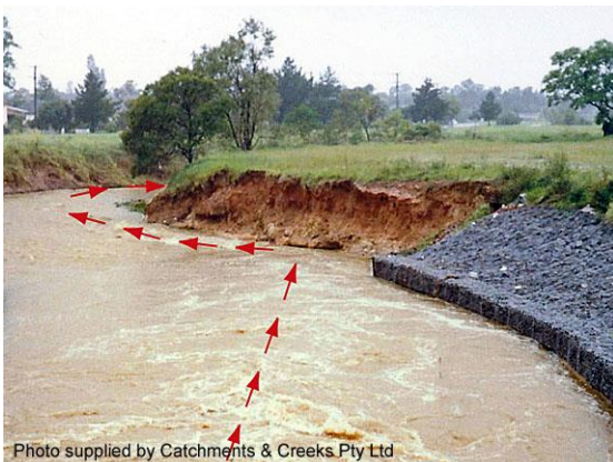
Velocity-induced soil scour (NSW)
