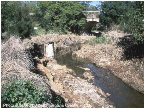
Bank erosion downstream of a sewer pit
