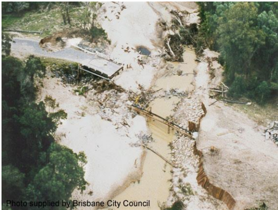
Severe streambed erosion (Qld)
