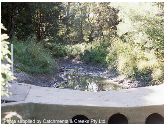
Scour hole downstream of a causeway
