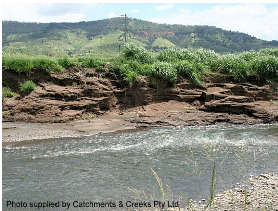
Bank scour (Qld)
