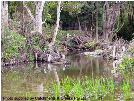
Artificial log groynes (NSW)
