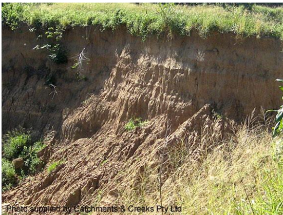
Bank slump (Qld)
