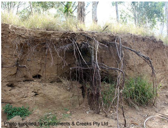
Tree roots exposed by undercutting
