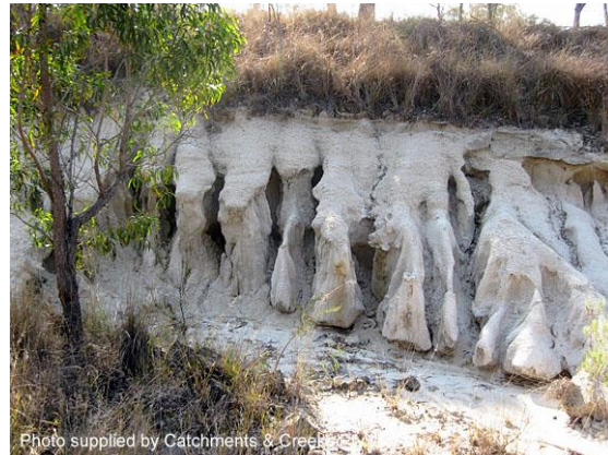
Fluting of a channel bank (Qld)
