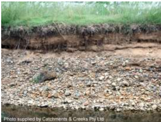
Gravel-filled creek bank (Qld)
