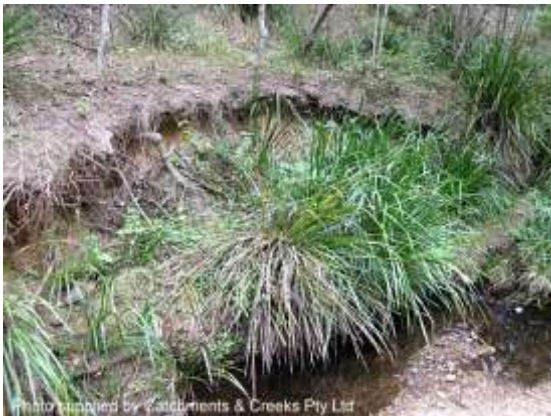
Bank slumping due to bed instability
