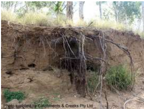
Tree roots exposed by undercutting
