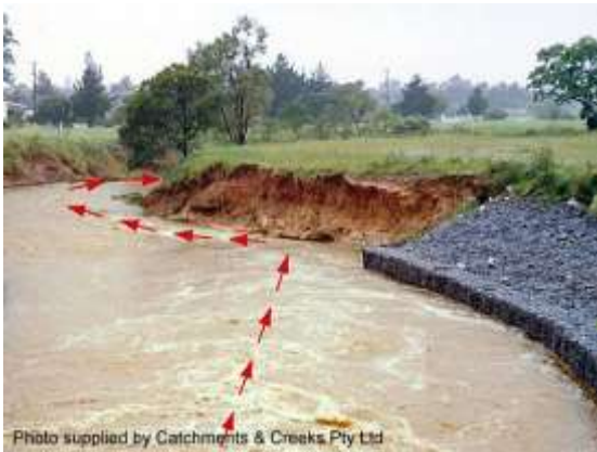
Velocity-induced soil scour (NSW)
