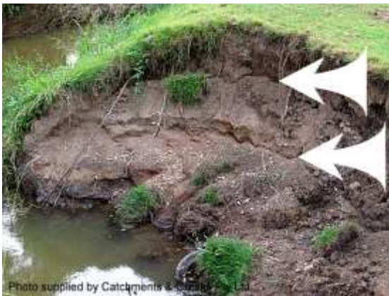
Bank slump (Qld)
