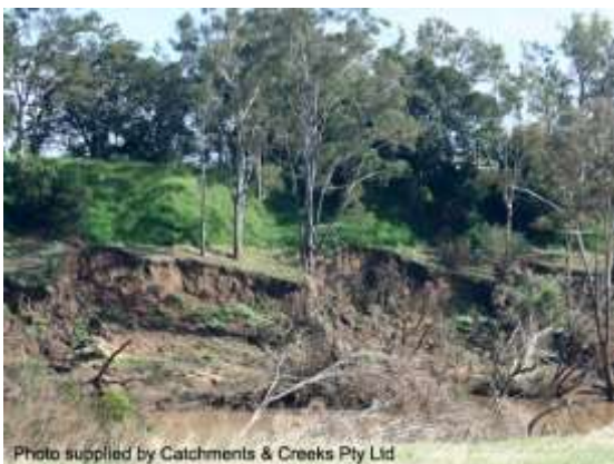
Flood damage to a river bank (Qld)
