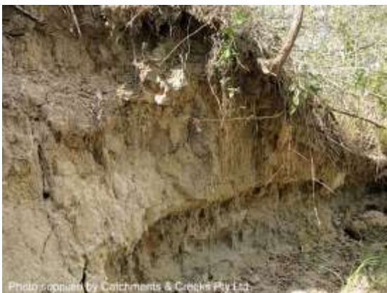
Bank undercutting (Qld)
