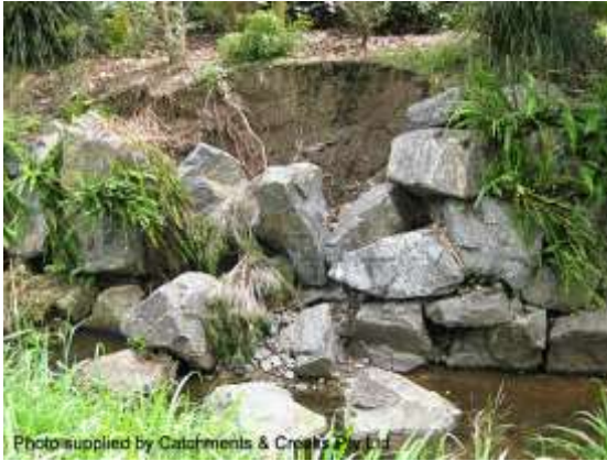
Failed rock stabilisation (Qld)
