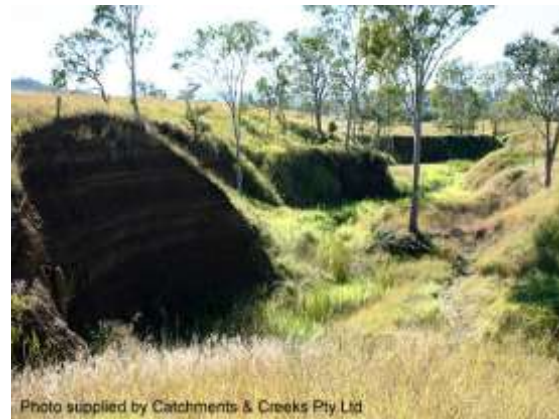
Photo supplied by Catchments & Creeks Pty Ltd Bank slumping along the north bank (Qld)
