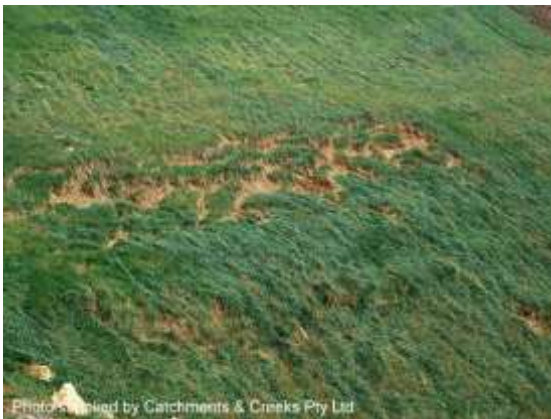
Gravity-induced stress cracks on a slope
