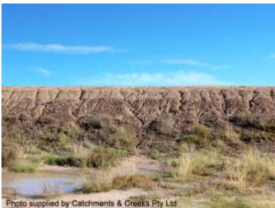
Rilling that extends to top of bank (Qld)
