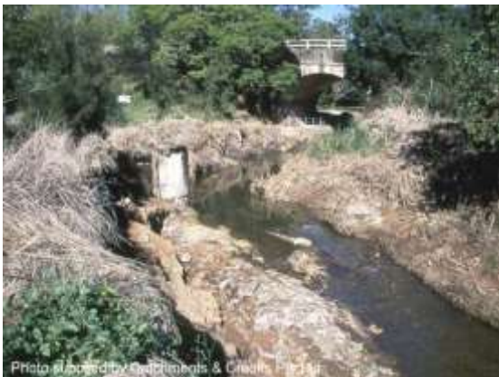
Bank erosion downstream of a sewer pit
