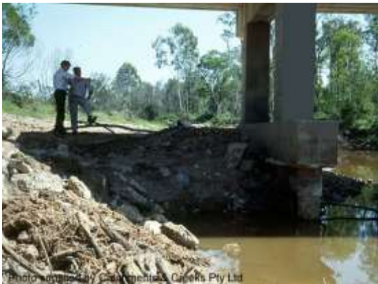
Erosion of bridge pier foundations (Qld)
