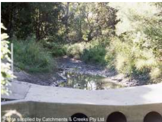
Scour hole downstream of a causeway
