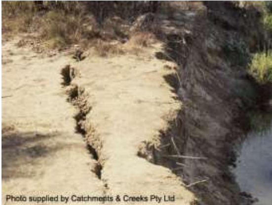
Crack in soil close to a creek bank (Qld)
