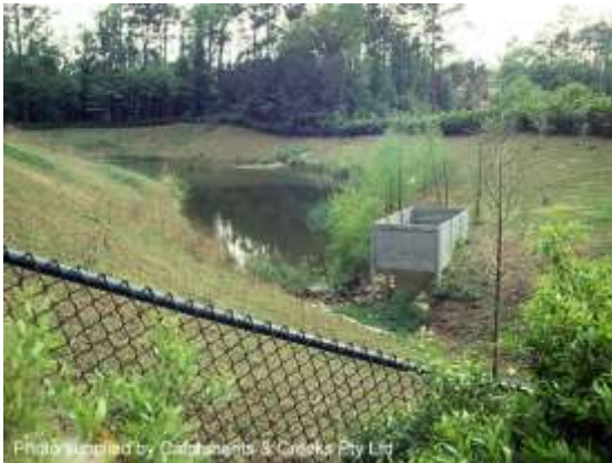
Stormwater retention basin (USA)
