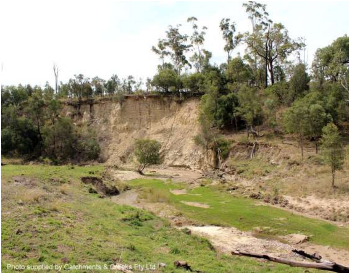
Bank undercutting on a channel bend adjacent a small bank slump, Miles, Queensland
