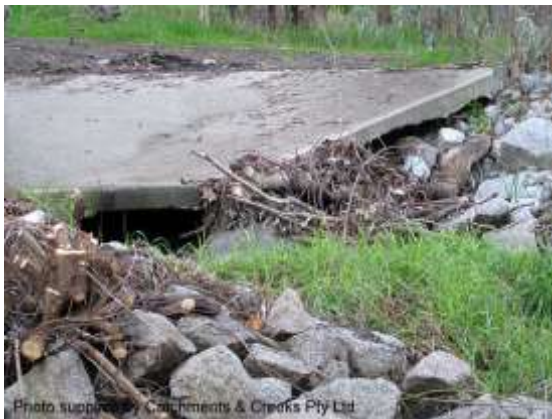
Rock displaced at end of concrete channel
