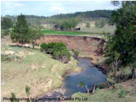
Bank erosion, Clarence River (NSW)
