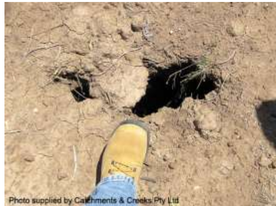
Tunnel erosion (Qld)
