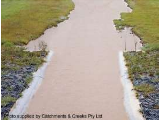
Channel erosion adjacent a concrete drain
