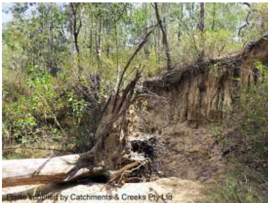
Fallen tree with adjacent bank damage
