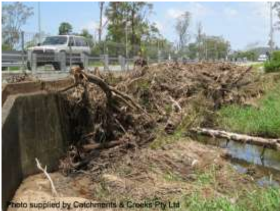
Debris blockage of a road culvert (Qld)
