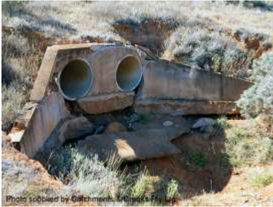
Photo supplied by Catchments & Creeks Pty Ltd Damage to a road culvert (NSW)
