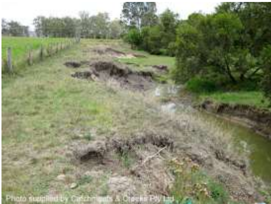
Lateral bank erosion (Qld)
