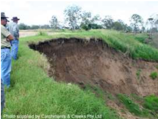
Bank slumping (Qld)
