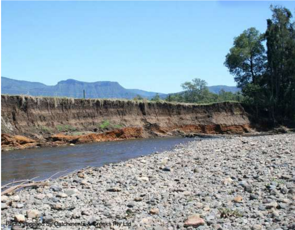
Warrell Creek, Aratula, Queensland (2011 flood damage on a channel bend)
