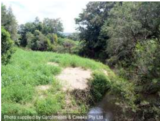
Sedimentation on inside of channel bend
