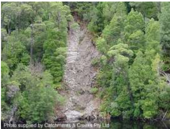
Bank slump in an unmodified waterway
