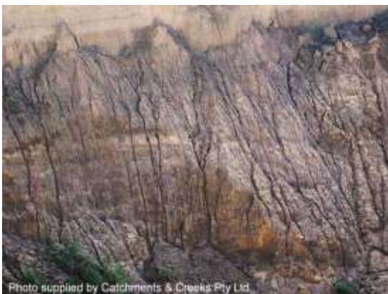
Minor runoff rilling (Qld)
