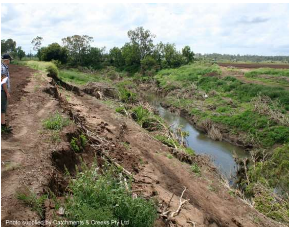
Tenthill Creek, Gatton, Queensland (2011 flood damage)
