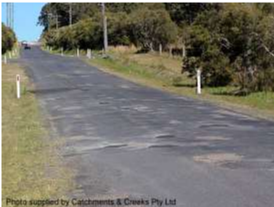
Heavily 'patched' bitumen road (NSW)
