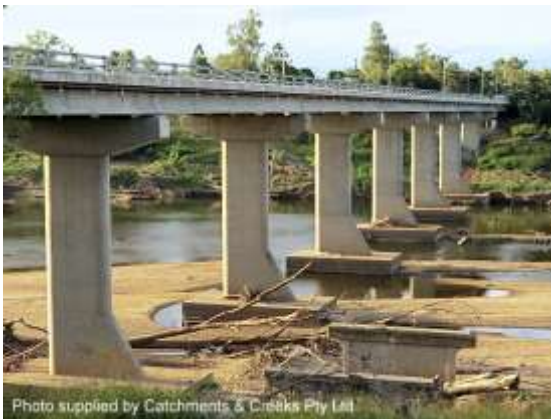
Localised bed scour around bridge piers
