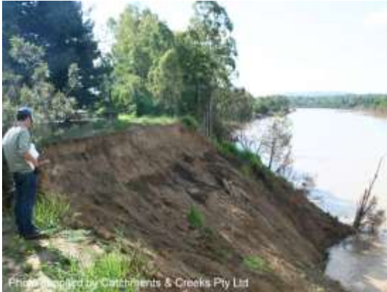
Bank failure, Brisbane River, 2011
