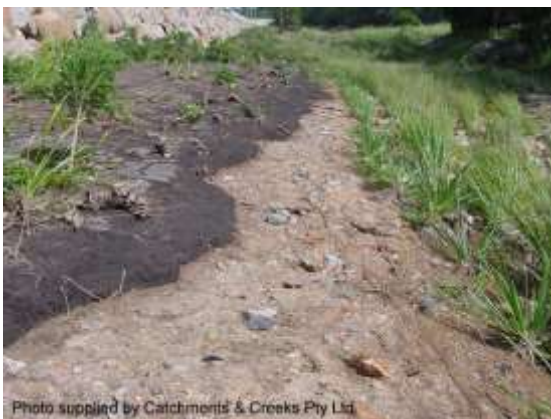
Flood damage to a grass-lined channel
