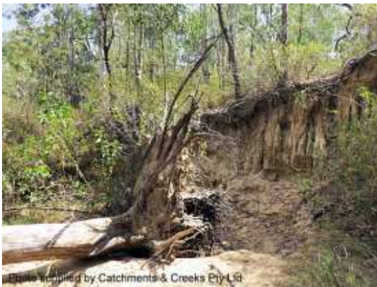
Bank erosion (Qld)
