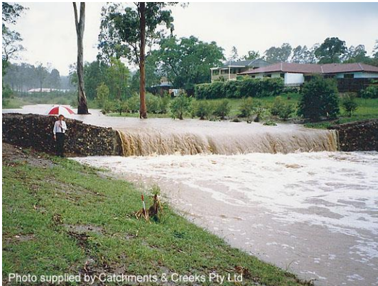
Photo supplied by Catchments & Creeks Pty Ltd Gabion drop structure (Qld)
