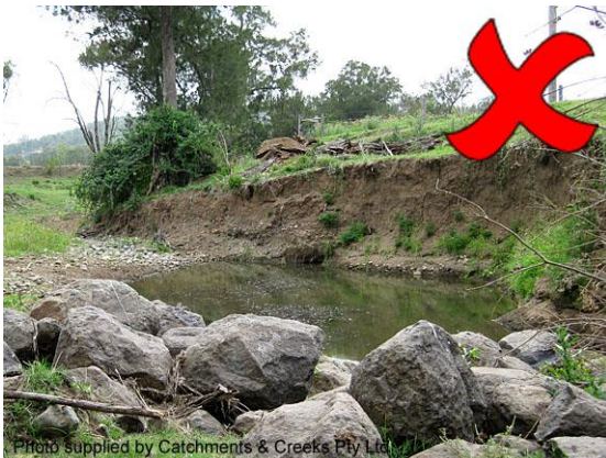
Erosion of adjacent creek bank
