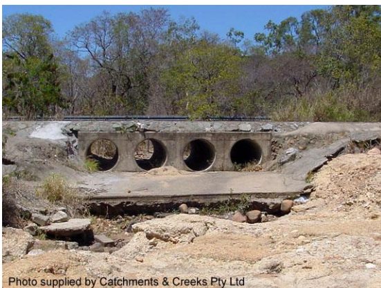
Bed level falling downstream of culvert
