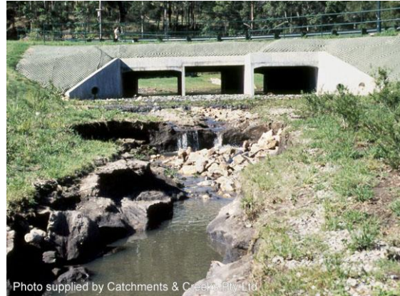
Failed placement of rock
