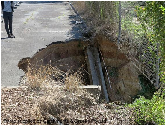
Bank erosion undermining a car park
