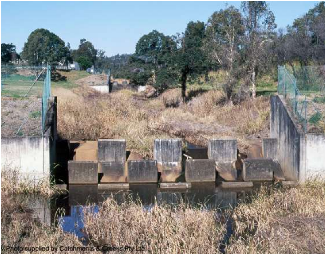
Baffled drop structure (Qld)
