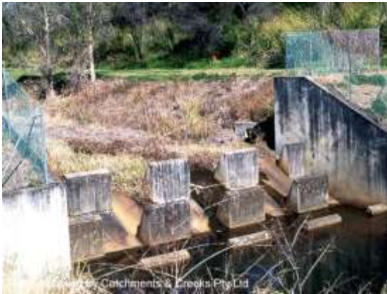
Baffled drop structure (Qld)
