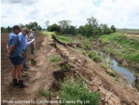
Bank scour (Qld)
