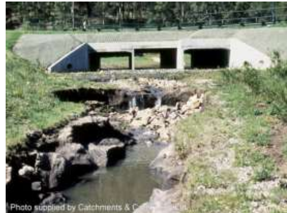
Failed placement of rock
