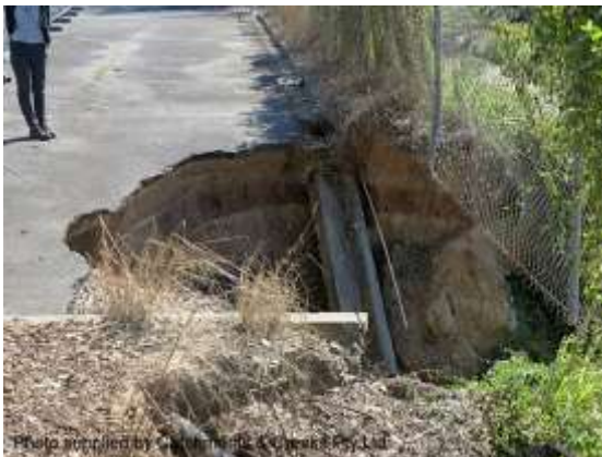
Bank erosion undermining a car park
