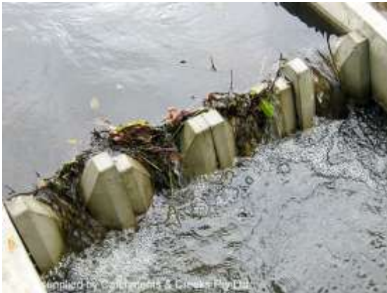
Debris blockage of fishway (Qld)
