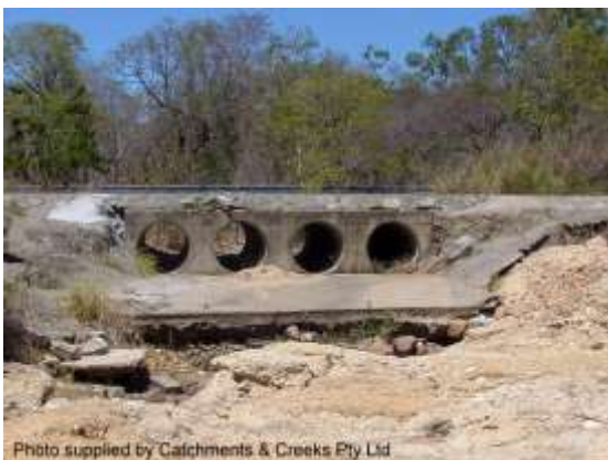
Bed level falling downstream of culvert
