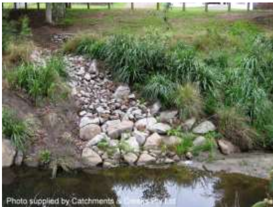
Stormwater inflow 'batter chute' (Qld)
