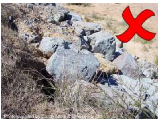
Erosion under rocks on a dispersive soil
