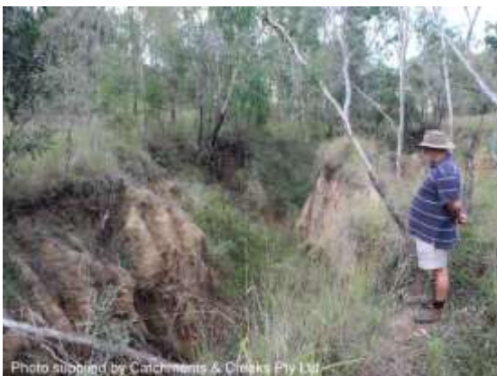
Gully erosion within a dispersive soil (Qld)
