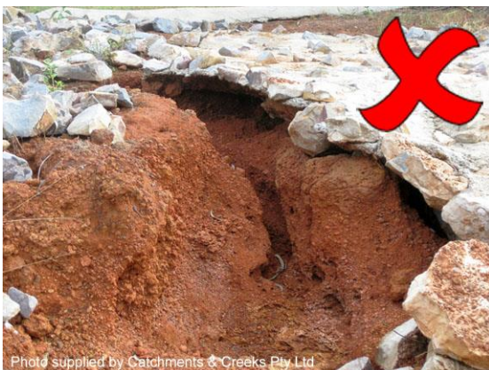
Erosion of a dispersive soil under concrete
