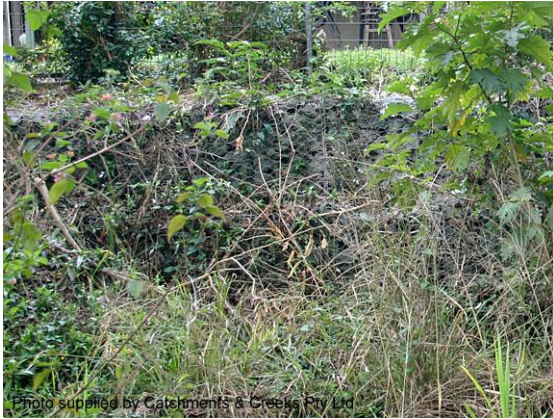
Gabion wall covered with weeds
