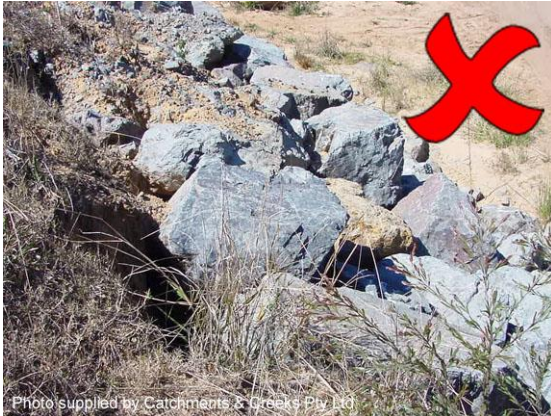
Tunnel erosion under rock stabilisation
