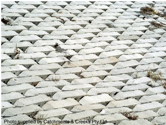
Flexible concrete mat bank protection
