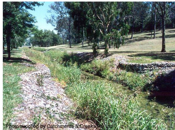
Weed invasion of the same drain (left)
