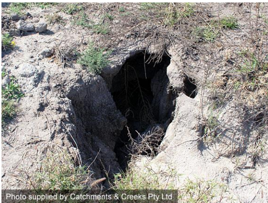
Tunnel erosion (Qld)
