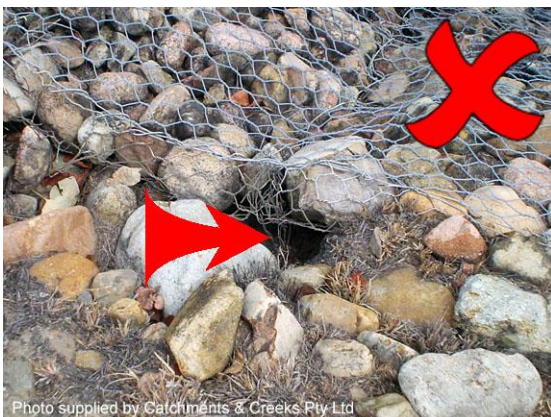
Tunnel erosion under rock mattress
