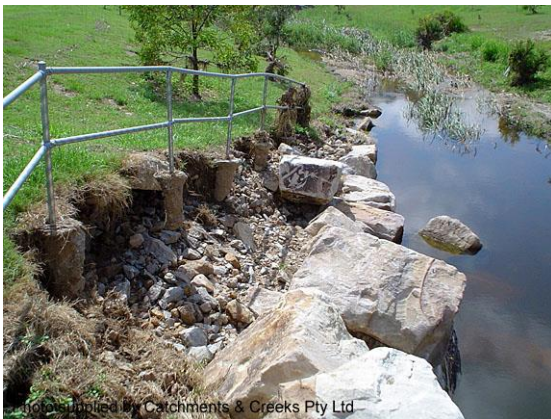
Soil erosion behind a retaining wall
