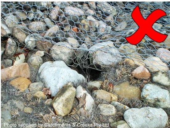
Tunnel erosion under a rock mattress
