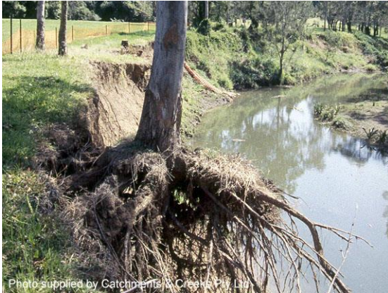
Exposed tree roots (Qld)
