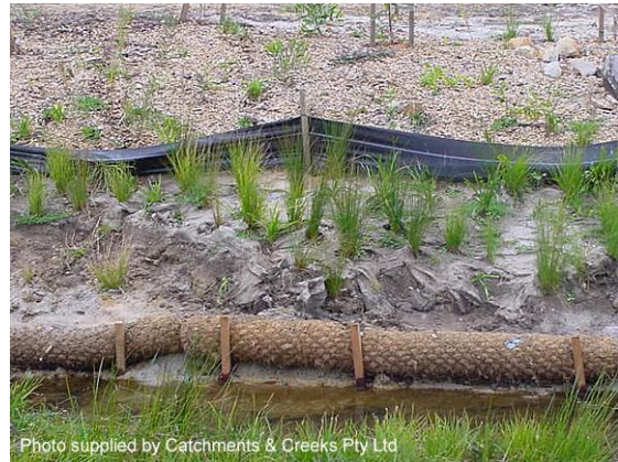
Note the soil scour behind geo logs
