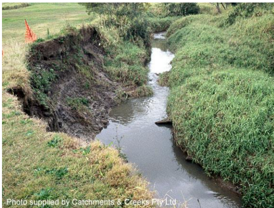
Erosion (left), grassed sediment (right)
