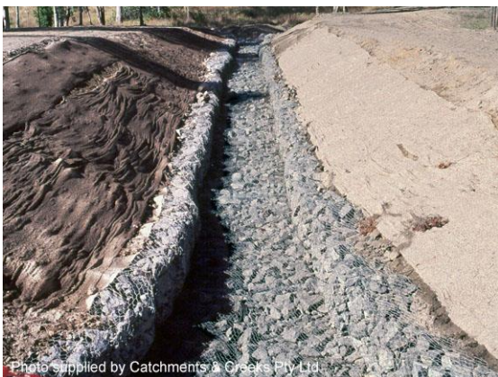
Non-vegetated rock mattress drain
