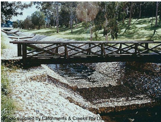
Non-vegetated rock mattress drain
