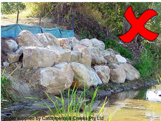
Poorly placed rocks on creek bank
