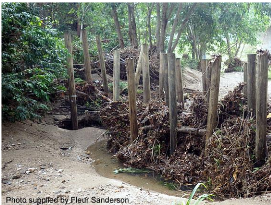
Erosion around the base of a pile field
