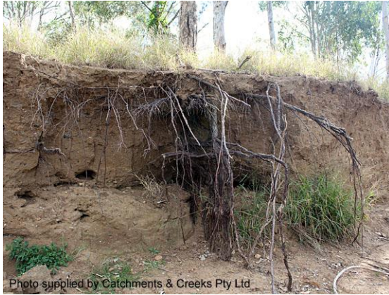
Bank undercutting (Qld)
