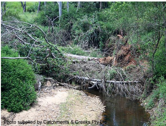
Photo supplied by Catchments & Creeks Pty Ltd Severe snag blockage (Qld)
