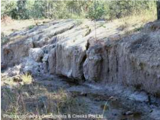
Dispersive soil erosion near the main bank
