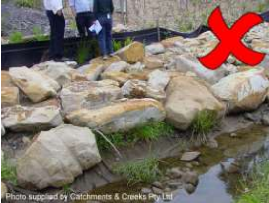
Undermining of toe rock
