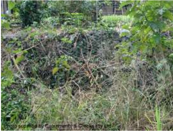
Gabion wall covered with weeds
