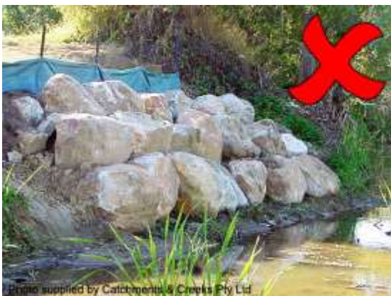
Poorly placed rocks on creek bank
