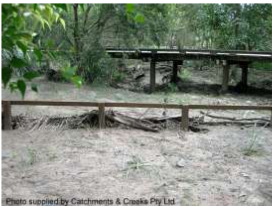
Overbank, timber, retard fence (Qld)
