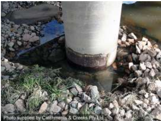
Scour around a bridge pier (Qld)
