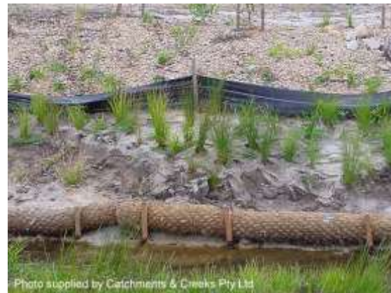
Note the soil scour behind geo logs
