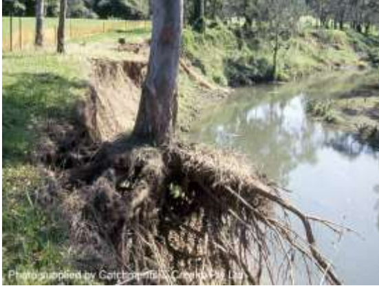
Exposed tree roots (Qld)
