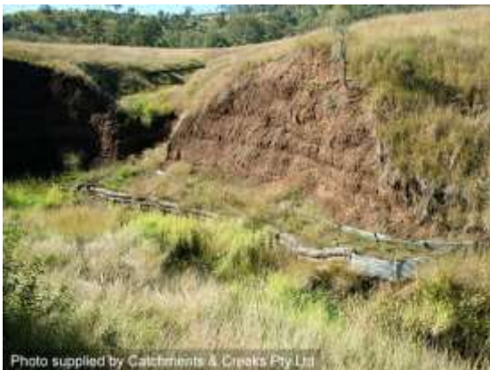
Retard fencing at the base of a bank slump
