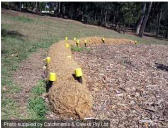
Geo log flow diversion bank (Qld)
