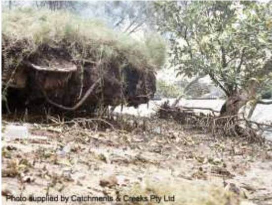
Fretting erosion (Qld)
