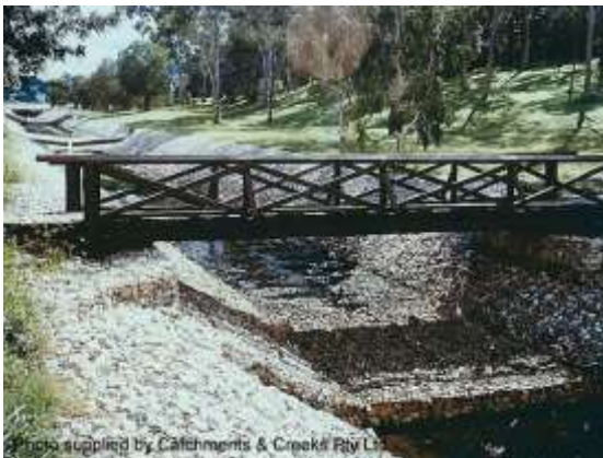
Non-vegetated rock mattress drain
