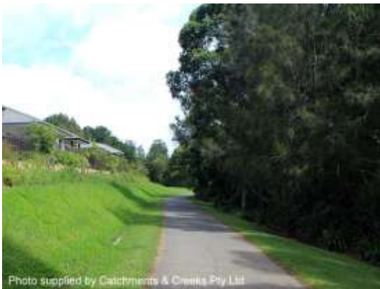
Constructed floodway (Qld)
