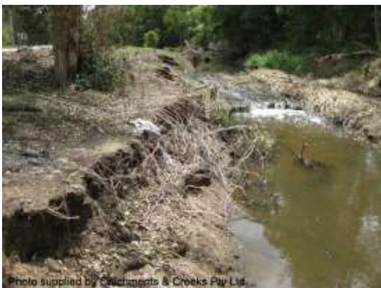
Bank erosion following weed removal
