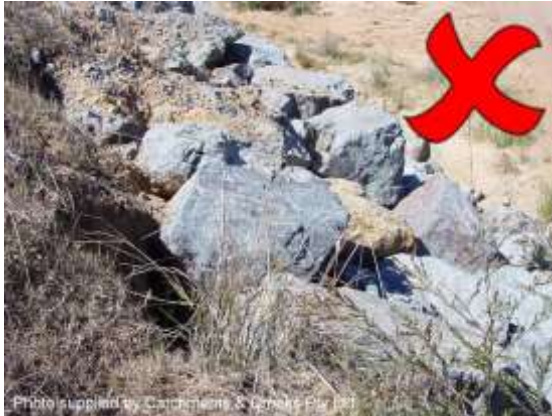
Tunnel erosion under rock stabilisation
