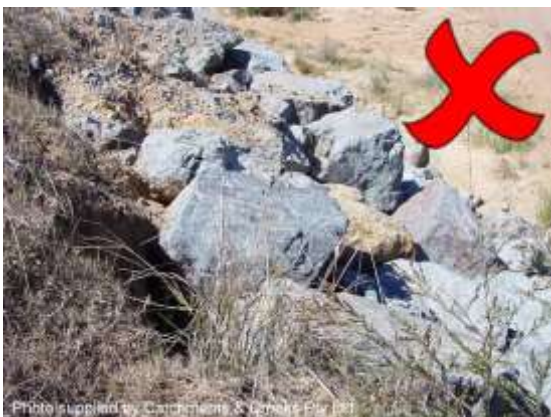
Erosion under rocks on a dispersive soil
