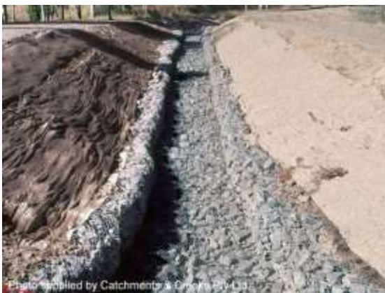
Non-vegetated rock mattress drain
