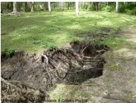
Initial stages of lateral bank erosion (Qld)
