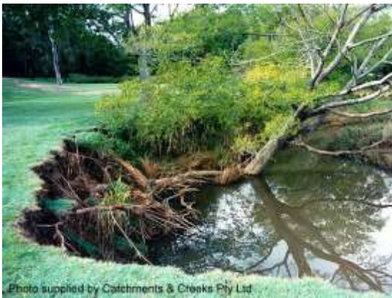
Bank erosion at a channel bend (Qld)
