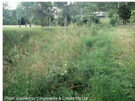
Weed invasion of the same drain (left)
