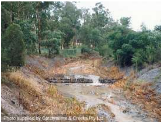
Weeds poisoned in a rock mattress drain
