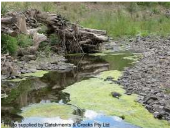
Scour hole downstream of log jam (Qld)
