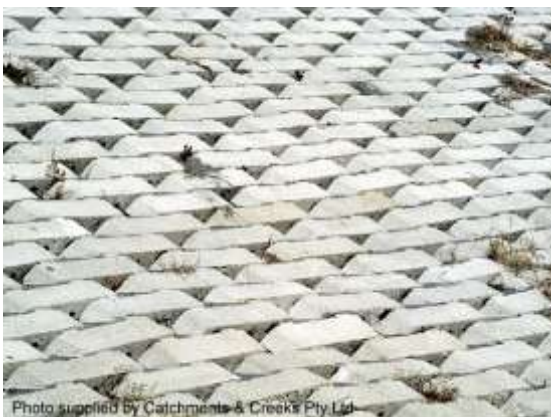
Flexible concrete mat bank protection
