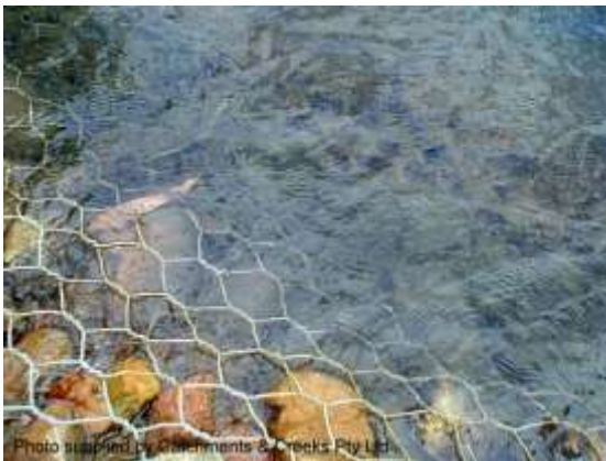
Rock mattress in a waterway environment
