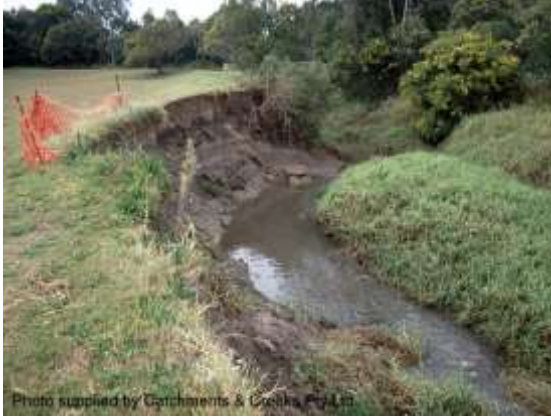
Bank scour (Qld)
