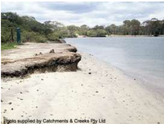
Wave-induced riverbank erosion (Qld)
