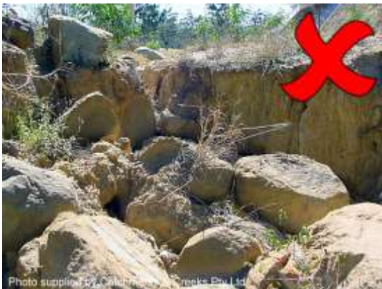
Collapsed dispersive soil bank
