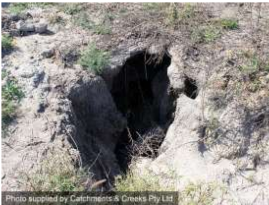
Tunnel erosion (Qld)
