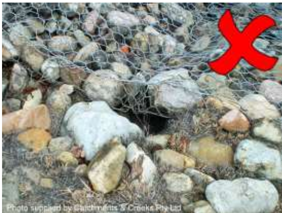
Tunnel erosion under a rock mattress
