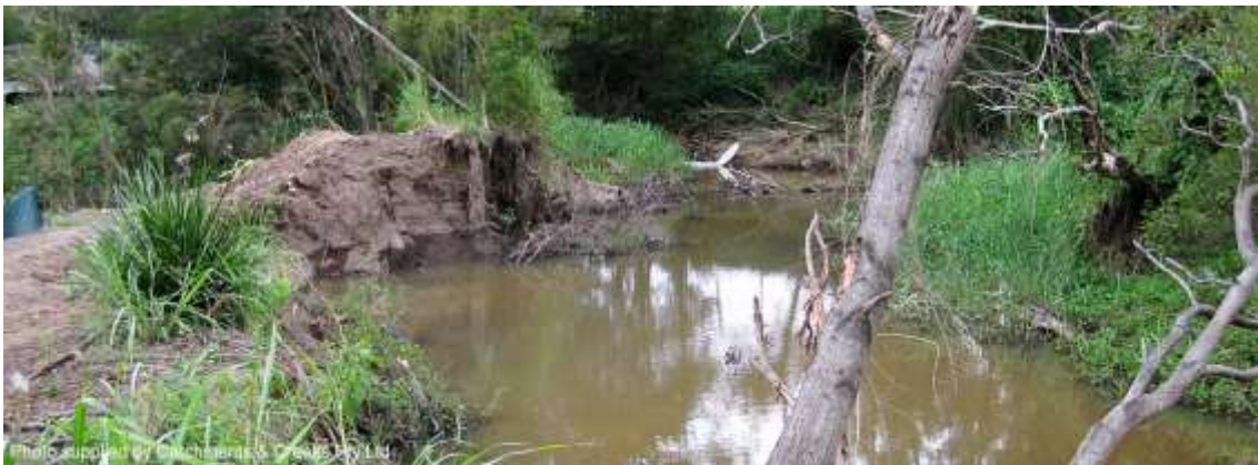
Post-flood eroded bank looking downstream (28/01/2011)
