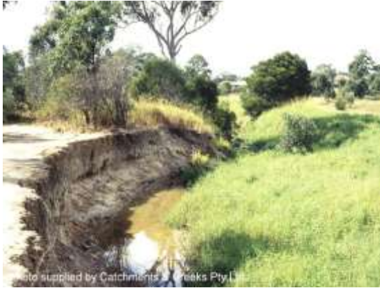
Bank erosion (left), sediment (right)
