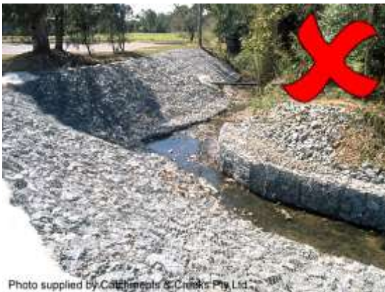
Undesirable erosion control outcome
