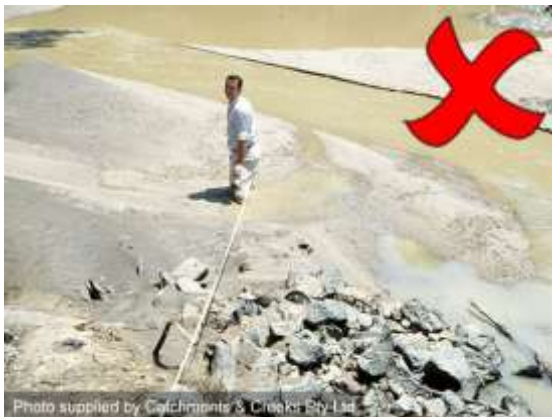
Weak sandy bed structure after a flood
