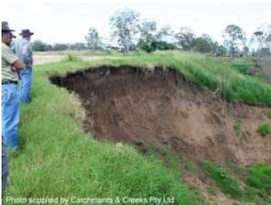
Bank slumping (Qld)
