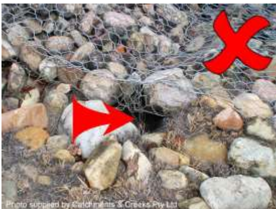
Tunnel erosion under rock mattress
