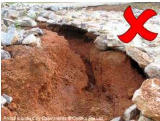
Erosion of a dispersive soil under concrete
