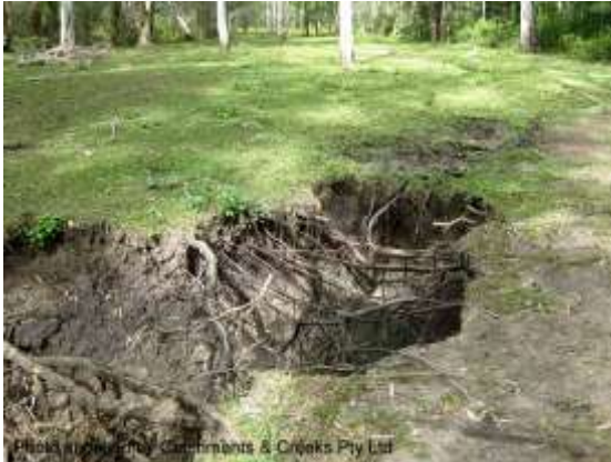
Initial stages of lateral bank erosion (Qld)
