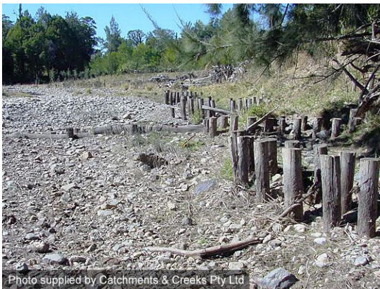
Pile field at the base of a creek bank (NSW)
