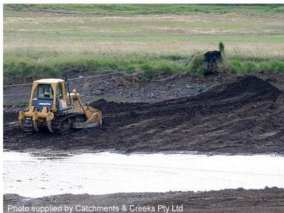
Gravel pushed up against the bank (Qld)
