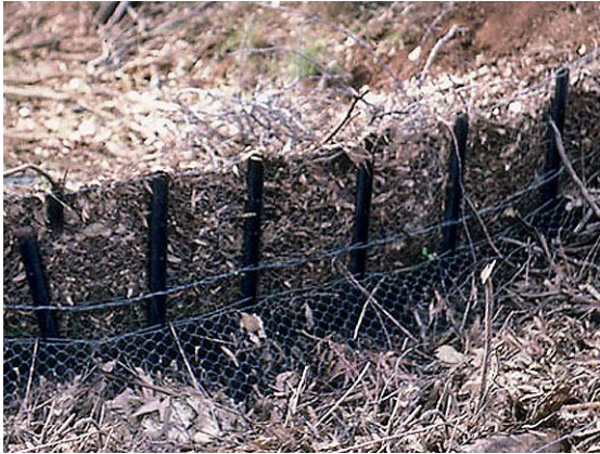
Mulch collecting on a wire mesh fence
