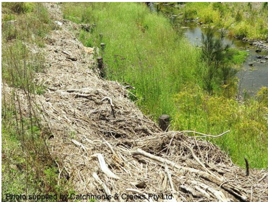
Brushwood toe protection (Qld)
