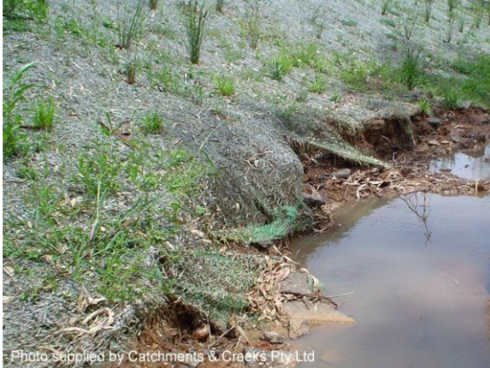
Toe erosion (Qld)
