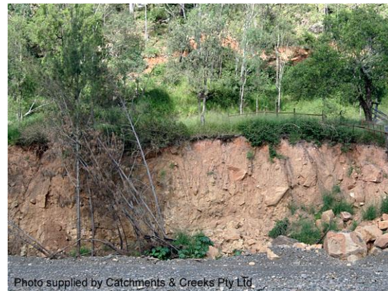
Post-flood bank erosion (Qld)
