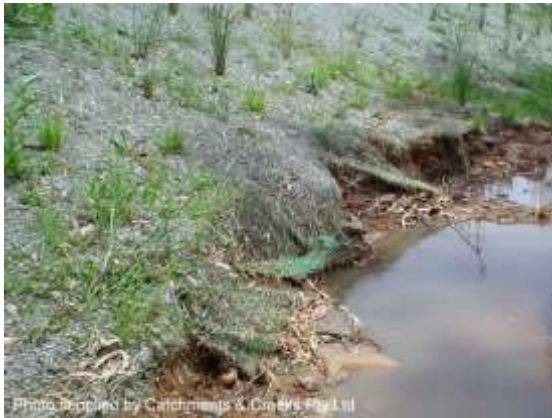
Toe erosion (Qld)
