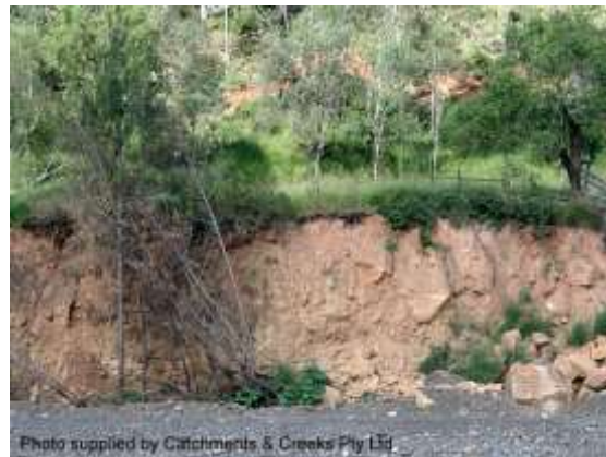
Post-flood bank erosion (Qld)
