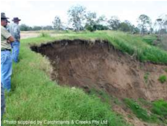
Bank slumping (Qld)
