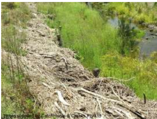
Brushwood toe protection (Qld)
