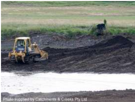
Gravel pushed up against the bank (Qld)
