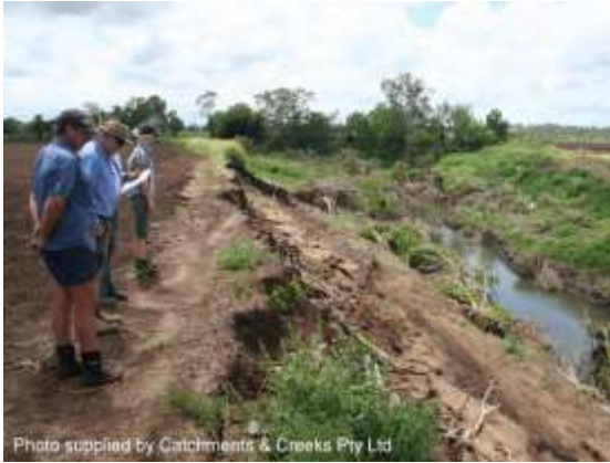
Bank scour (Qld)
