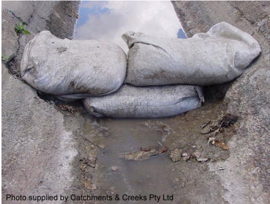
Water leakage past sandbags
