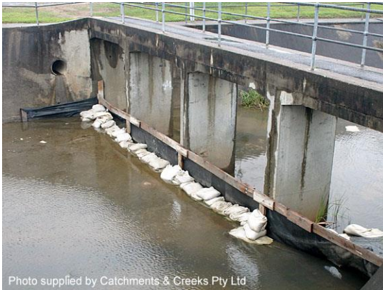
Simple filter wall (Qld)
