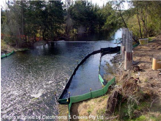
Photo supplied by Catchments & Creeks Pty Ltd Sediment fence isolation barrier (NSW)
