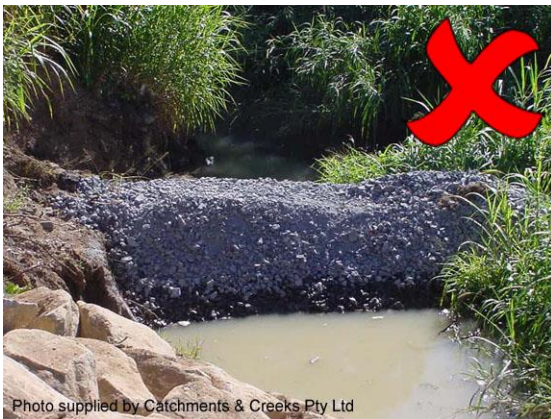
Embankment could easily wash away
