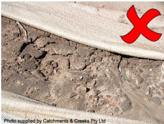
Inappropriate anchorage pegs
