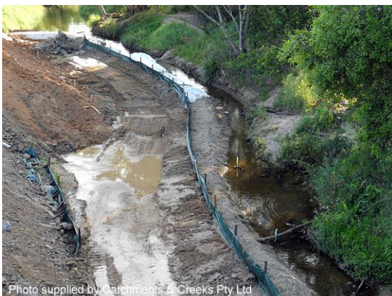
Photo supplied by Catchments & Creeks Pty Ltd Flow diversion system (Qld)
