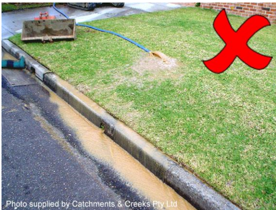
Sediment passes over saturated soil
