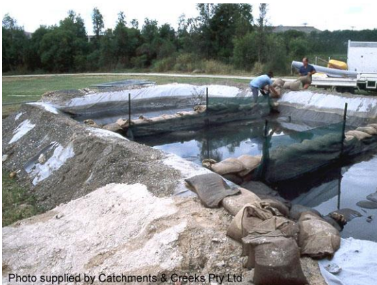
Off-stream de-watering settling pond (Qld)
