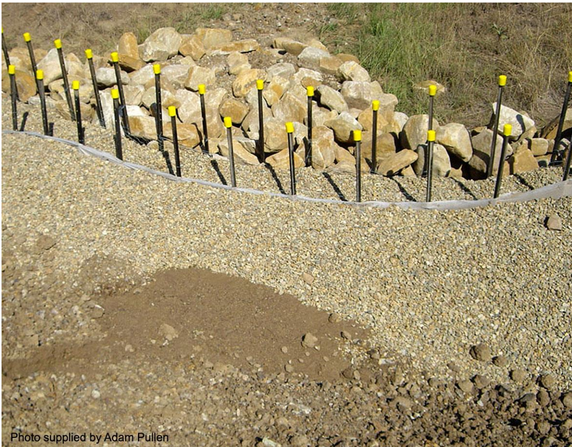
Sediment weir with aggregate filter (looking downstream)
