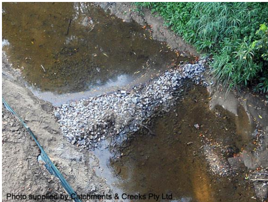
Rock filter dam
