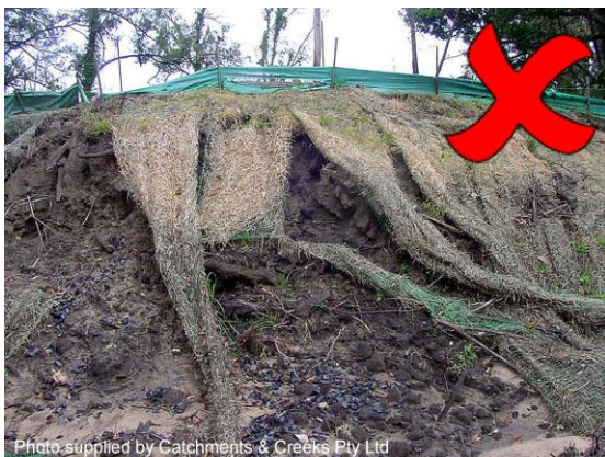
Mats overlapped in the wrong direction
