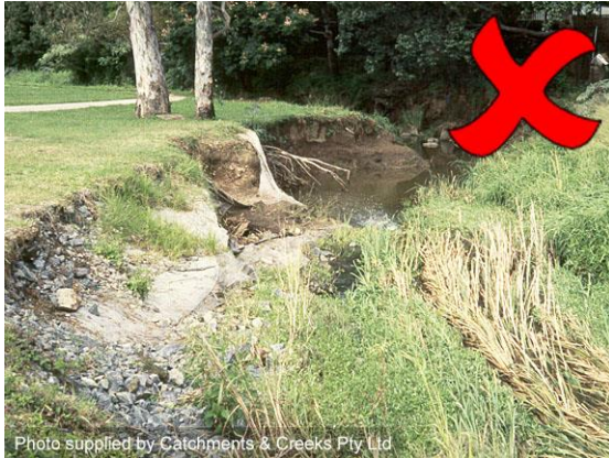
Bank erosion at d/s end of rock work
