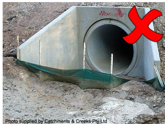
Inappropriate sediment control
