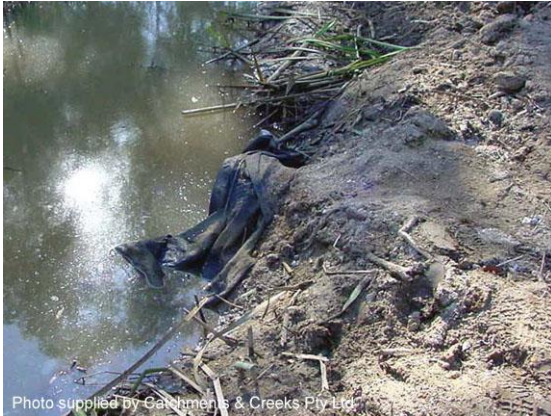
Inlet of solid pipe covered with screen
