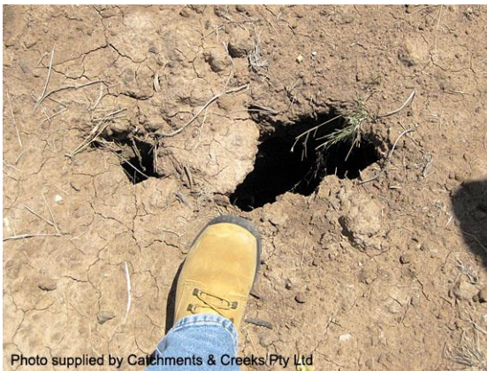
Deep rilling and tunnel erosion
