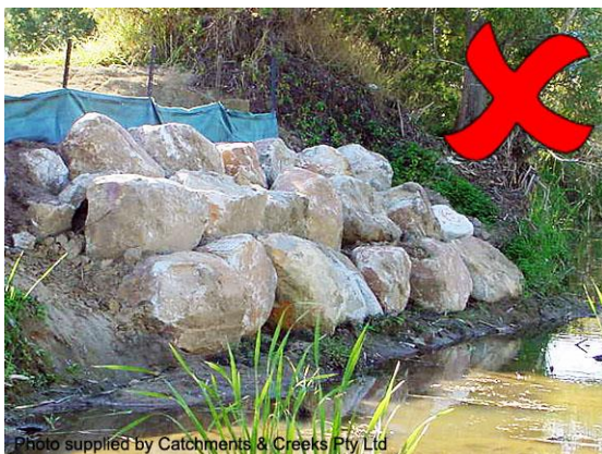
Poorly placed rocks on creek bank
