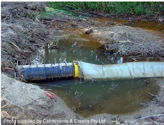
Outlet of solid pipe connected to filter tube
