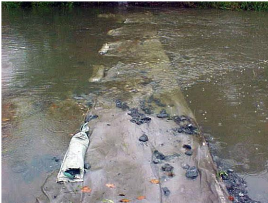
Embankment overtopped during a storm
