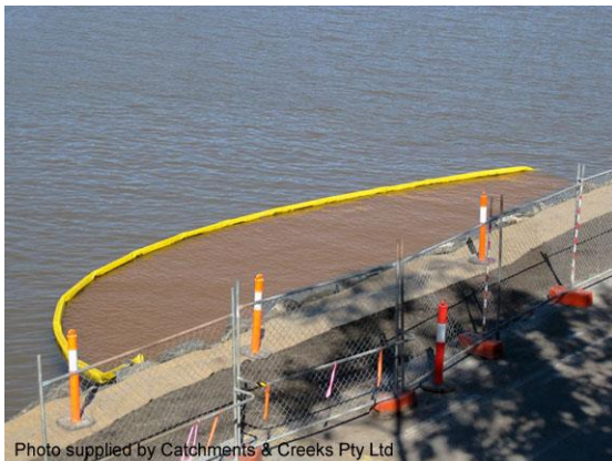
Floating silt curtain (Qld)
