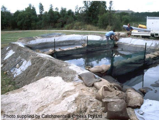
Subdivided settling pond
