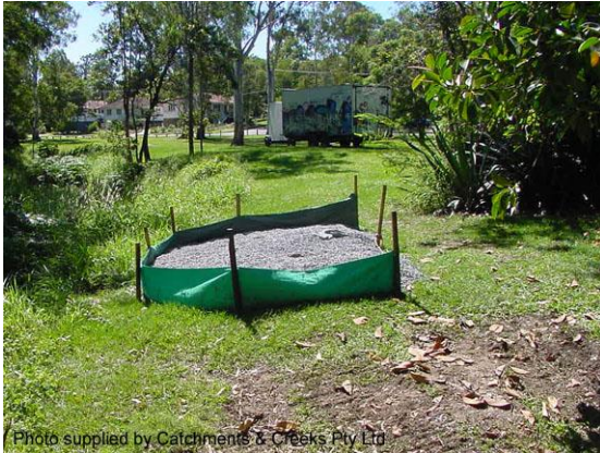
Filter fence water treatment system (Qld)
