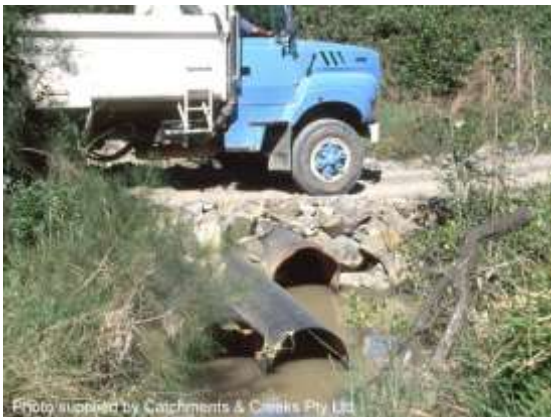
Photo supplied by Catchments & Creeks Pty Ltd Temporary pipe culvert (Qld)
