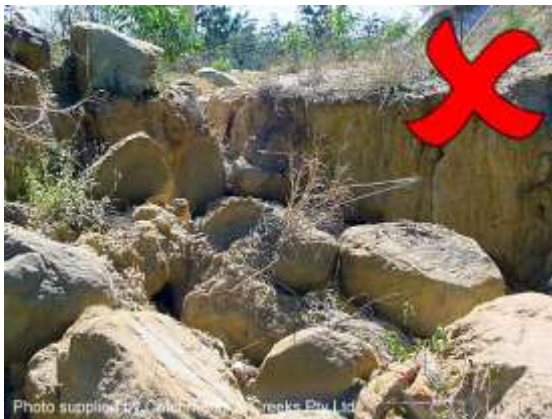
Collapsed dispersive soil bank
