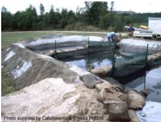
Subdivided settling pond
