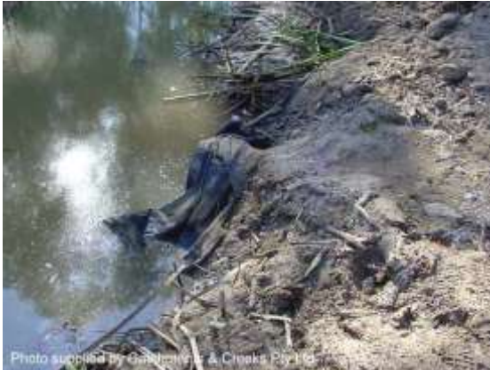
Inlet of solid pipe covered with screen
