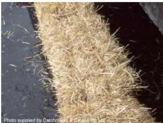
Straw bale flow diversion bank (Qld)
