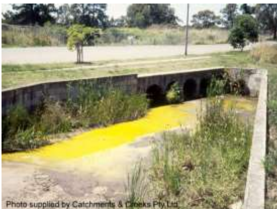
The remains of industrial runoff (Qld)
