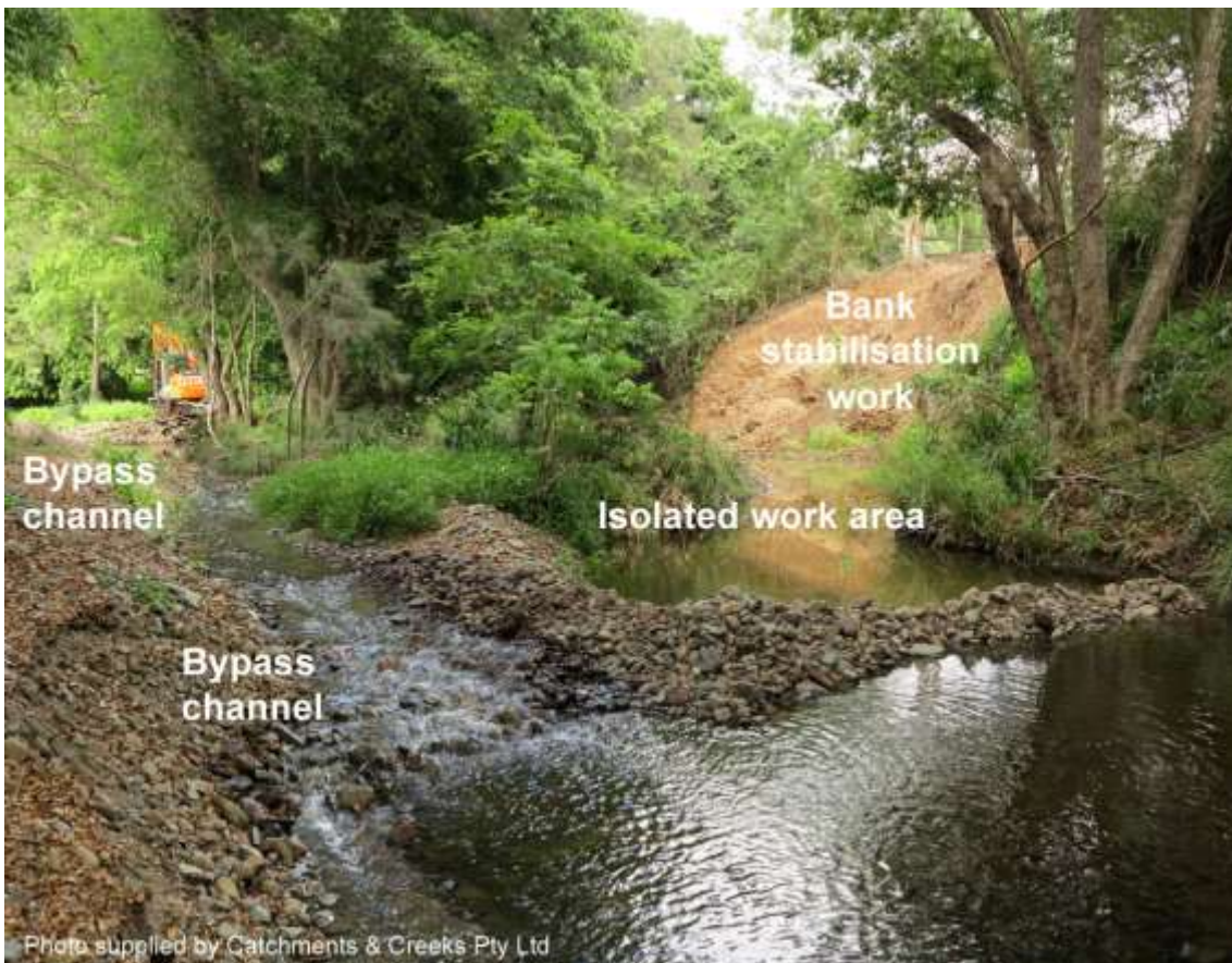
Cedar Creek with the bypass channel on the left and the work site on the right
