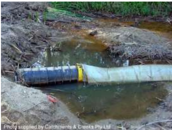
Outlet of solid pipe connected to filter tube
