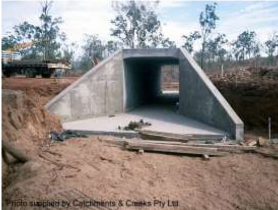
Photo supplied by Catchments & Creeks Pty Ltd Culvert construction in a dry creek bed
