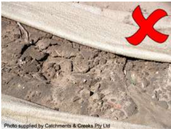
Inappropriate anchorage pegs
