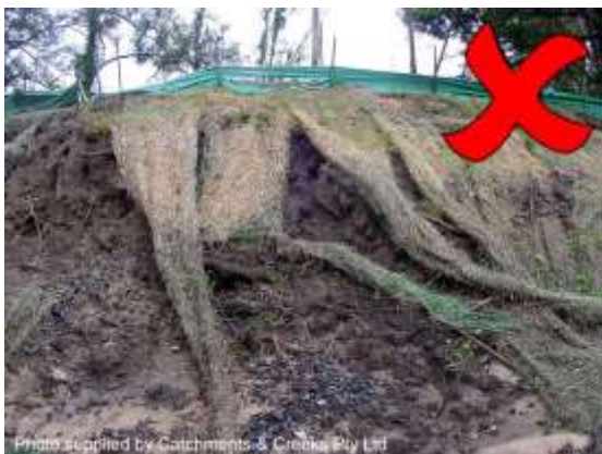
Mats overlapped in the wrong direction
