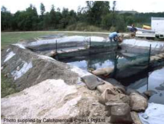
Settling pond (Qld)
