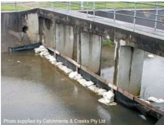
Simple filter wall (Qld)
