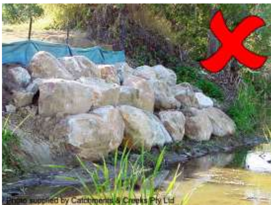
Poorly placed rocks on creek bank
