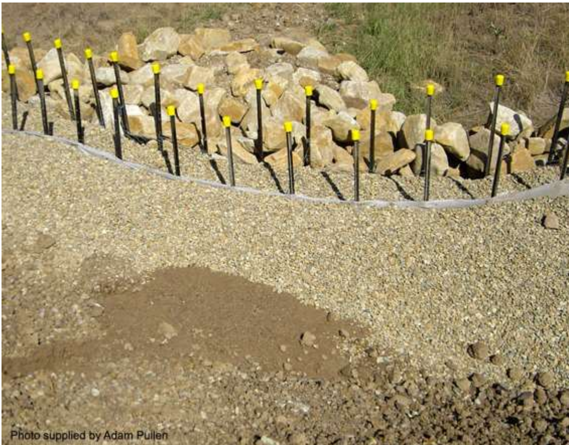
Sediment weir with aggregate filter (looking downstream)
