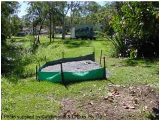
Filter fence water treatment system (Qld)
