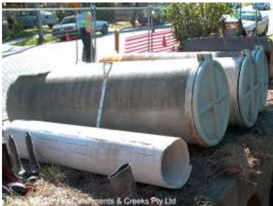
Floodgates prior to their installation
