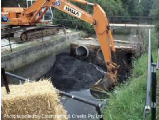
Sediment stockpiled inside the drain
