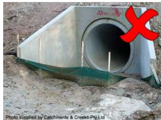
Inappropriate sediment control
