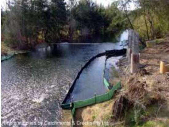
Sediment fence isolation barrier (NSW)
