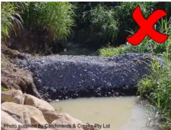
Embankment could easily wash away
