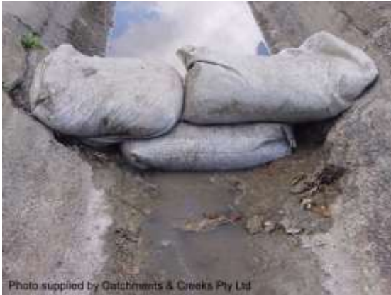
Water leakage past sandbags
