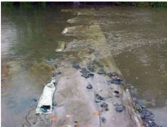
Embankment overtopped during a storm
