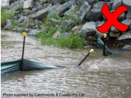
Failed sediment fence (north of NSW)
