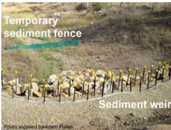
Sediment fence in an overland flow path
