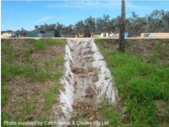
Temporary drainage chute (Qld)
