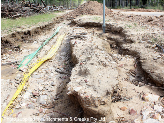
Storm damage to pipe trench
