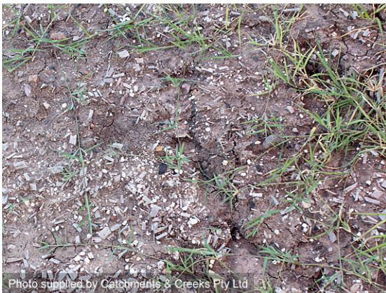
Embankment subject to sheet erosion
