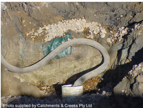
Sump pit acting as a pipe intake filter
