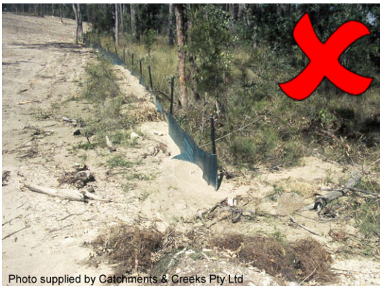
Fence not returned up-slope at end
