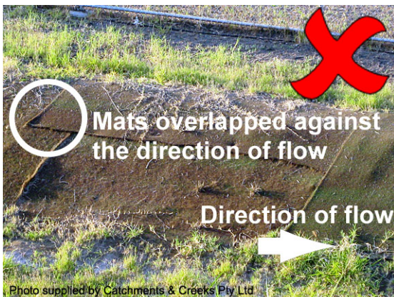
Mats overlapped in wrong direction
