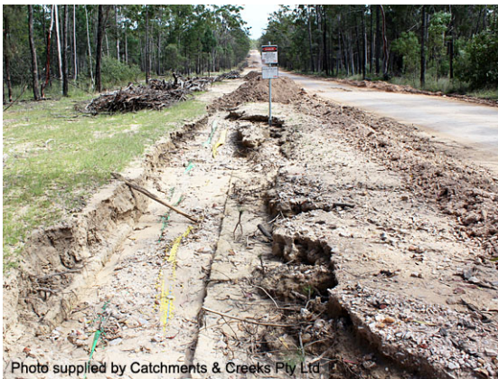
Erosion along a slaking soil trench
