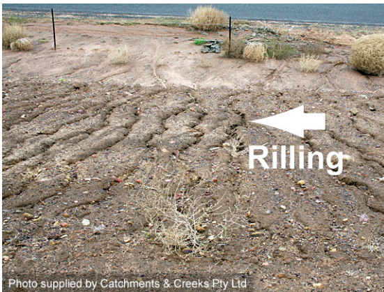
Rill erosion on an embankment
