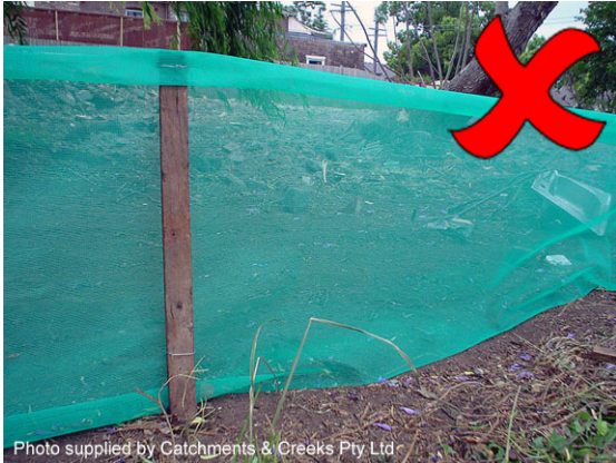
Inappropriate use of shade cloth
