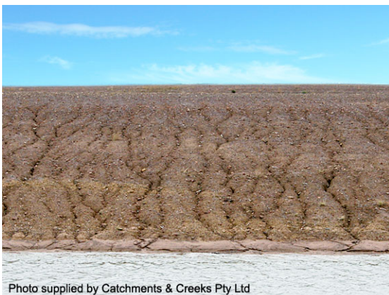
Severe rilling known as 'fluting'
