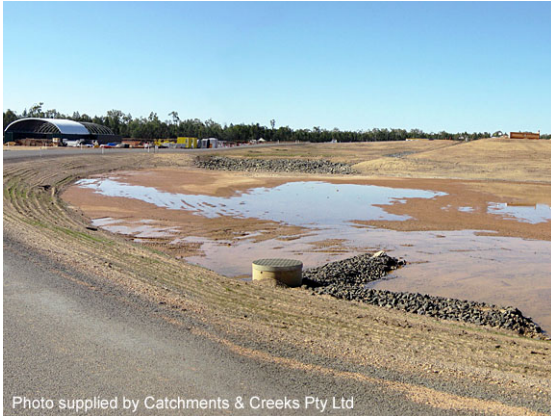
Sediment basin (Type 1)
