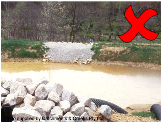
Poor sediment basin spillway design
