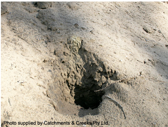
Inlet to tunnel erosion in pipe trench
