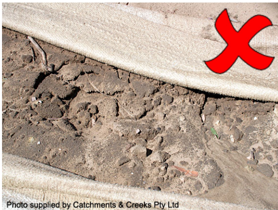
Inappropriate anchorage pegs
