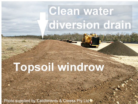
Topsoil windrow diversion drain
