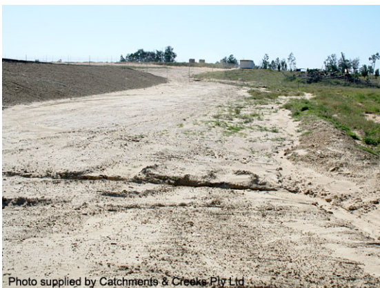
Rill erosion across an access track
