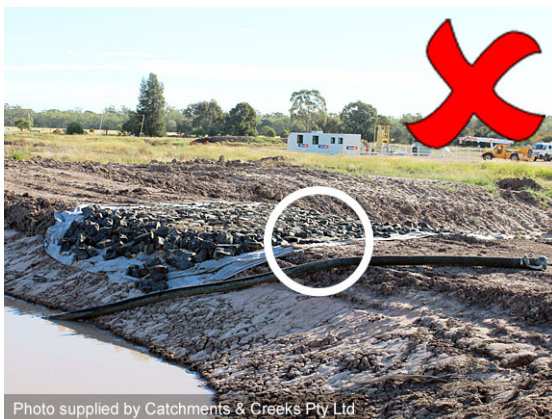
Rocks sit above the embankment height
