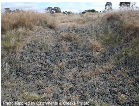
Rock mattress lined basin spillway
