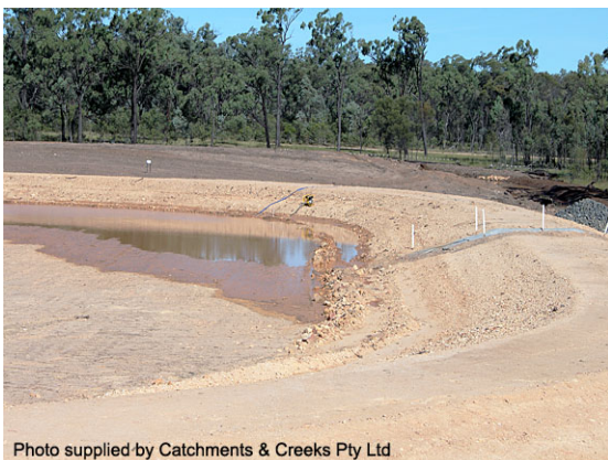
Type D sediment basin
