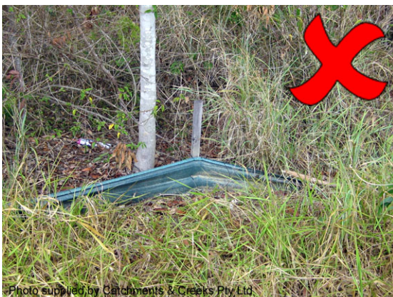
Sediment fence not removed after use
