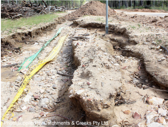
Storm damage to pipe trench
