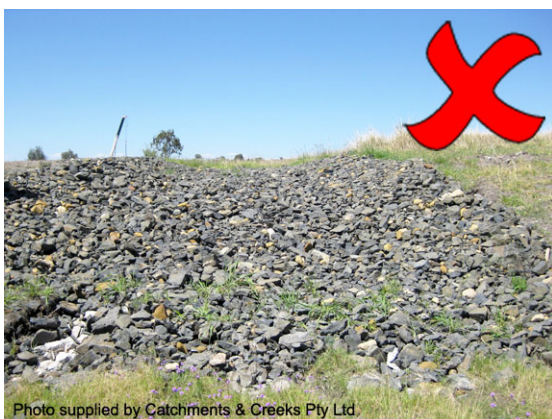
Inadequate rock size
