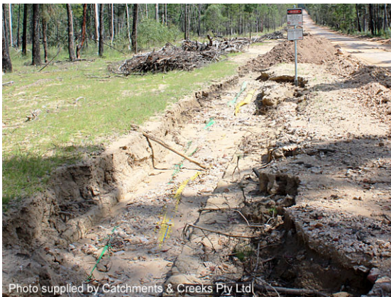
Erosion of backfilled pipe trench
