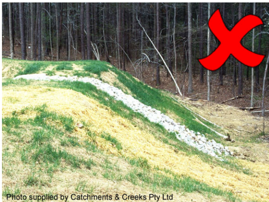
Insufficient scour protection at outlet
