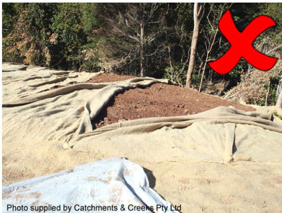
Blankets displaced by wind
