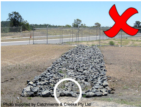
Inflow prevented from entering drain
