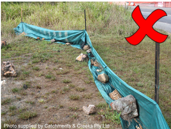
Toe of fabric incorrectly anchored
