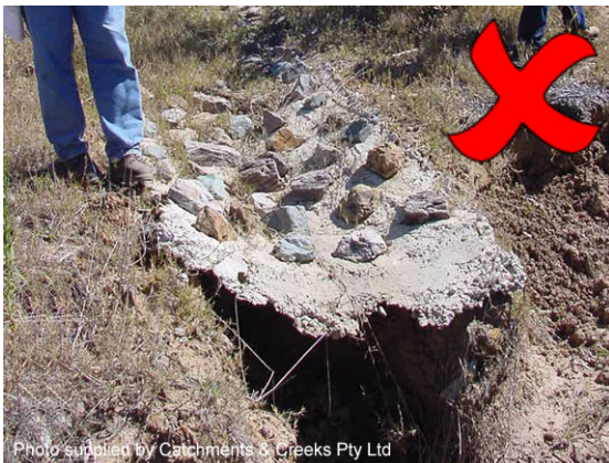
Tunnel erosion under concrete
