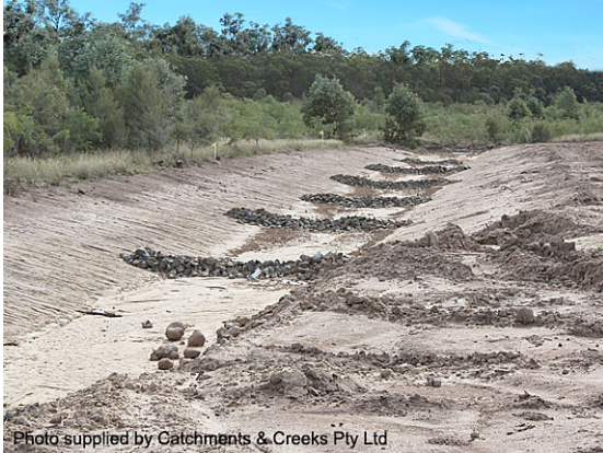
Check dam sediment trap
