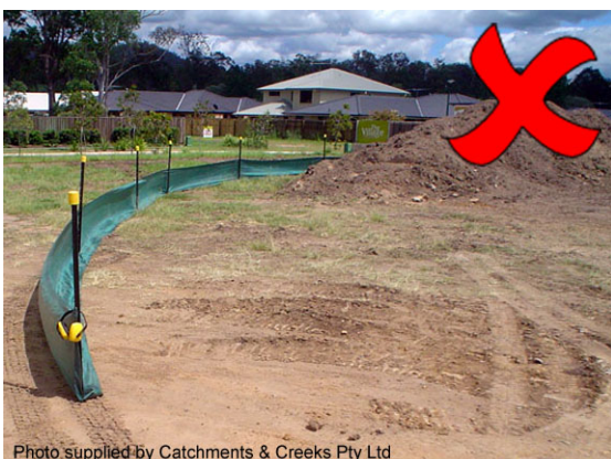
Post placed on wrong side of fence
