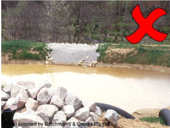
Poorly defined spillway crest
