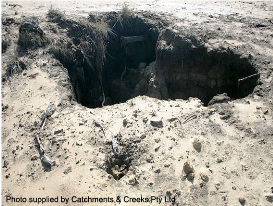
Entrance to tunnel erosion
