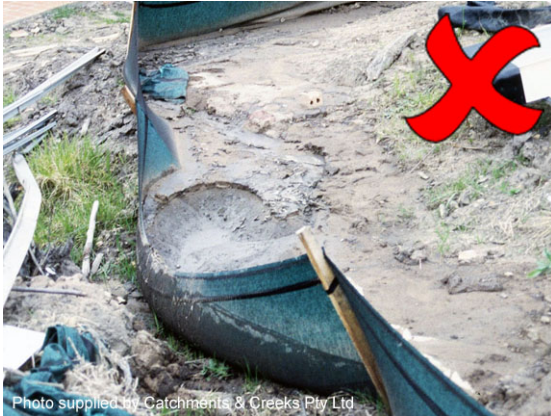
Sediment fence in need of maintenance
