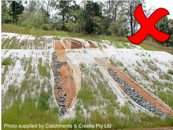
Blankets displaced by winds
