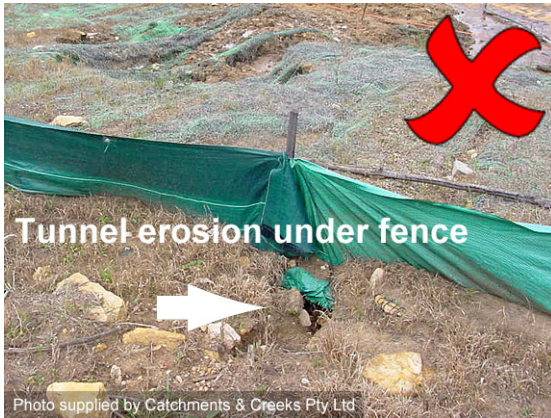
Storm damage to sediment fence
