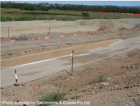
Drained wash bay
