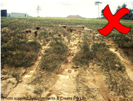
Erosion of recently seeded surface
