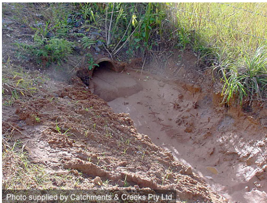
Deposition of sediment in a storm drain
