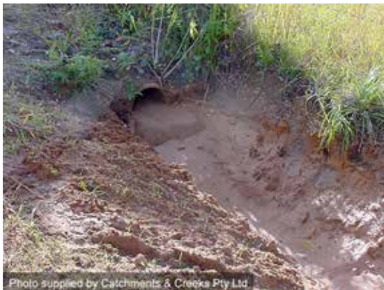
Deposition of sediment in a storm drain
