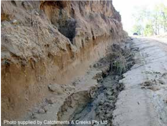
Deep rilling within a sandy soil
