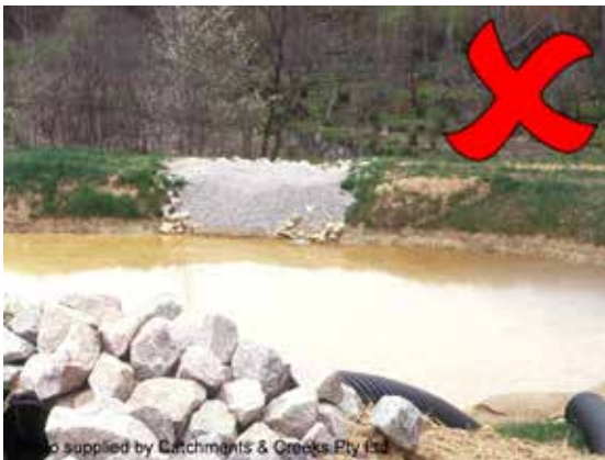
Poor sediment basin spillway design
