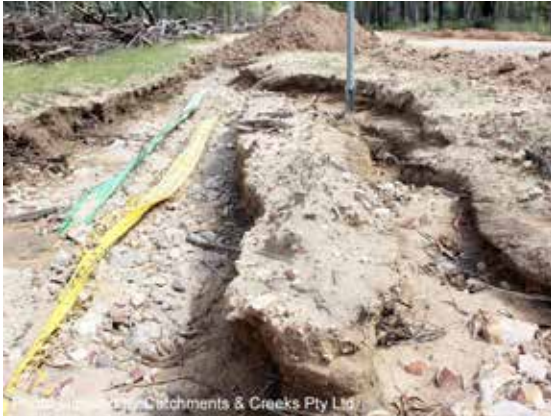
Storm damage to pipe trench
