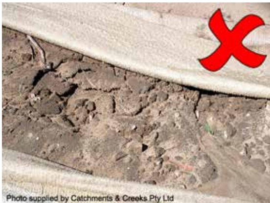
Inappropriate anchorage pegs
