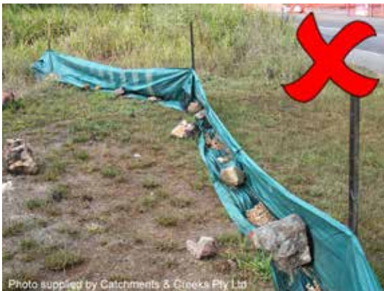
Toe of fabric incorrectly anchored
