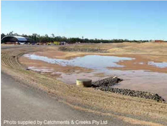
Sediment basin (Type 1)
