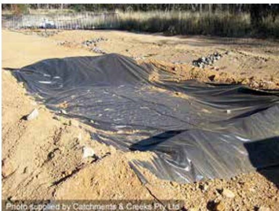
Concrete truck wash-out point
