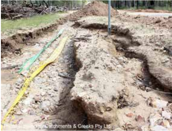
Storm damage to pipe trench
