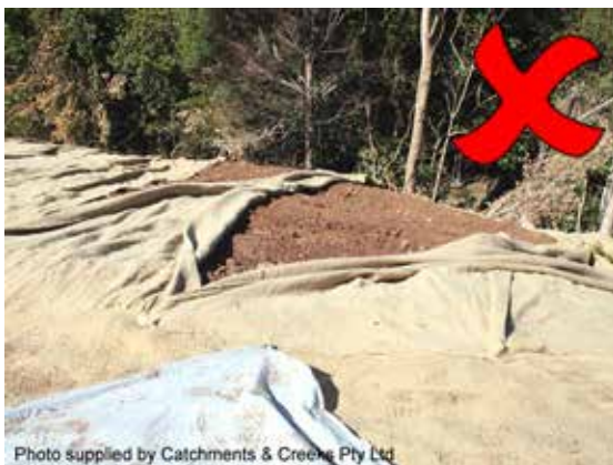
Blankets displaced by wind
