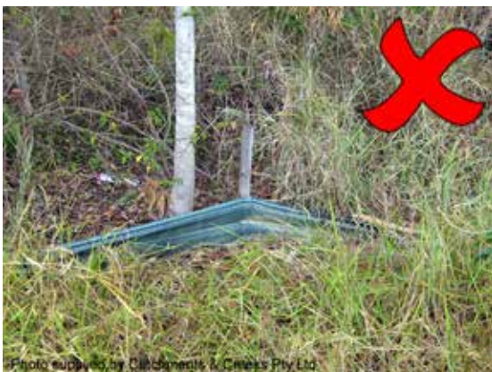
Sediment fence not removed after use
