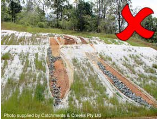
Blankets displaced by winds
