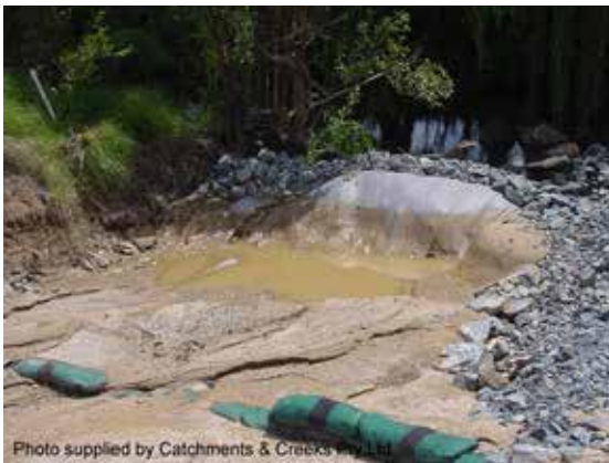
Rock filter dam (Type 2)
