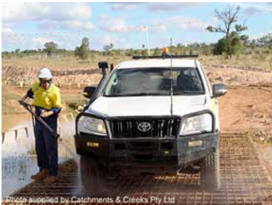
Vehicle wash-down area
