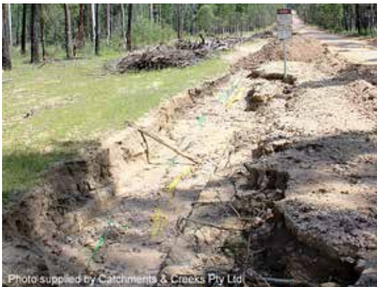
Erosion of backfilled pipe trench
