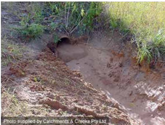
Sedimentation of drainage pipe
