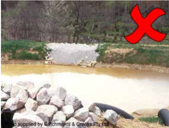
Poorly defined spillway crest
