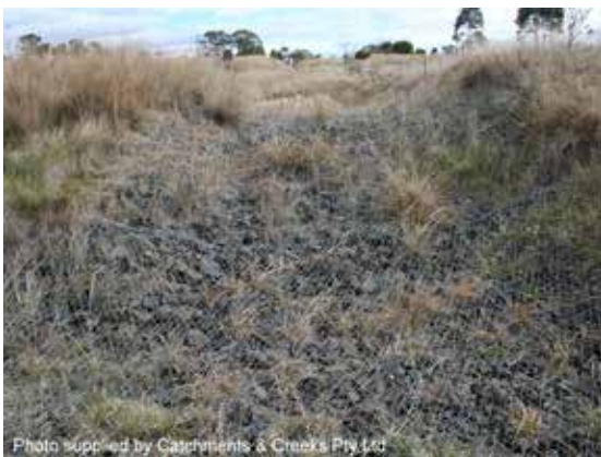
Rock mattress lined basin spillway
