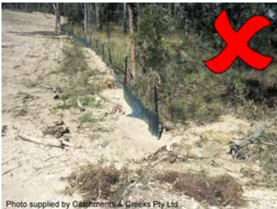
Fence not returned up-slope at end
