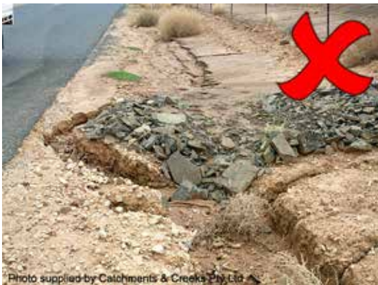
Failure of a check dam on a dispersive soil
