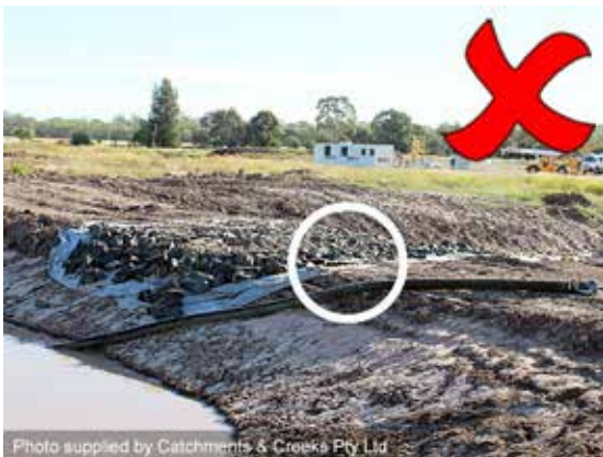
Rocks sit above the embankment height
