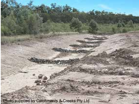
Check dam sediment trap
