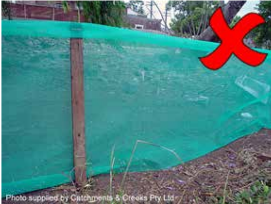
Inappropriate use of shade cloth
