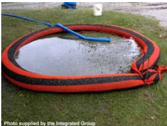
Compost-filled filter sock
