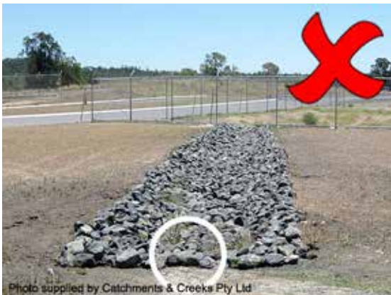
Inflow prevented from entering drain
