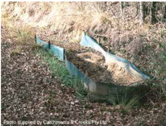
U-shaped sediment trap in steep drain
