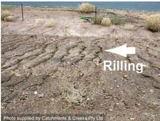
Rill erosion on an embankment
