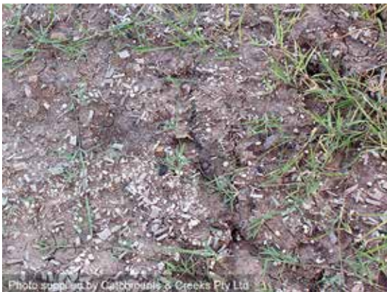
Embankment subject to sheet erosion
