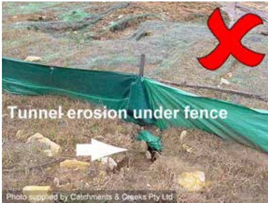
Storm damage to sediment fence
