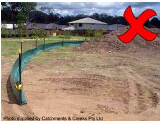
Post placed on wrong side of fence
