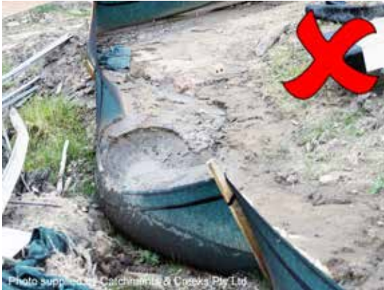
Sediment fence in need of maintenance
