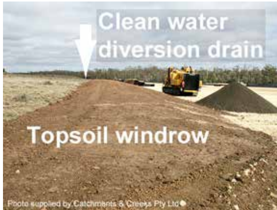
Topsoil windrow diversion drain
