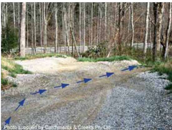
Cross bank drainage
