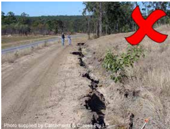
Catch drain cut into a dispersive soil
