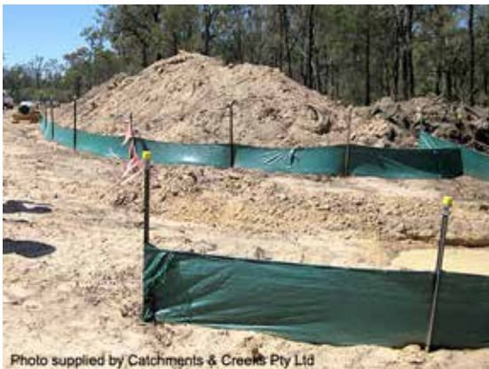
Sediment trap on pipeline RoW
