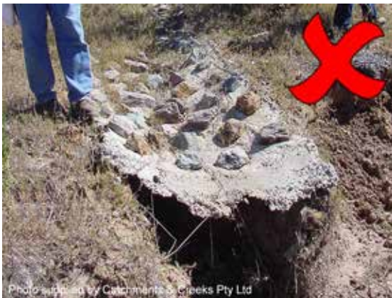
Tunnel erosion under concrete
