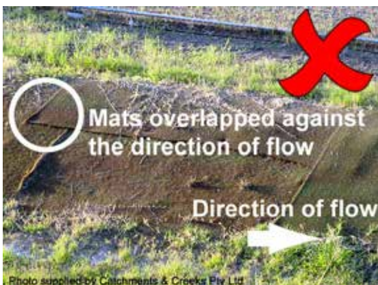
Mats overlapped in wrong direction
