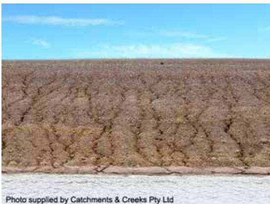
Severe rilling known as 'fluting'
