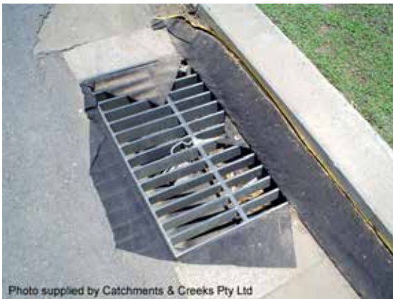
Gully bag sediment trap
