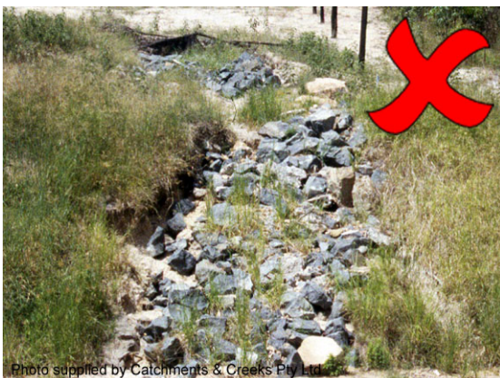
Rock placed on a dispersive soil bank
