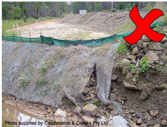
Bank erosion adjacent pipe alignment
