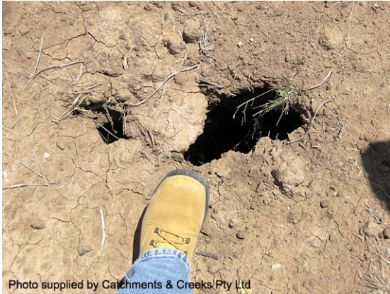
Tunnel erosion above pipeline
