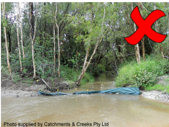
Inappropriate instream sediment control
