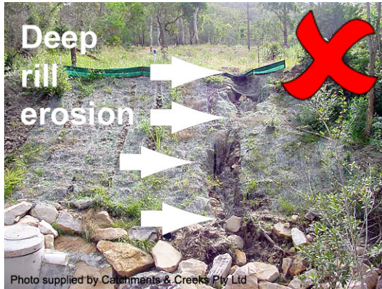
Failure of bank stabilisation works
