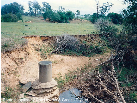
Bank erosion exposes sewer pipe
