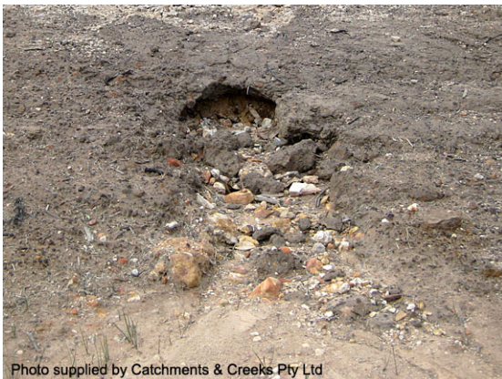
Outlet of above tunnel erosion
