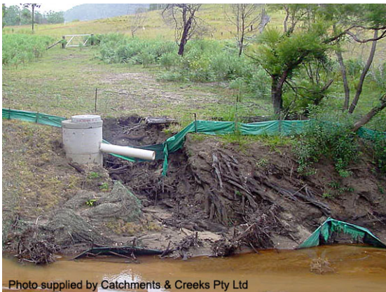
Bank erosion adjacent access pit
