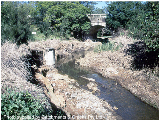
Bank erosion downstream of chamber
