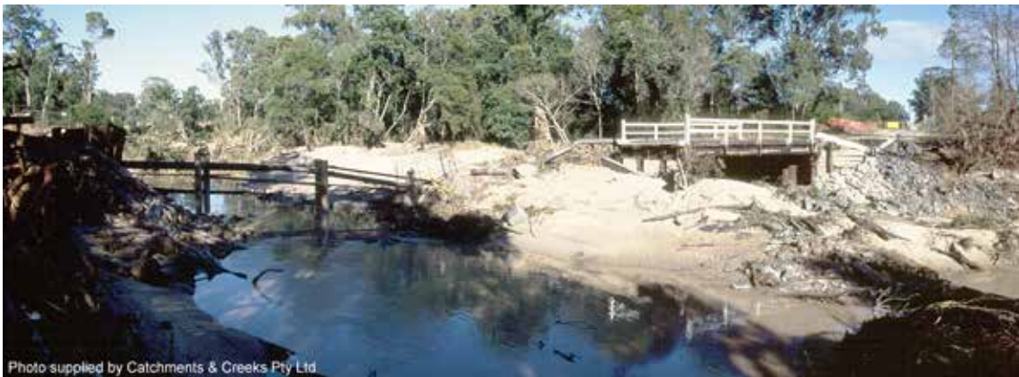
Flood damaged Brookbent Rd bridge abutment and attached pipe work
