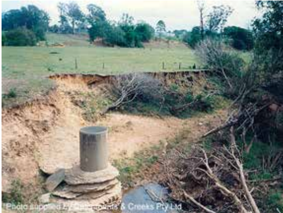
Bank erosion exposes sewer pipe
