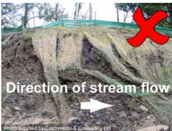
Failed erosion control mat
