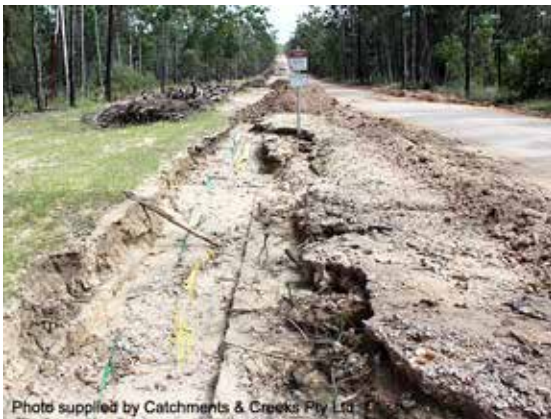
Erosion along the pipeline RoW
