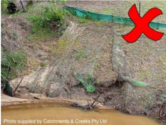
Erosion along toe of bank
