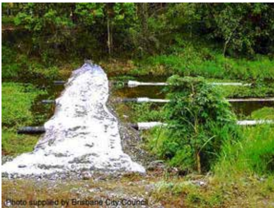
Rock filter dam with filter tubes
