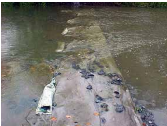
Elevated stream flows at work site
