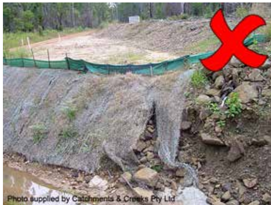
Bank erosion adjacent pipe alignment
