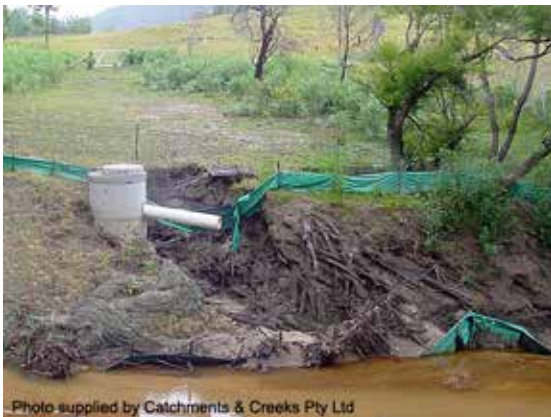
Bank erosion adjacent access pit
