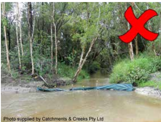
Inappropriate instream sediment control
