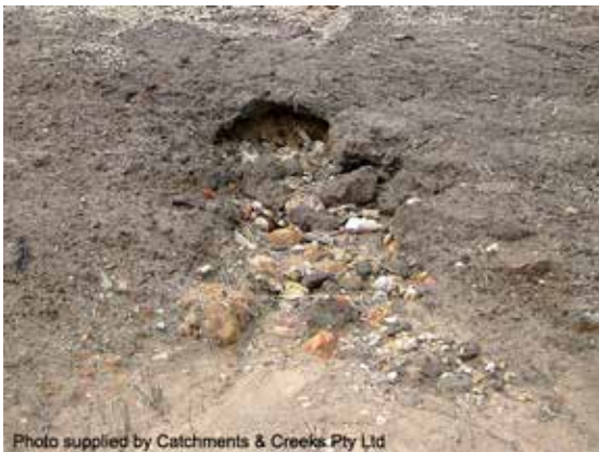
Outlet of above tunnel erosion
