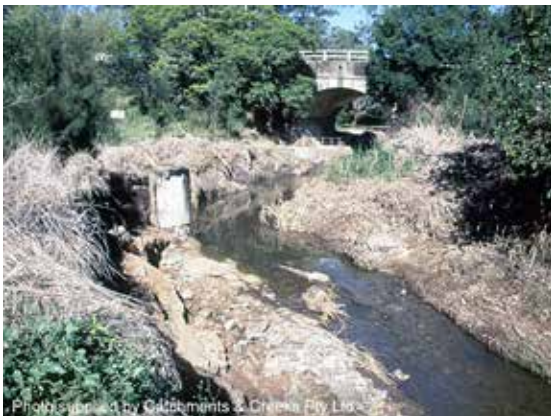
Bank erosion downstream of chamber
