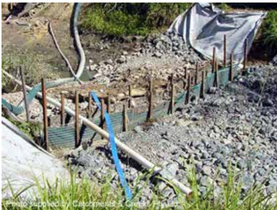
Instream sediment weir
