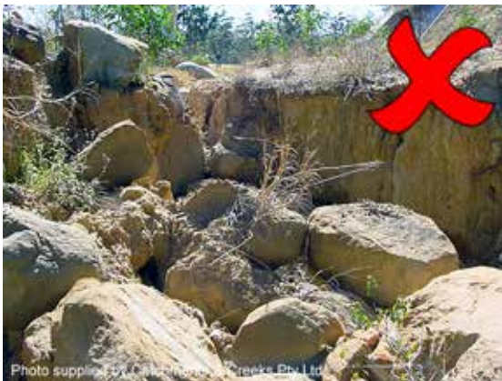
Collapsed dispersive soil bank
