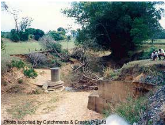
Pipeline exposed by migrating waterway
