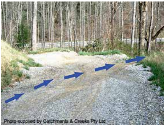
Flows diverted off access track
