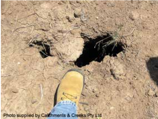
Tunnel erosion above pipeline
