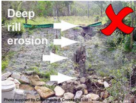
Failure of bank stabilisation works
