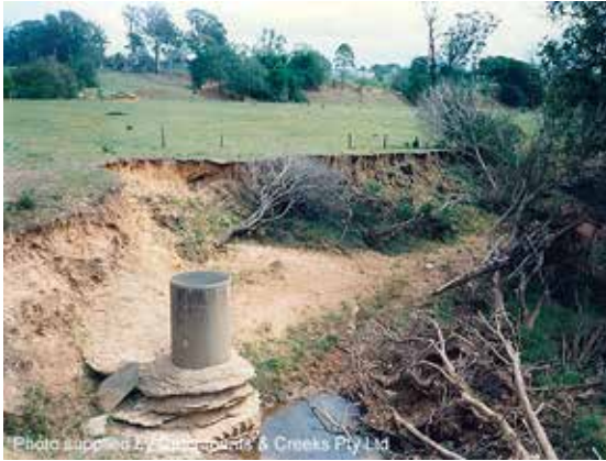
Bank erosion exposes sewer pipe
