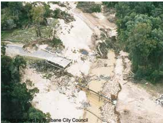
Flood damage to bridge & buried pipes
