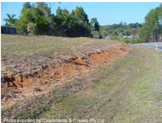
Loss of vegetation from the road batter
