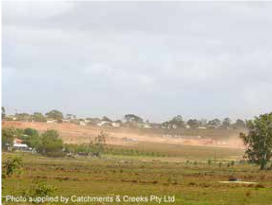
Construction site dust
