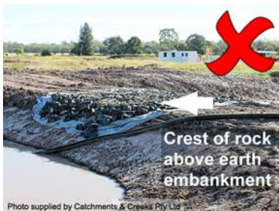
Inappropriate spillway crest profile
