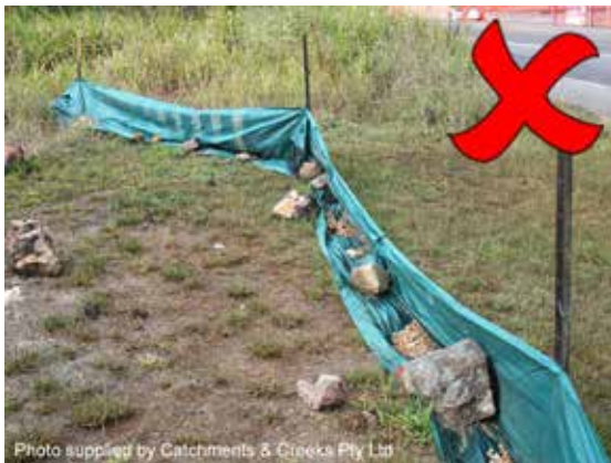
Toe of fabric incorrectly anchored
