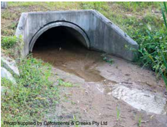
Sedimentation of drainage pipe
