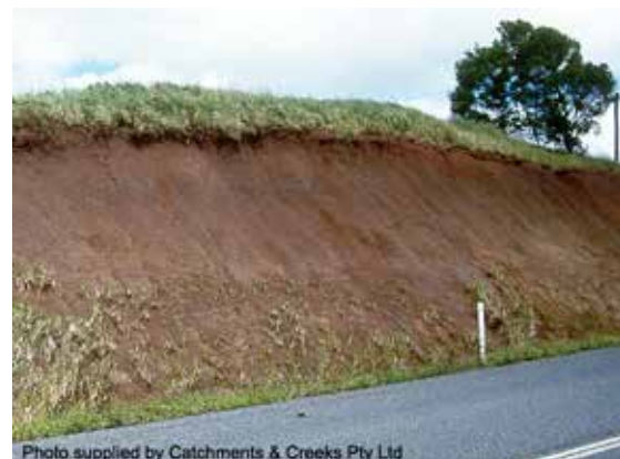
Eroded road batter
