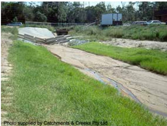
Deposition of sediment in a storm drain
