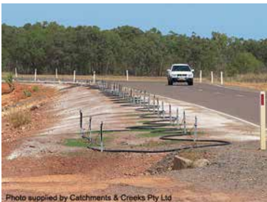
Temporary irrigation system
