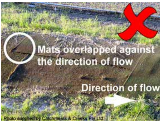
Mats overlapped in wrong direction
