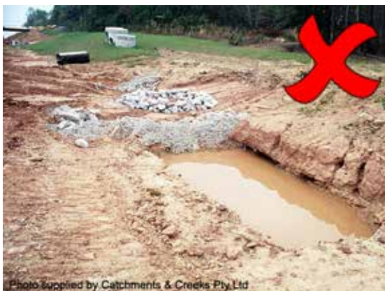
Sediment sump formed in dispersive soil
