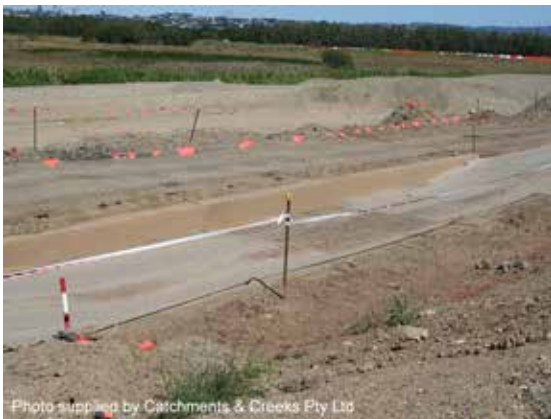
Drained wash bay (vibration grid)
