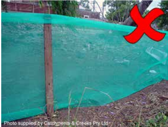
Inappropriate use of shade cloth
