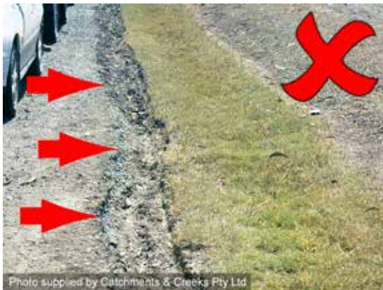
Rilling along the edge of turf
