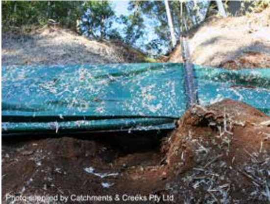
Storm undermines a sediment fence
