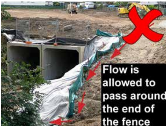
Sediment fence fails to capture sediment
