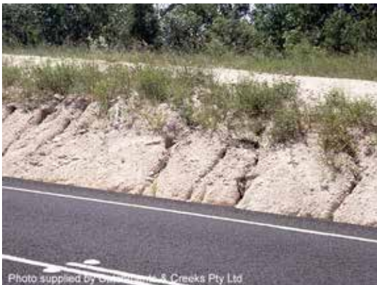
Rill erosion on a cut batter
