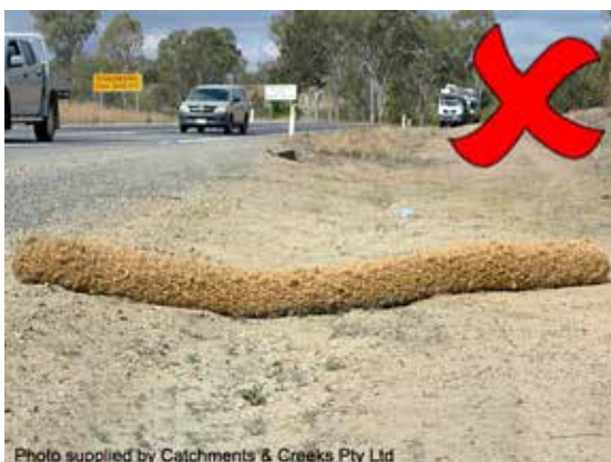
Geo log not adequately staked
