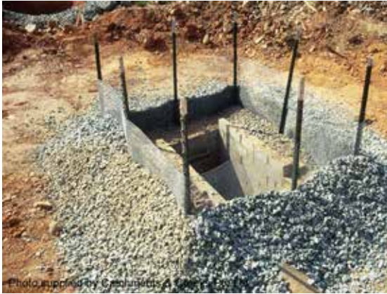
Mesh & aggregate drop inlet protection
