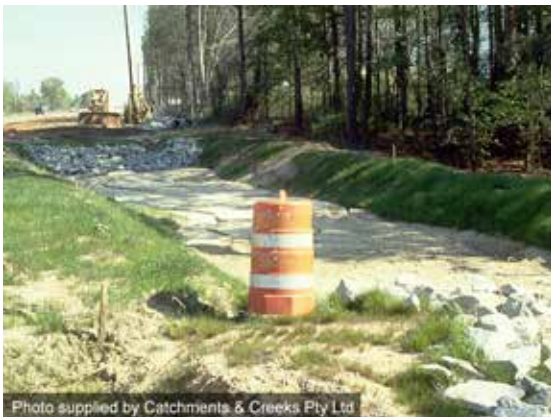
Rock filter dam
