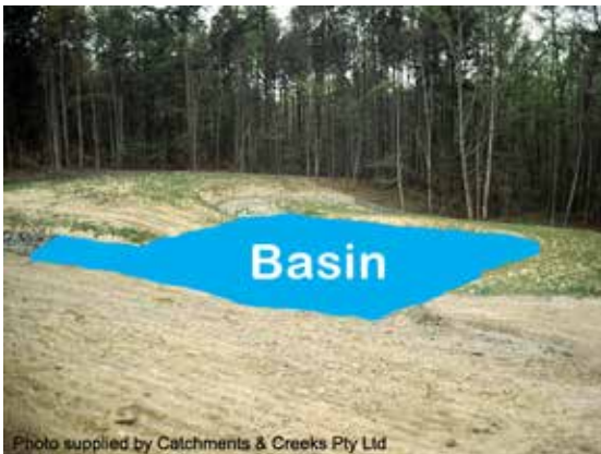
Roadside sediment basin
