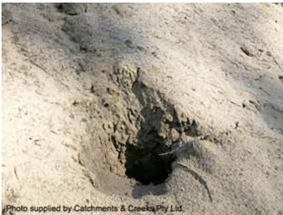
Inlet to tunnel erosion in pipe trench
