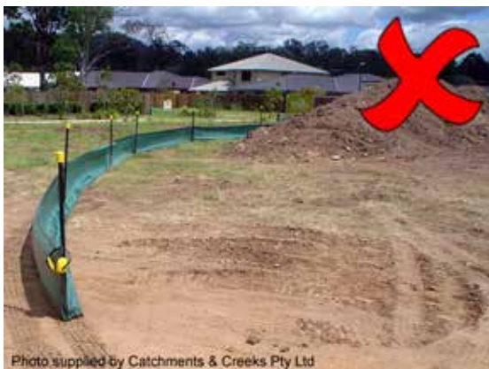
Post placed on wrong side of fence
