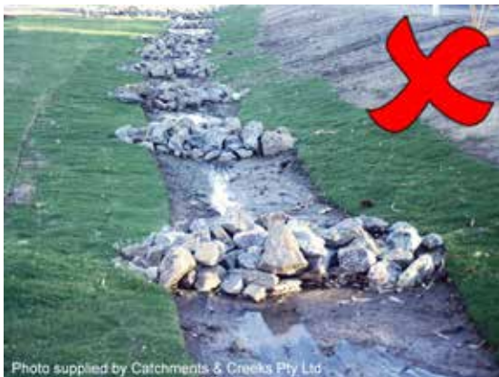
Flows forced to pass around check dams
