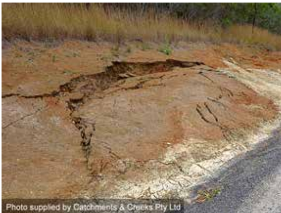
Bank slumping on a cut batter
