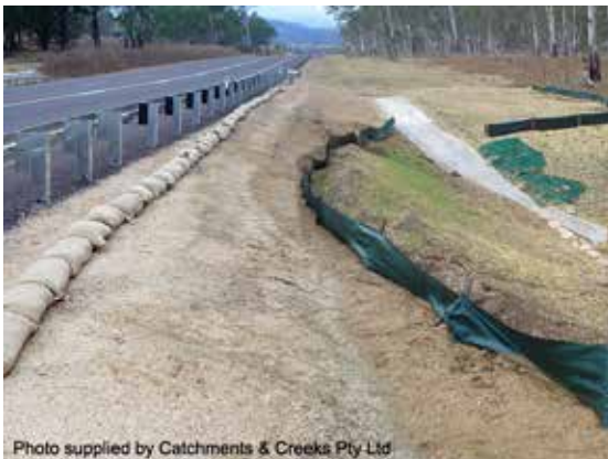
Sandbags used to divert road runoff
