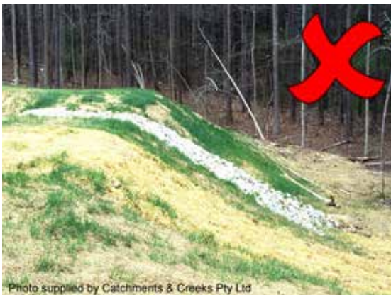
Insufficient scour protection at outlet
