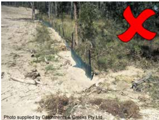
Fence not returned up-slope at end
