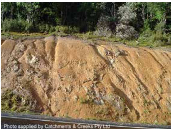
Rilling that extends to top of bank
