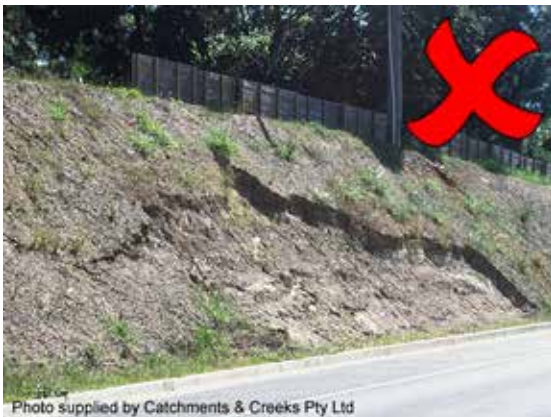
Slippage of topsoil from steep batter
