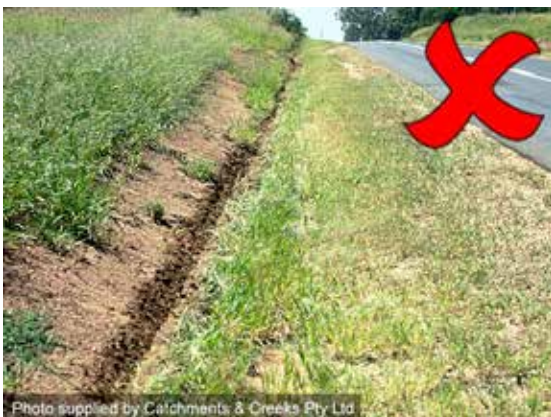
Scour damage to batter toe
