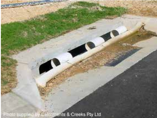
Sag inlet sediment trap
