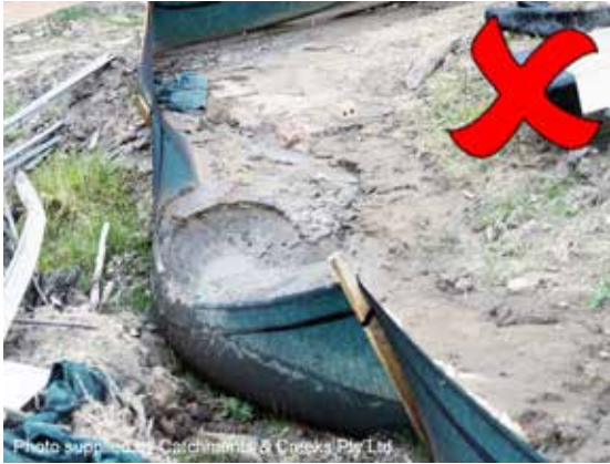
Sediment fence in need of maintenance
