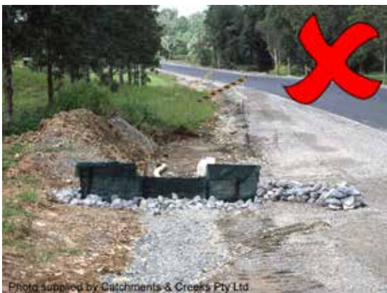
Common sense gone missing!
