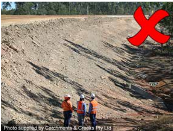
Batter without appropriate erosion control
