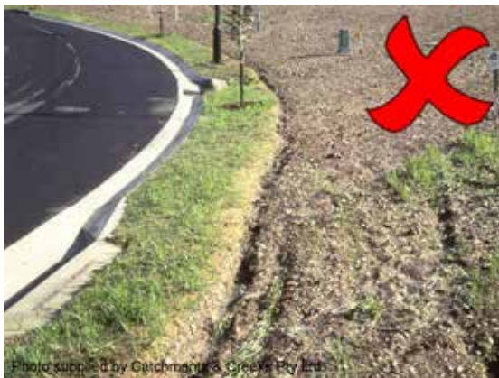
Rilling along the edge of turf
