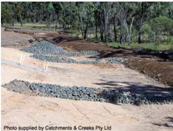
Velocity control check dams
