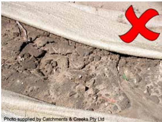
Inappropriate anchorage pegs
