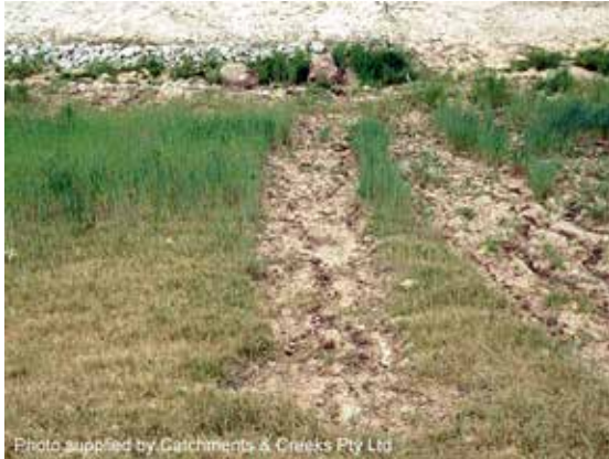
Rilling on a newly seeded batter
