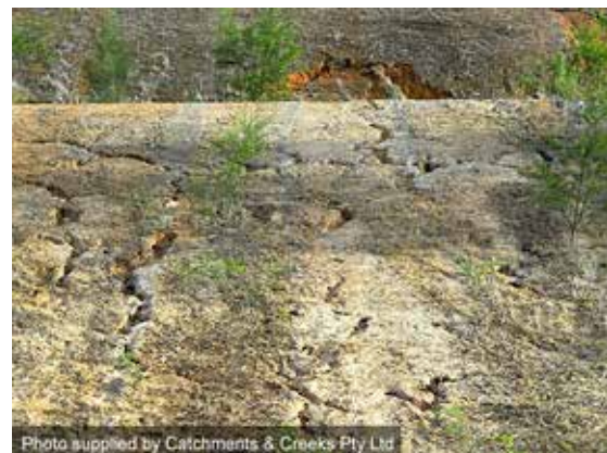
Evidence of ongoing rill erosion (2013)
