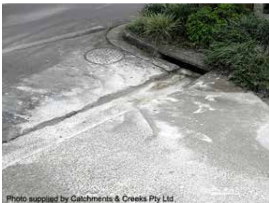
Deposition of cement wash-off on a road
