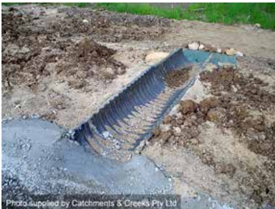
Temporary half-pipe batter chute
