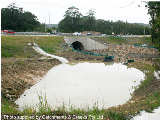
Stormwater treatment pond (2009)
