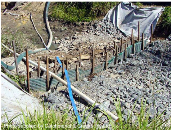
Instream sediment weir
