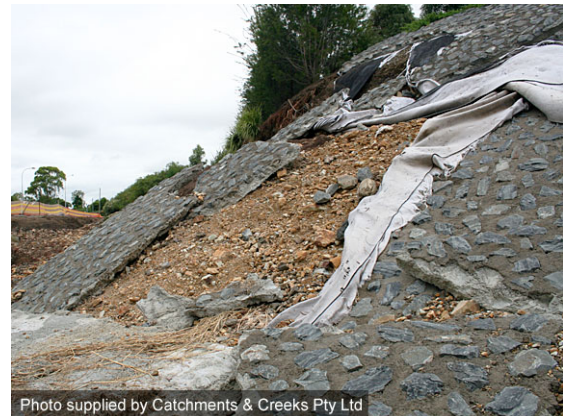
Failed stone pitching (same bridge)
