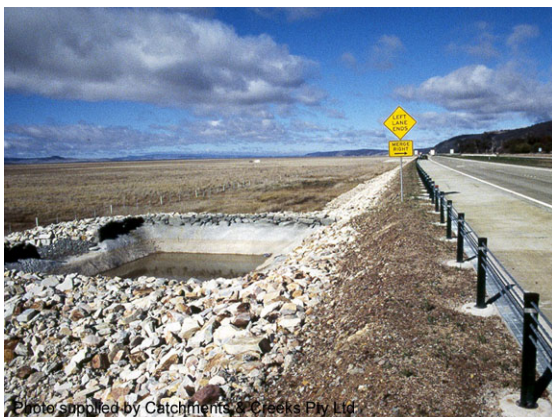
Roadside pollution containment pond
