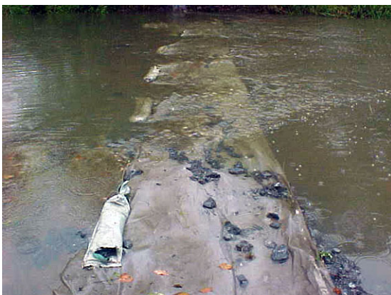
Elevated stream flows at work site
