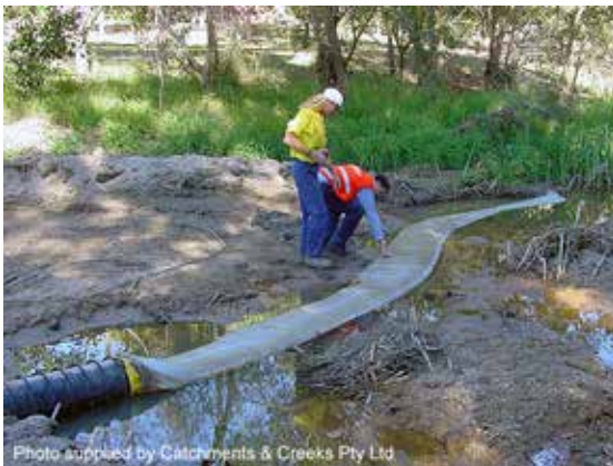
Instream sediment control system
