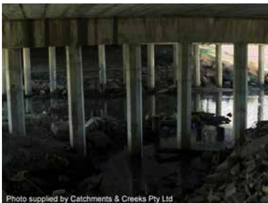
Poor light conditions under a bridge
