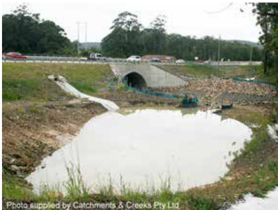
Stormwater treatment pond (2009)
