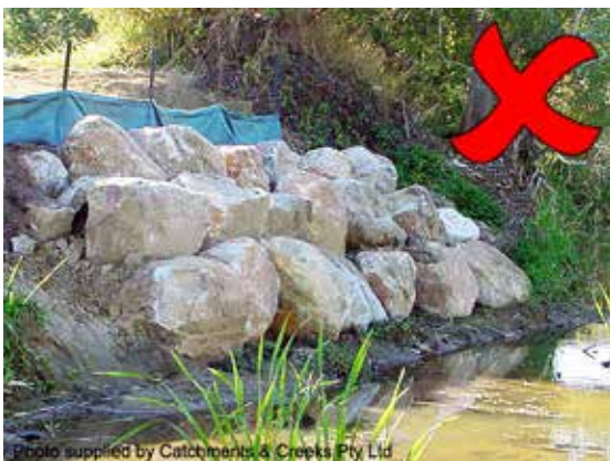
Poorly placed rocks on creek bank
