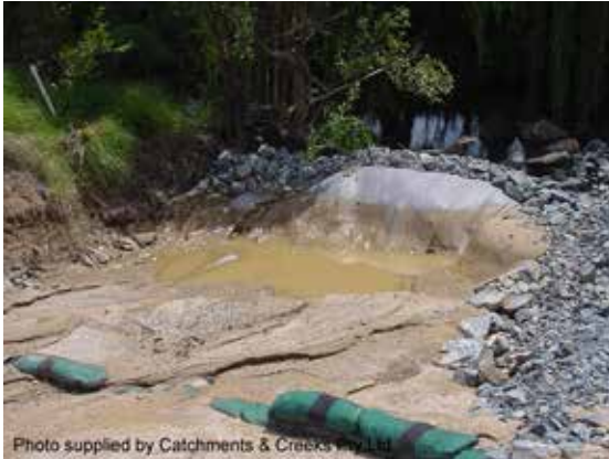
Rock filter dam (Type 2 sediment trap)
