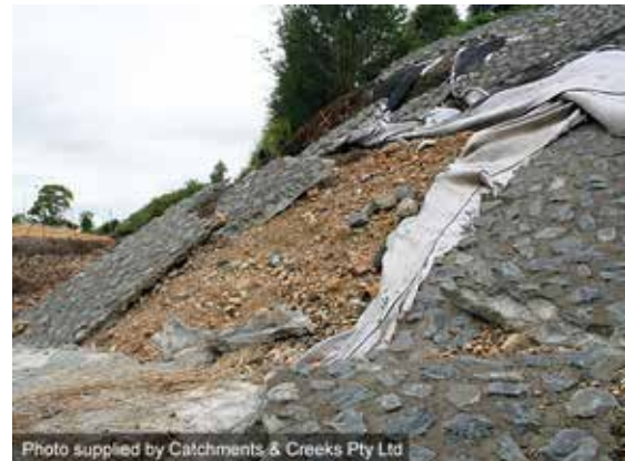
Failed stone pitching (same bridge)
