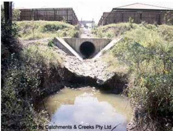
Urban stormwater pipe drainage line
