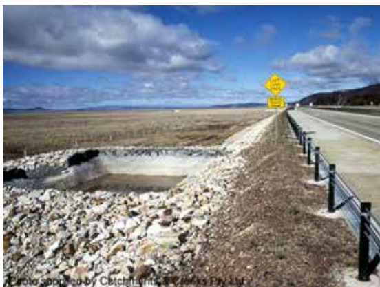
Roadside pollution containment pond
