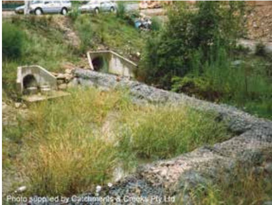
Roadside bio-retention system
