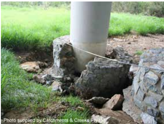
Flood damage to bridge pier
