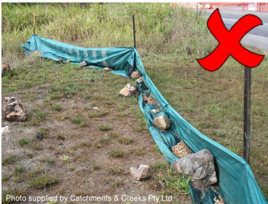
Toe of fabric incorrectly anchored
