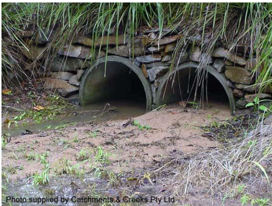
Sedimentation of drainage pipes
