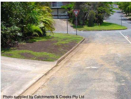
Soil swept from roadway
