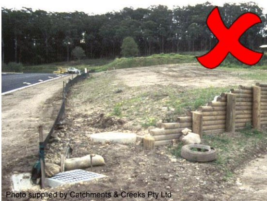
Fence not returned up-slope at end
