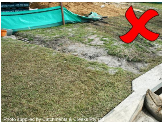
Poorly backfilled service trench
