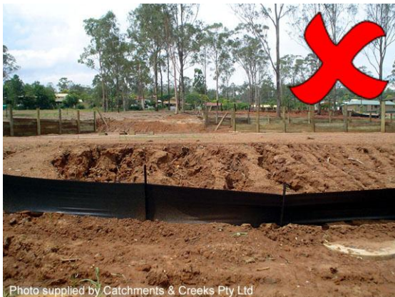
Severe rill erosion
