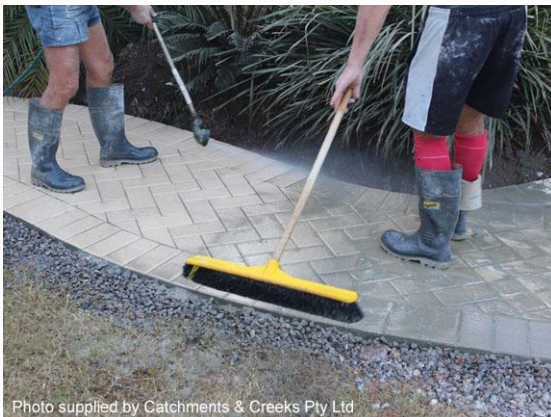
Cement washed onto porous soil
