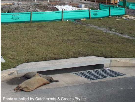
Retention of down-slope grass filter
