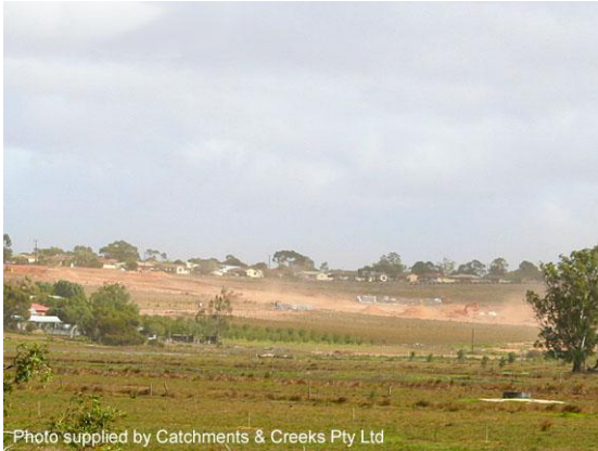
Dust generated on a construction site
