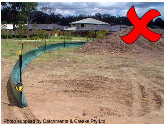
Post placed on wrong side of fence
