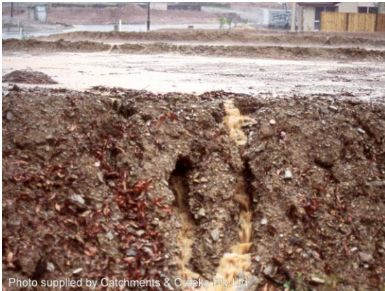
Rill erosion adjacent a building pad
