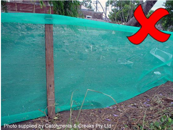
Inappropriate use of shade cloth
