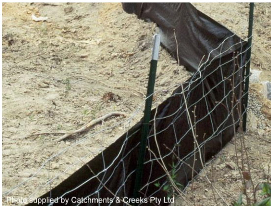
Wire mesh backing
