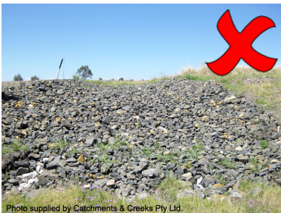
Inadequate rock size
