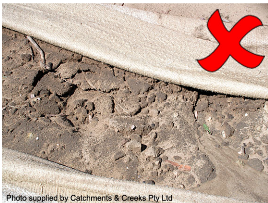
Inappropriate anchorage pegs
