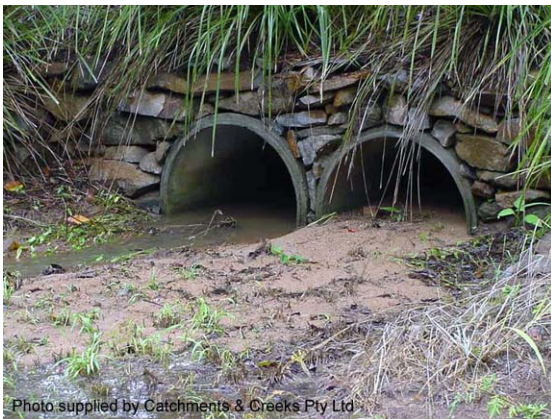
Sedimentation of a drainage pipe
