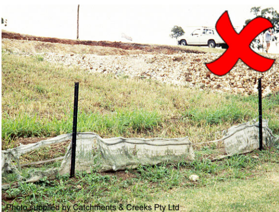
Sediment fence well past its 'use-by' date
