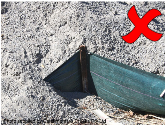
Sediment fence in need of maintenance
