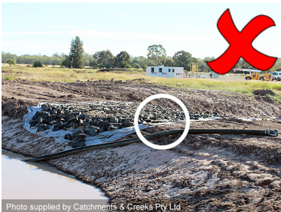
Rocks sit above the embankment height
