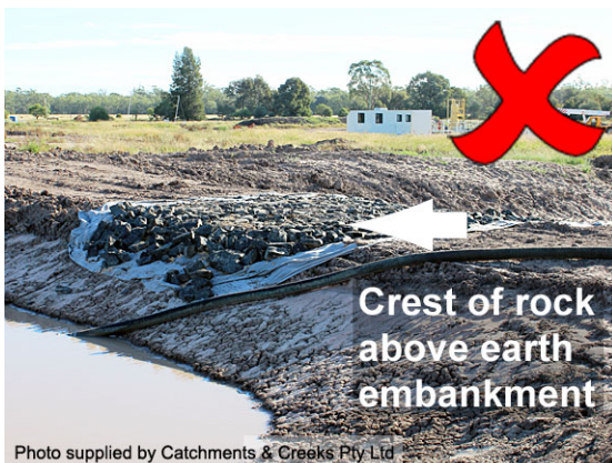
Inappropriate spillway crest profile
