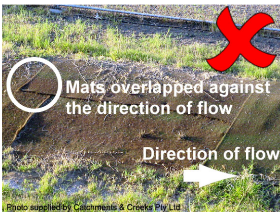
Mats overlapped in wrong direction
