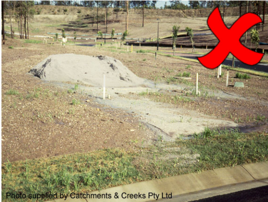
Inappropriately located sand stockpile
