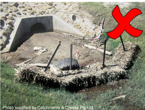
Inappropriate choice of sediment trap
