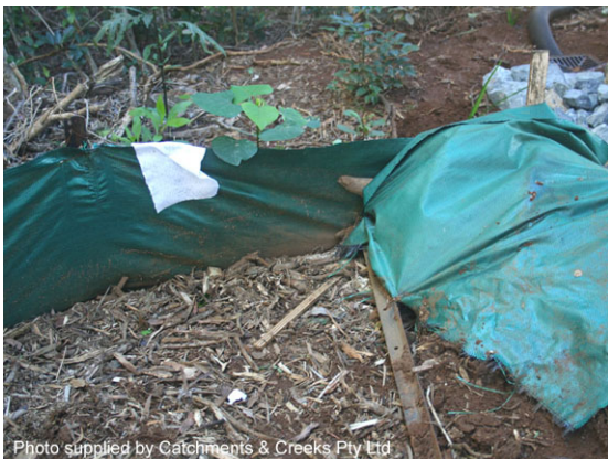
Damaged fence tagged (white) for repair
