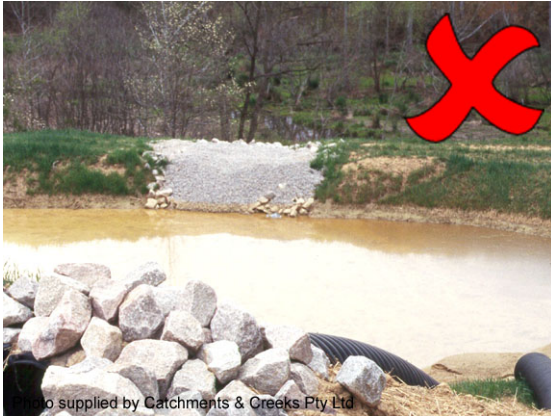
Poorly defined spillway crest
