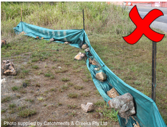
Toe of fabric incorrectly anchored
