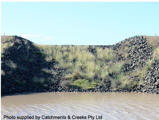
Energy dissipation pond
