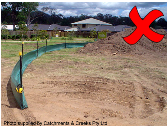
Post placed on wrong side of fence
