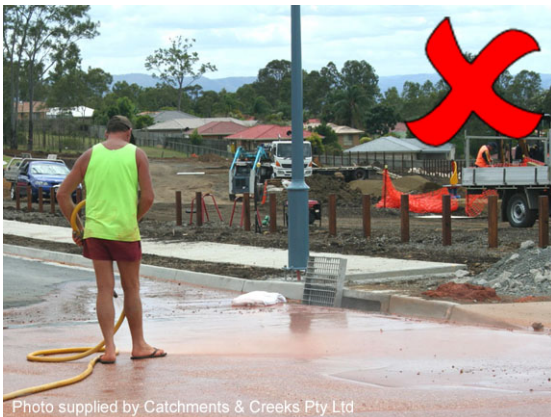
Poor maintenance practice
