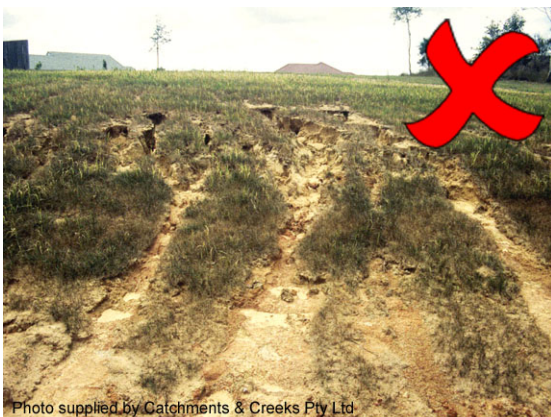
Erosion of recently seeded surface
