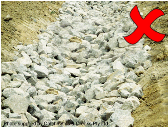
Poorly placed rock
