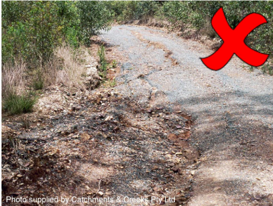
Inadequate drainage and erosion controls
