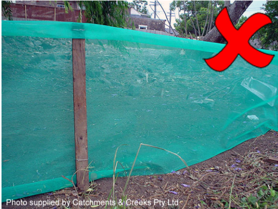
Inappropriate use of shade cloth
