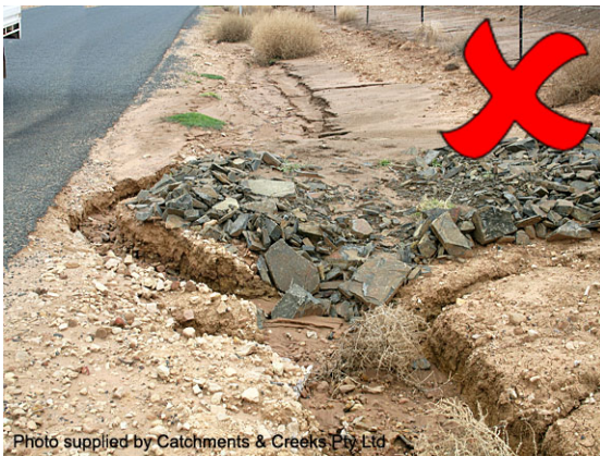
Failure of a check dam on a dispersive soil
