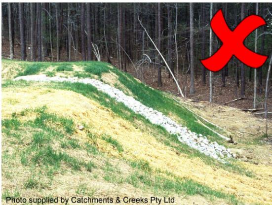
Insufficient scour protection at outlet
