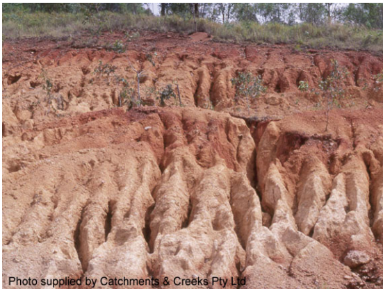
Erosion of a dispersive soil
