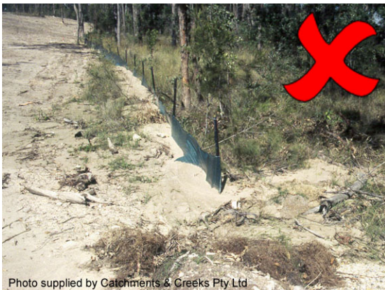
Fence not returned up-slope at end
