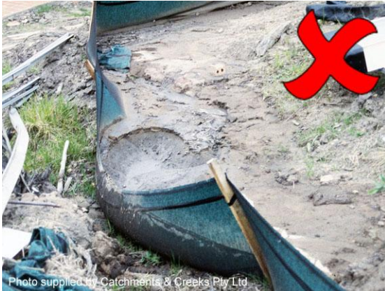
Sediment fence in need of maintenance
