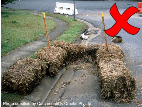
Potential traffic hazard
