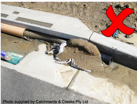
Sediment slowing washing into the inlet
