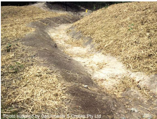
Loss of mulch by storm flows
