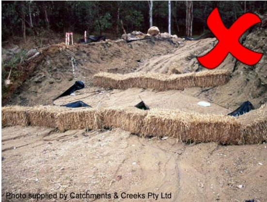
Inappropriate controls on a steep slope
