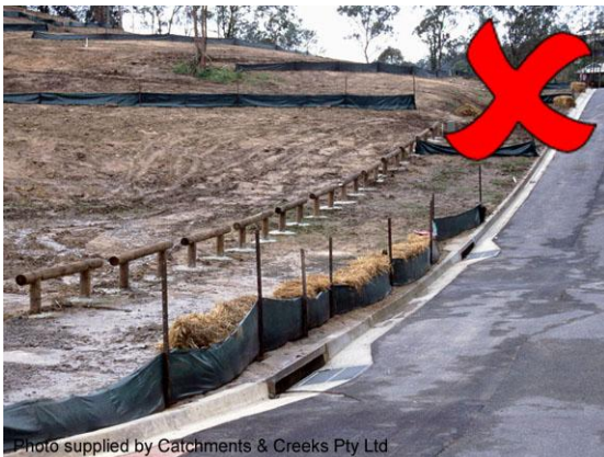
Inappropriate use of sediment fences
