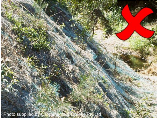
Misuse of synthetic blanket on creek bank
