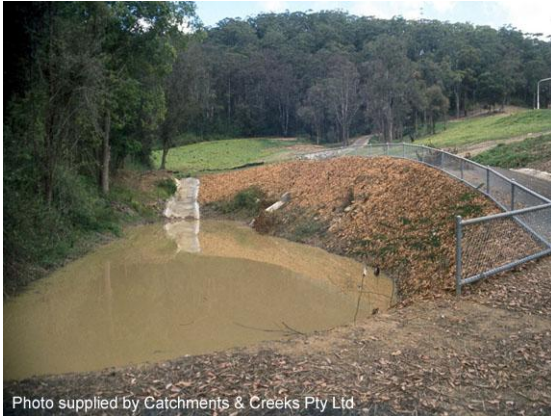
Basin with limited maintenance access
