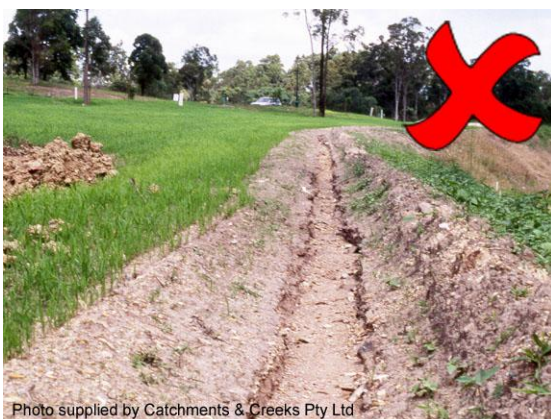
Erosion along channel invert
