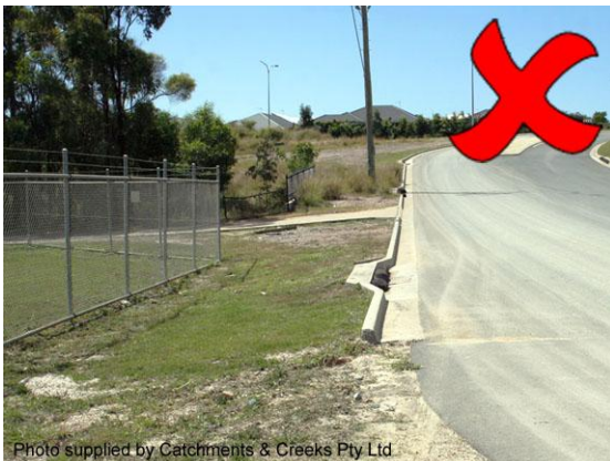
Sediment simply flows off the roadway
