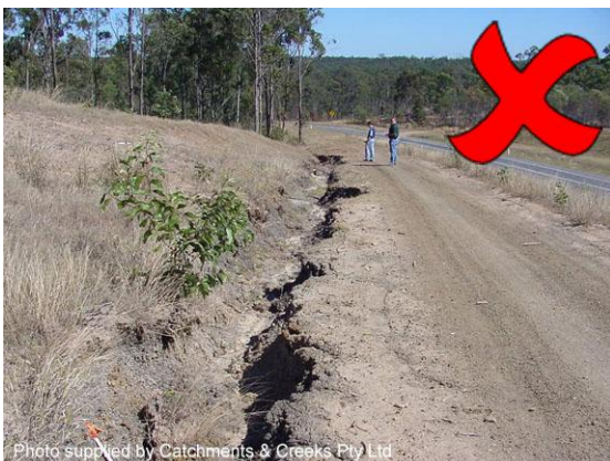
Batter drain cut into a dispersive soil
