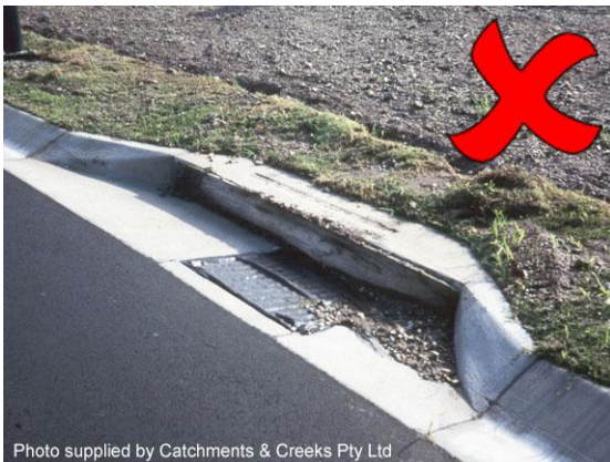
Fully blocked on-grade inlet
