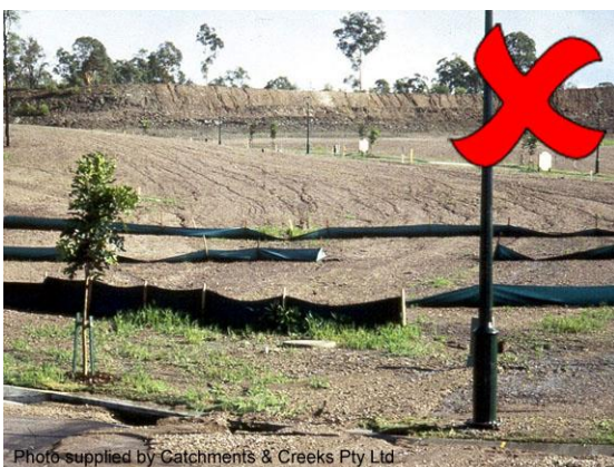
Inappropriate use of sediment fences
