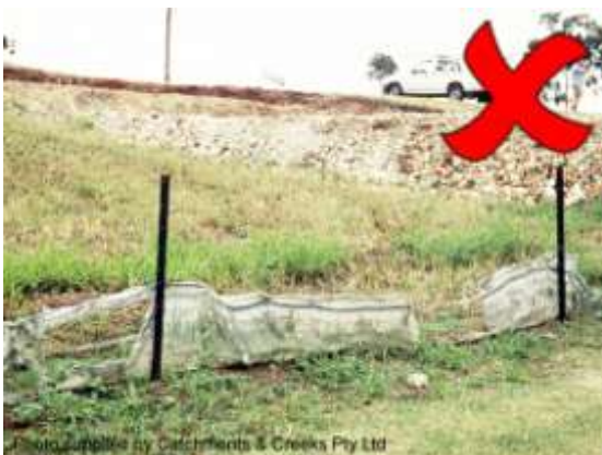
Sediment fence well past its 'use-by' date
