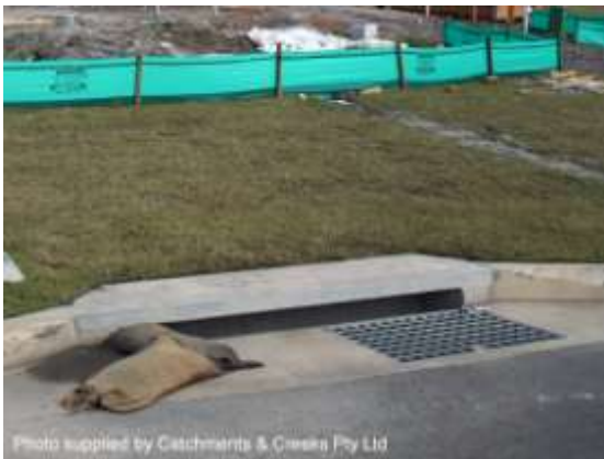
On-grade kerb inlet sediment trap
