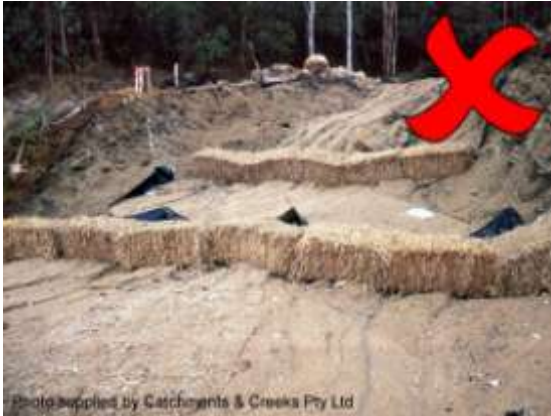
Inappropriate controls on a steep slope
