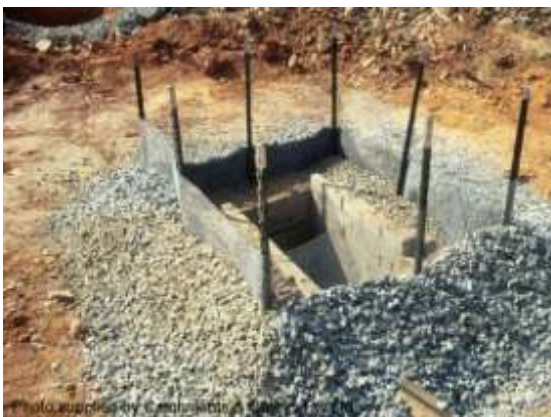
Mesh and aggregate drop inlet protection
