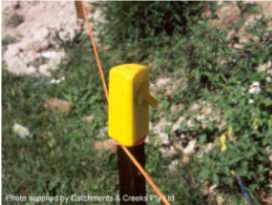
Safety cap on sediment fence stake
