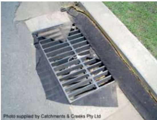
Gully bag sediment trap
