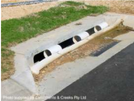
Photo supplied by Catchments & Creeks Pty Ltd Sag-type kerb inlet control system
