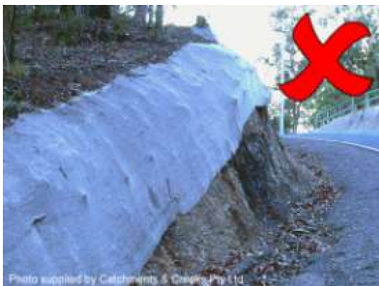
Poorly applied blanket
