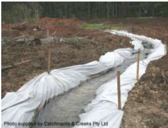
Clean water diversion drain
