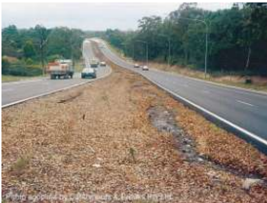
Loose mulch displaced by storms
