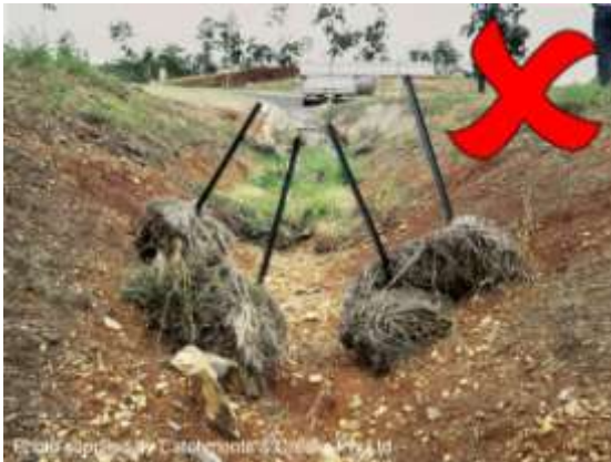
Failed straw bale sediment trap
