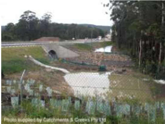
Post-construction sediment basins
