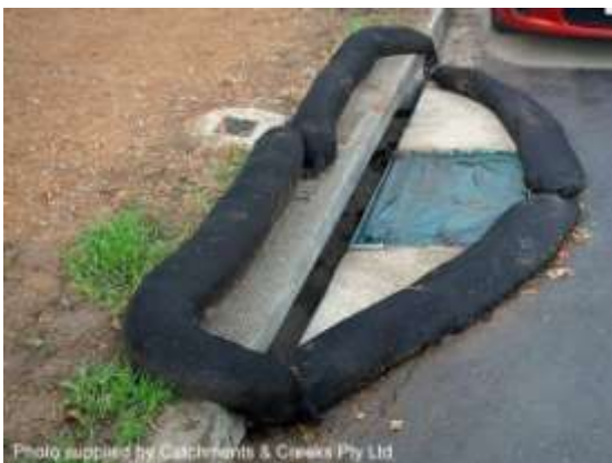
Sag inlet sediment trap
