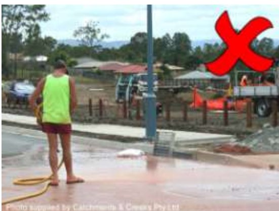
Inappropriate clean-up procedures
