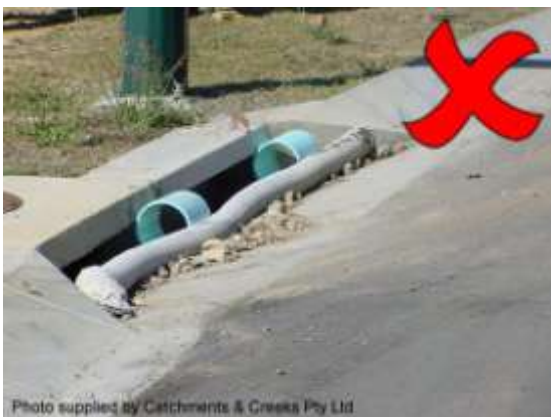
Common sense gone missing!
