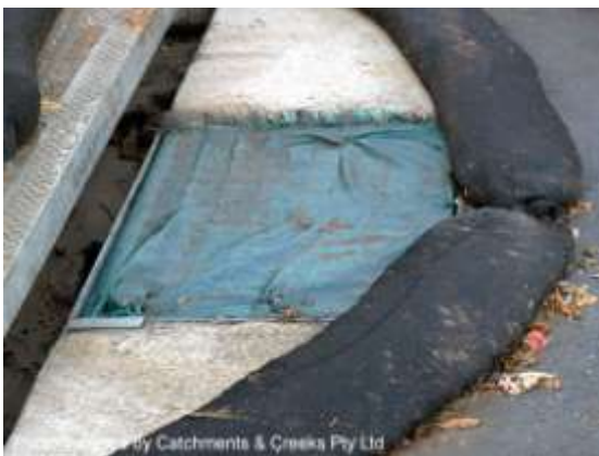
Inappropriate use of fabrics
