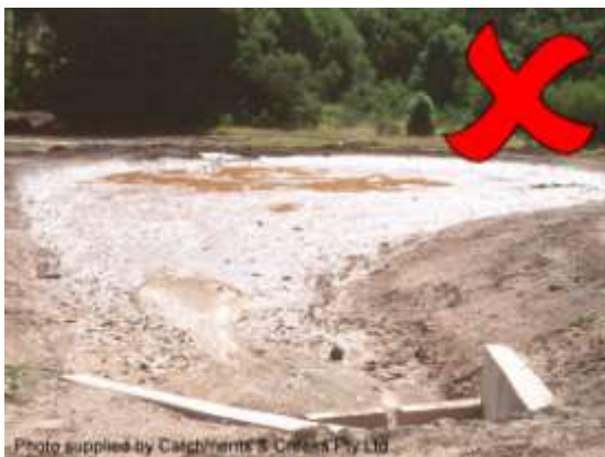
Undersized sediment basin
