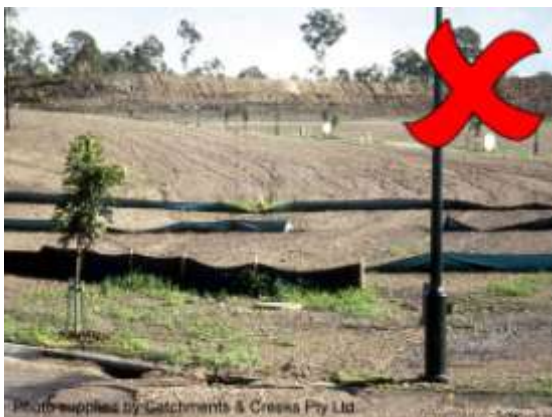
Inappropriate use of sediment fences
