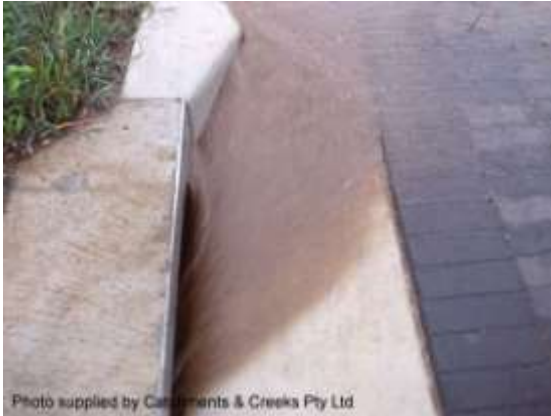
Sediment-laden runoff from work site
