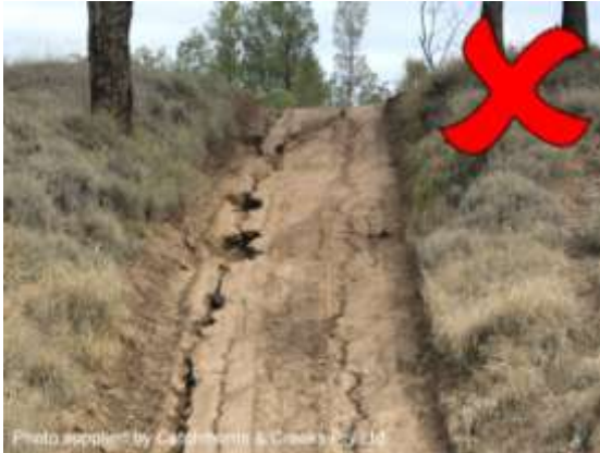
Drainage damage to an access road
