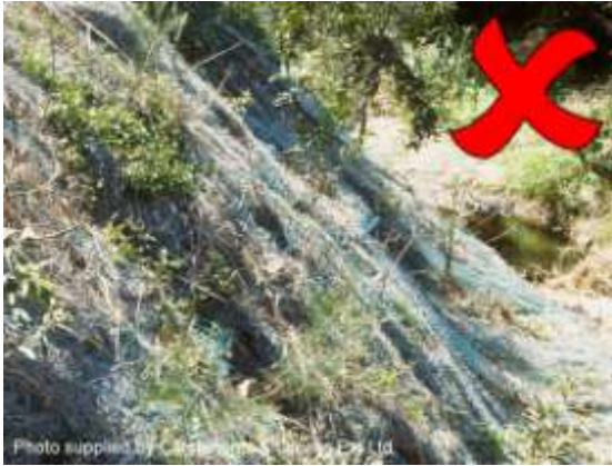
Misuse of synthetic blanket on creek bank
