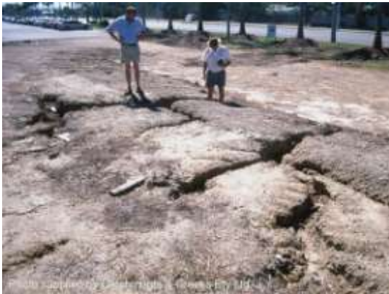
Inspecting storm damage
