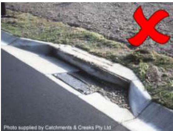
Fully blocked on-grade inlet
