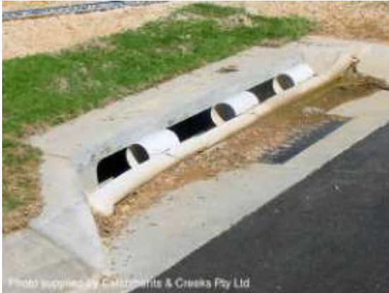
Sag inlet sediment trap
