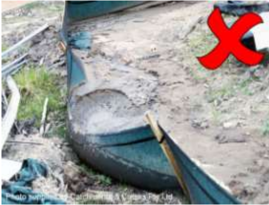
Sediment fence in need of maintenance
