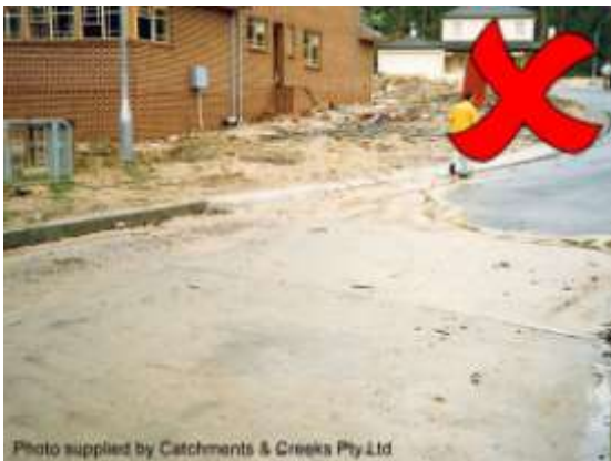
Sediment deposition on roadway
