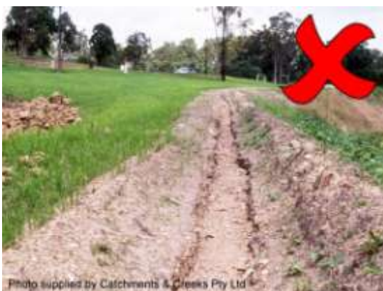
Erosion along channel invert
