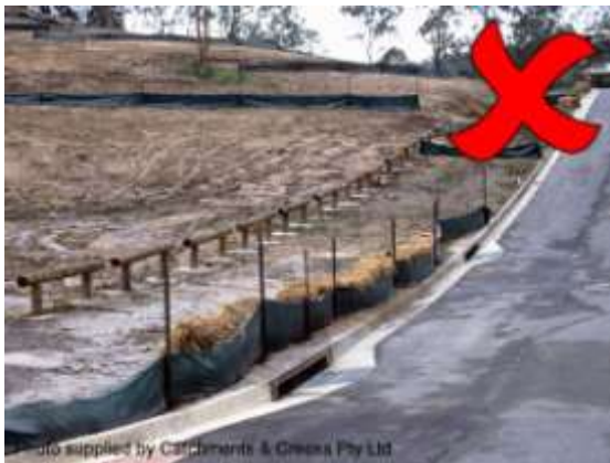
Inappropriate use of sediment fences
