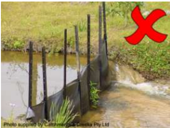
Poorly designed sediment trap
