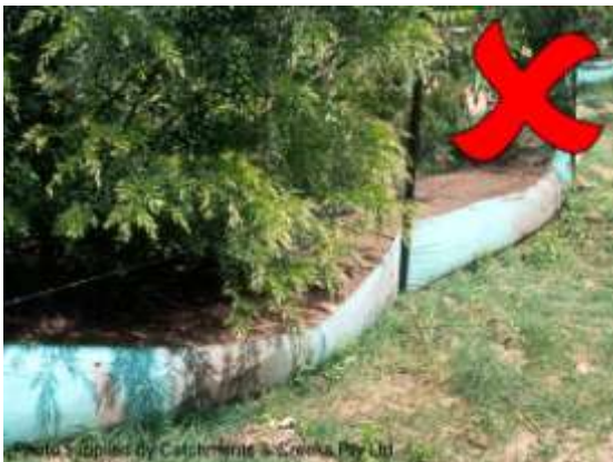
Sediment fence in need of maintenance
