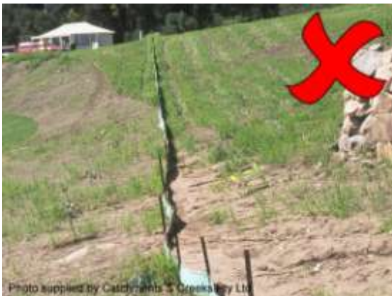
Inappropriate installation of a fence
