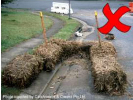
Potential traffic hazard
