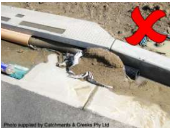
Sediment slowing washing into the inlet
