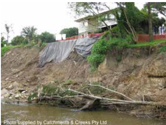
Creek bank failure
