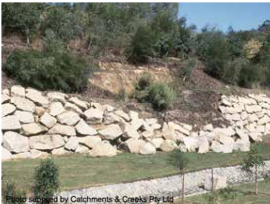
Failed rock retaining wall
