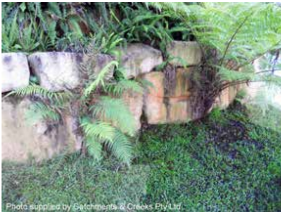
Groundwater weeping from retaining wall
