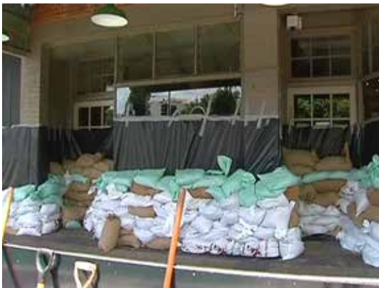
Flood-proofing of low-level building
