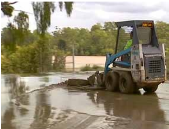
Post flood clean-up
