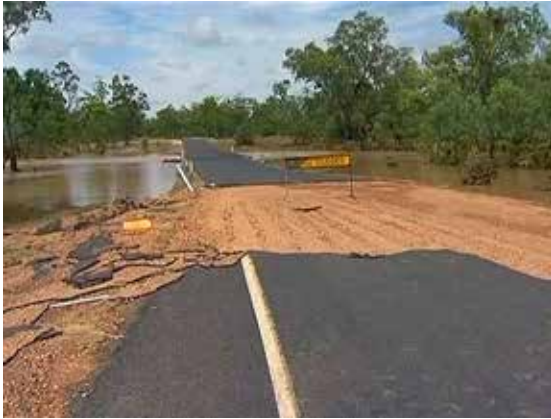
Asphalt lifted from roadway
