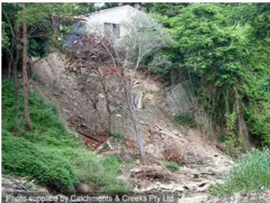
Bank erosion on outside of channel bend
