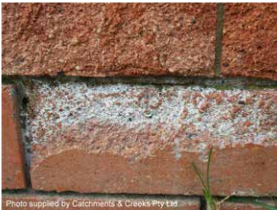
Salt damage to brickwork
