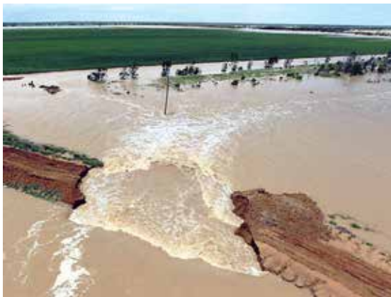
Failure of earth embankment
