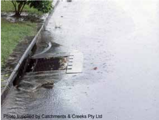
Roadside kerb inlet to stormwater pipe
