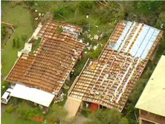
Storm damage to roofs
