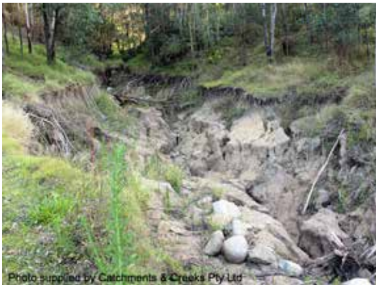
Gully erosion up-slope of a new home
