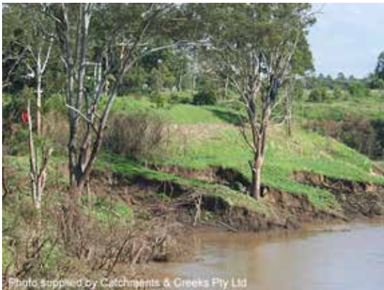
Bank slumping downstream of a dam
