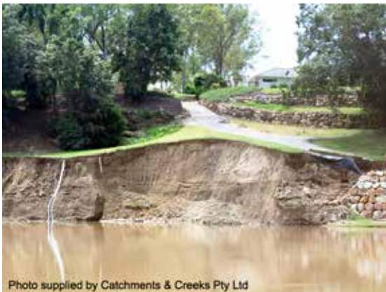
Landslip following river flooding
