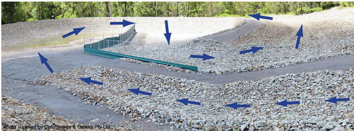
Internal flow control baffle on a quarry site (Qld)
