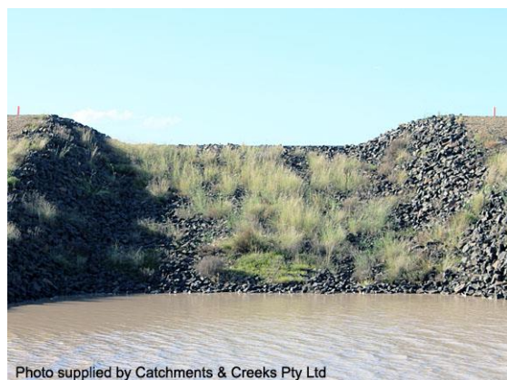
Energy dissipation pond (Qld)
