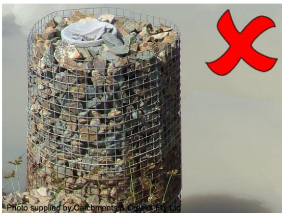
Gabion riser without fabric wrap
