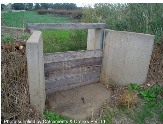
'Stop-board' outlet control system (SA)
