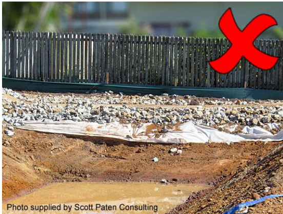
Spillway aimed at neighbour's fence
