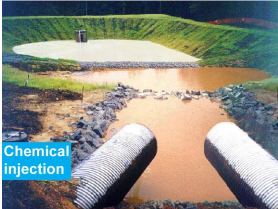
Chemical injection and mixing
