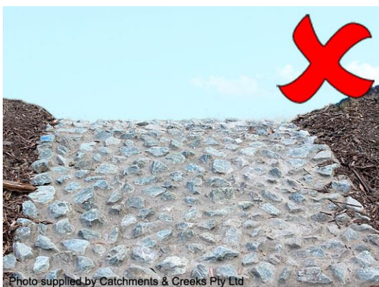
Spillway chute with not side walls!
