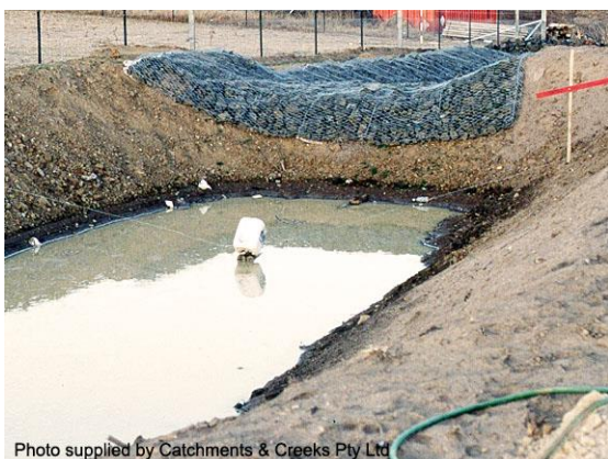
Rock mattress spillway (NSW)
