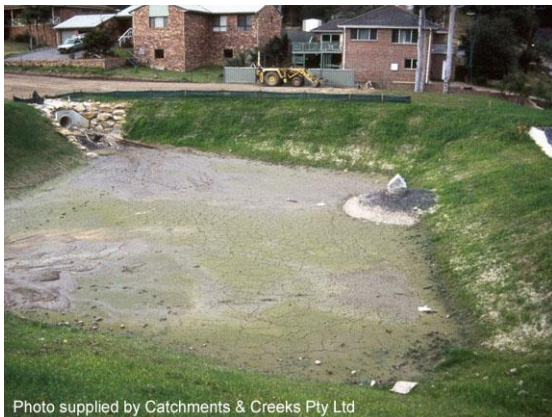
Type C sediment basin (NSW)
