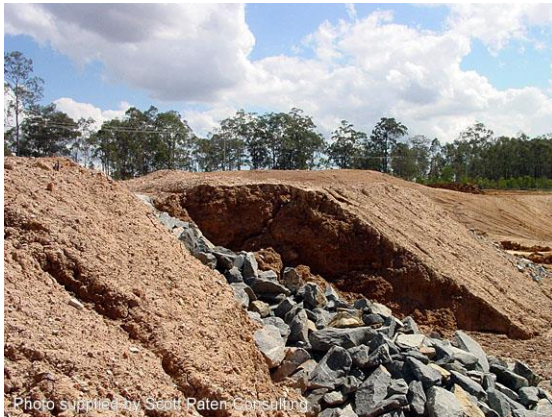
Failed sediment basin spillway
