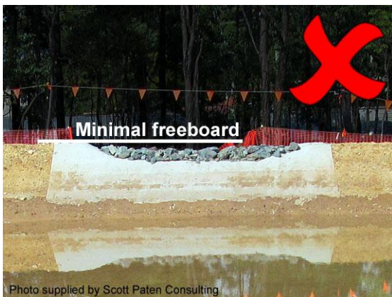
Spillway with insufficient freeboard
