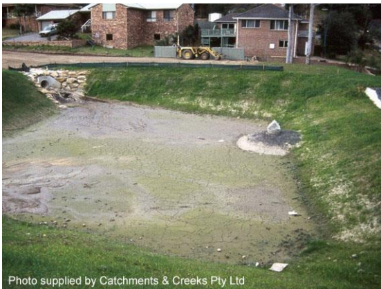
Type C sediment basin (NSW)
