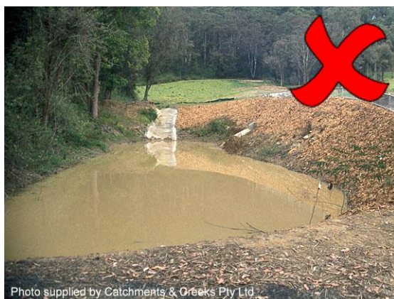
Limited access for basin de-silting
