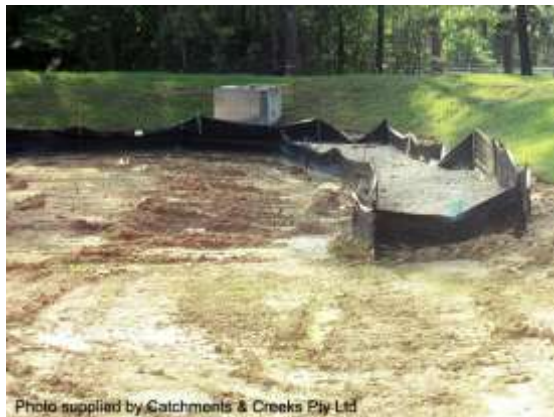
Sand filter surrounded by sed-fence (USA)
