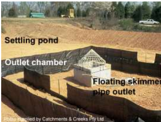
Skimmer pipe inside an outlet chamber
