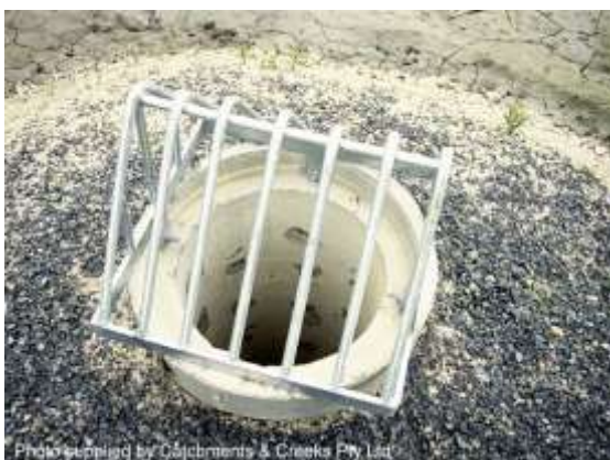
Riser pipe with aggregate filter (NSW)
