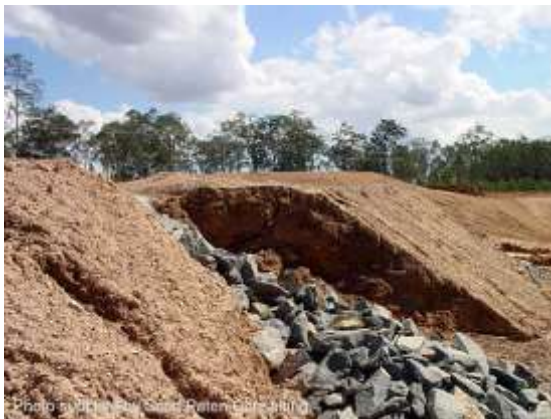
Failed sediment basin spillway
