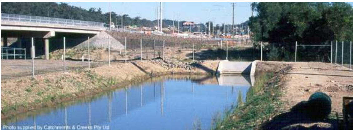
Type D sediment basin retained for permanent stormwater treatment (Qld)
