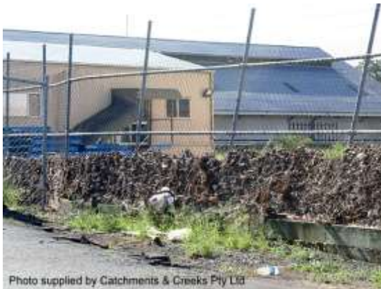
Debris blockage of a property fence (Qld)
