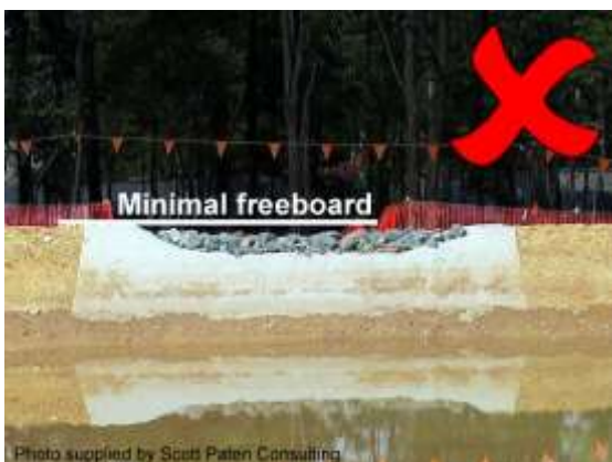
Spillway with insufficient freeboard
