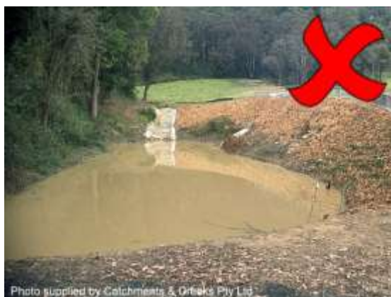
Limited access for basin de-silting
