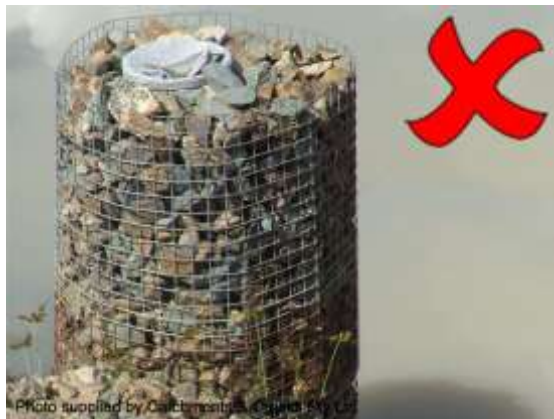
Gabion riser without fabric wrap
