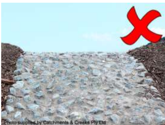
Spillway chute with not side walls!
