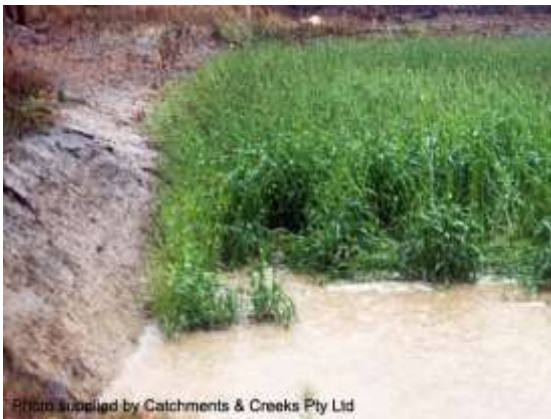
Very steep and slippery bank slope (Qld)
