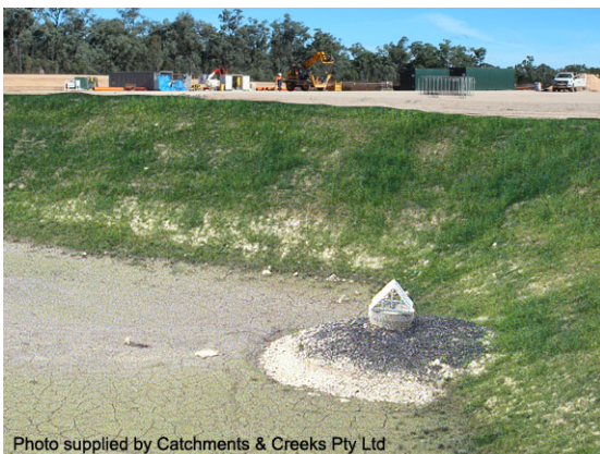
Riser pipe decant
