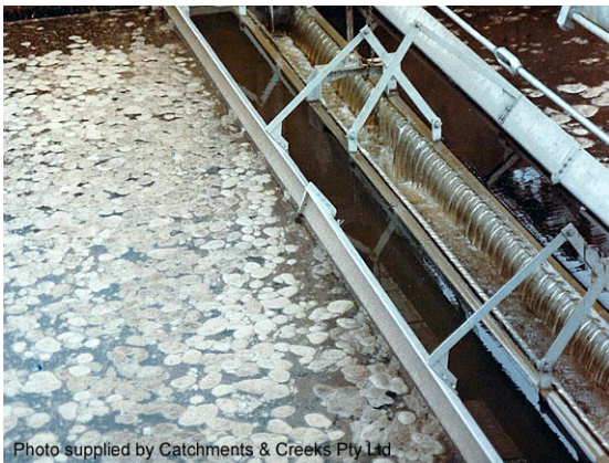
Bathurst Box decant trough
