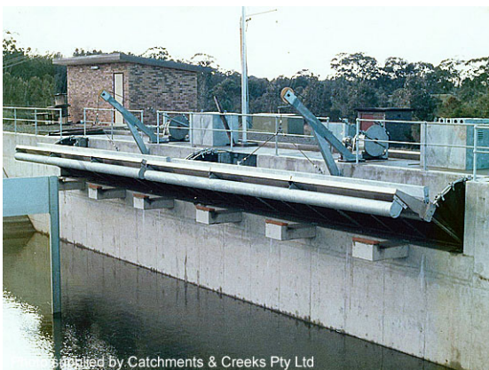
Floating decant system with slow fall
