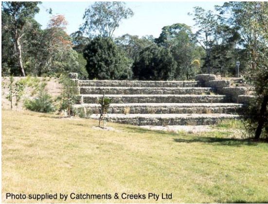
Photo 3 – Permanent, gabion-lined stepped spillway located on a detention basin
