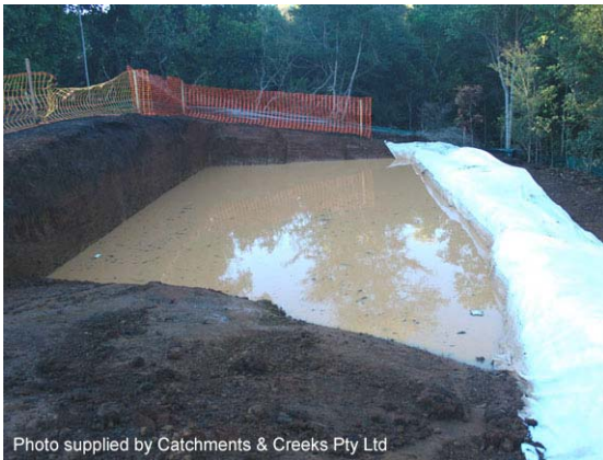
Photo 5 – Recessing the basin into the ground allows the natural ground level to become the spillway
