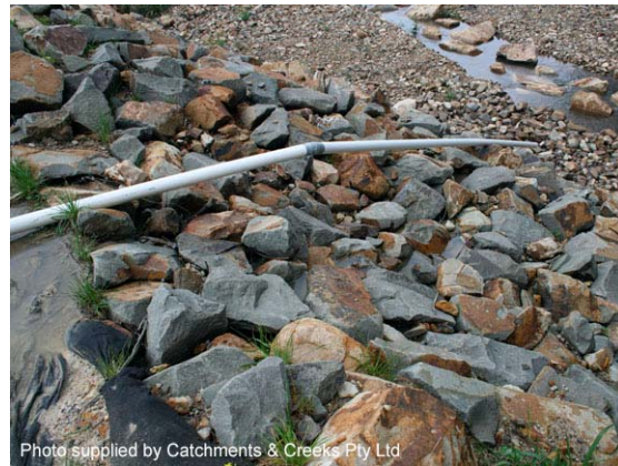
Photo 6 – Spillways lined with loose rock generally have a high risk of failure compared to concrete and rock mattress linings
