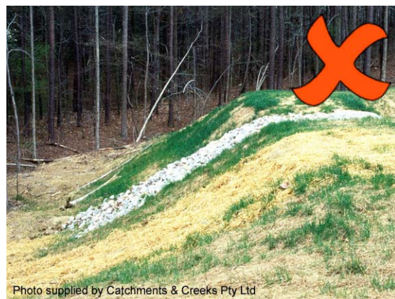
Photo 8 – A suitable energy dissipater must exist at the base of the spillway
