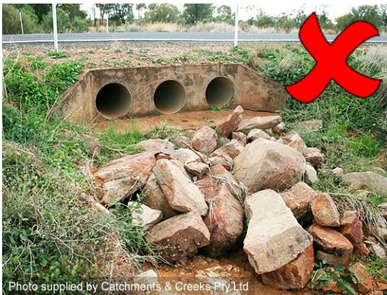
Inappropriate rock placement
