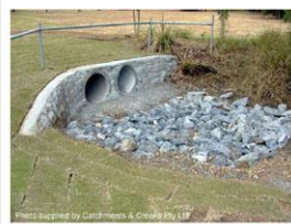
Photo 1 – Rock pad outlet structure at end of a dual stormwater pipe outlet
