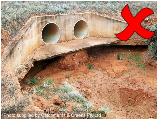
Undermining of culvert
