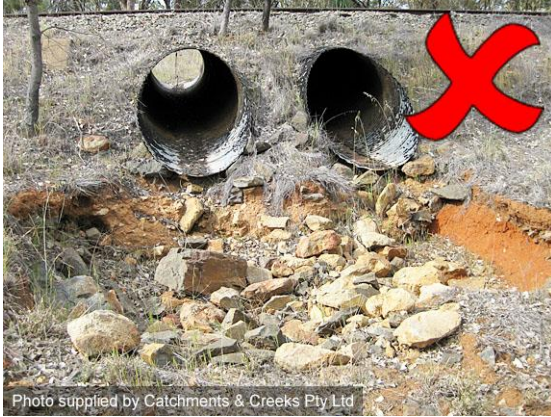
Displacement of rock pad
