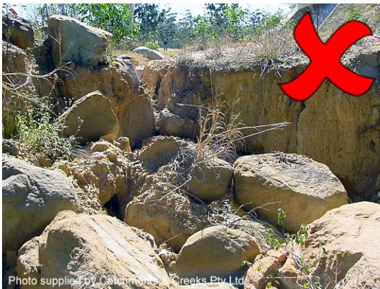
Collapsed dispersive soil bank
