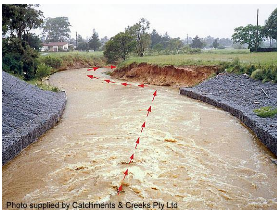
Bank erosion well downstream of culvert
