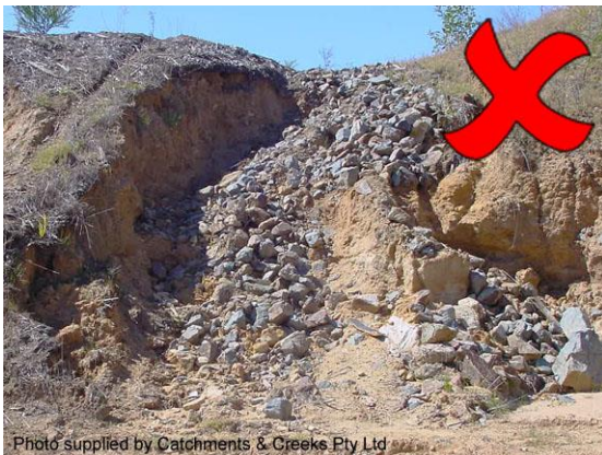
Failure of rock-lined batter chute
