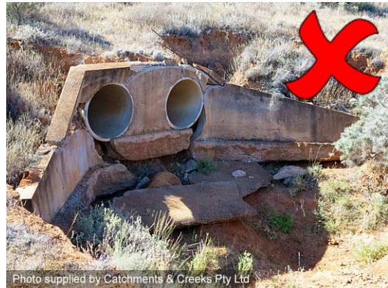
Same culvert outlet eight years later
