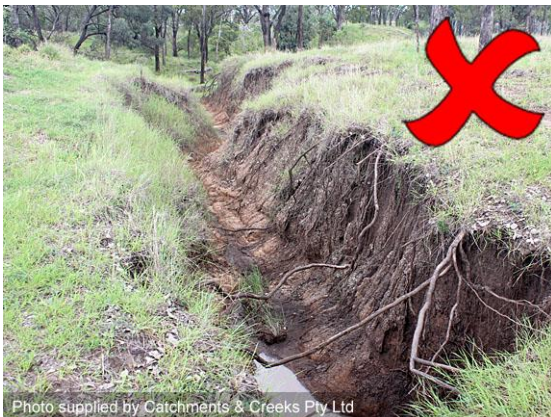
Erosion of a dam's bywash (spillway)
