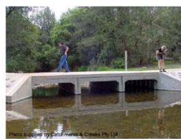
Photo 1 – Fish-friendly box culvert with roughened bed conditions
