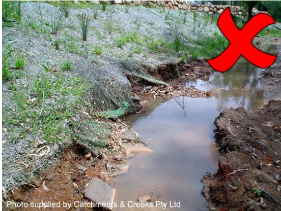
Erosion along toe of bank
