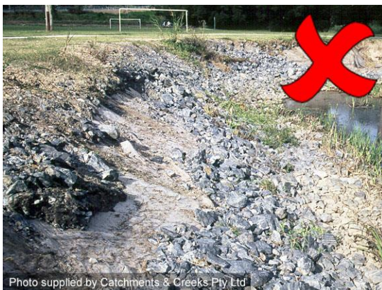
Rocks displaced down filter cloth
