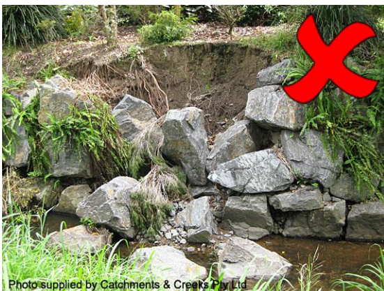
Failed boulder wall
