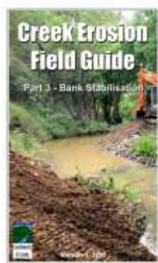
Creek Erosion, parts 1, 2, 3 & 4
