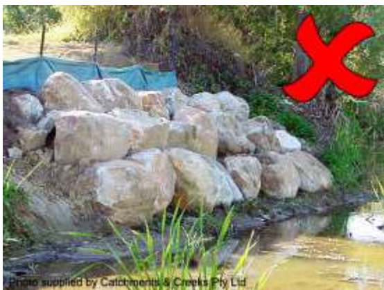
Poorly placed rocks on creek bank
