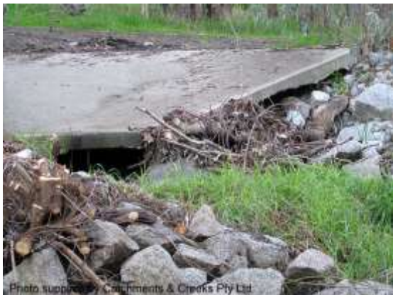
Photo supplied by Catchments & Creeks Pty Ltd Rock displaced at end of concrete channel
