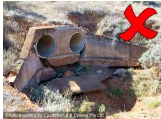
Same culvert outlet eight years later
