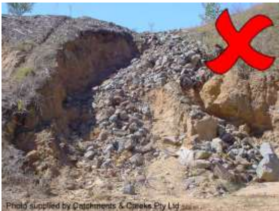
Failure of rock-lined batter chute
