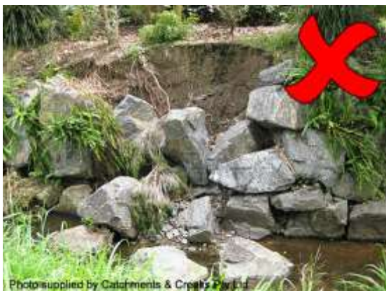
Failed boulder wall
