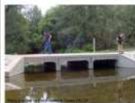
Photo 1 – Fish-friendly box culvert with roughened bed conditions
