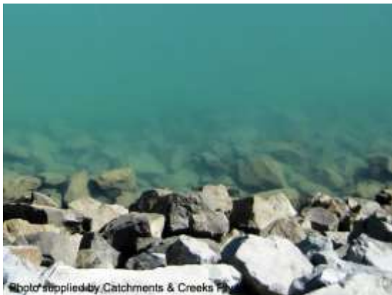
Open voids below permanent waterline
