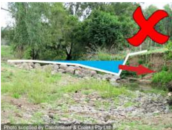
Flows spill unevenly over the rock weir
