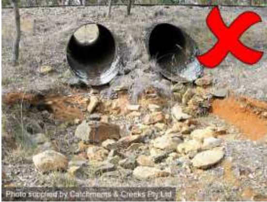
Displacement of rock pad
