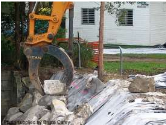
Photo supplied by Bruce Carey Rocks placed over a geotextile filter (Qld)
