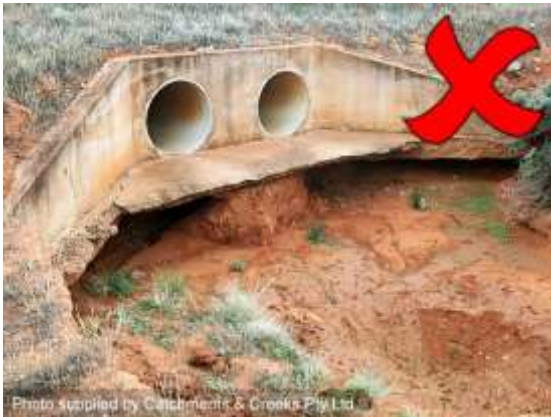
Undermining of culvert
