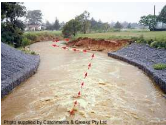
Bank erosion well downstream of culvert
