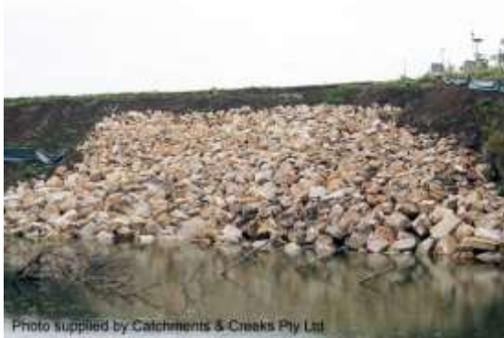
Poor aesthetics without vegetation cover
