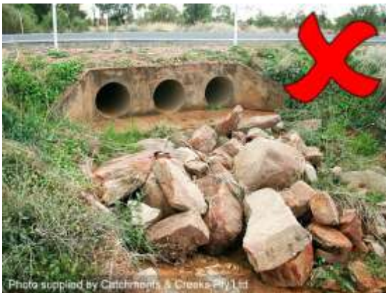
Inappropriate rock placement
