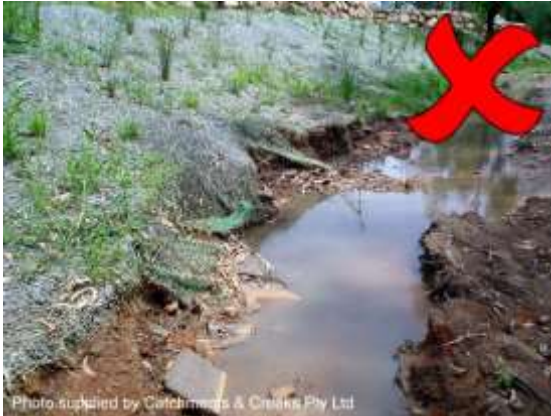
Erosion along toe of bank
