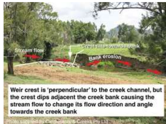
Bank erosion produced from weir (left)
