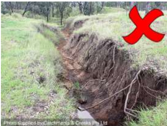
Erosion of a dam's bywash (spillway)
