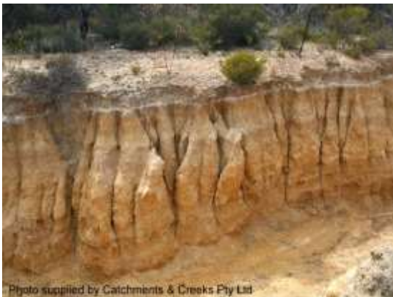
Fluting erosion in a dispersive soil (SA)
