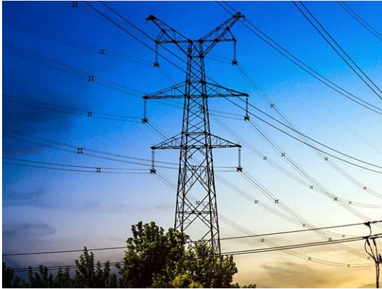
Electrical power lines
