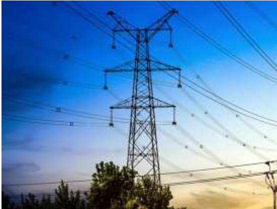
Electrical power lines
