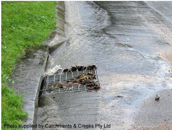
Roadside kerb drainage
