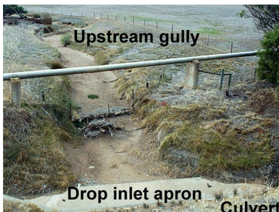
Gully erosion upstream of a drop inlet
