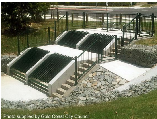
Complex inlet screen (Gold Coast, Qld)
