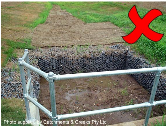
Drop inlet with no raised weir
