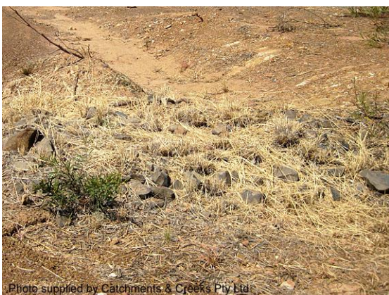
Recessed rock check dam (NT)
