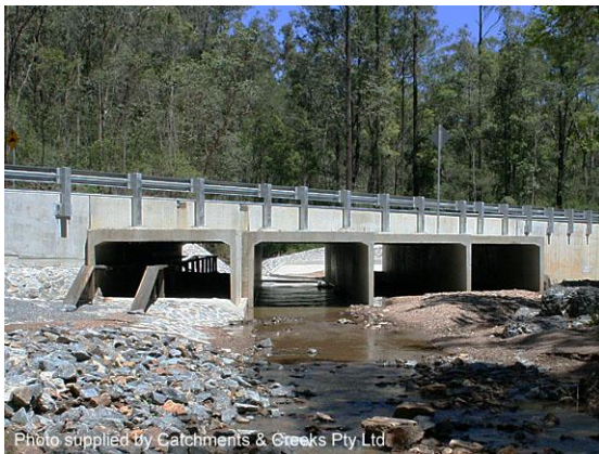
Dry cells set just above base flow level
