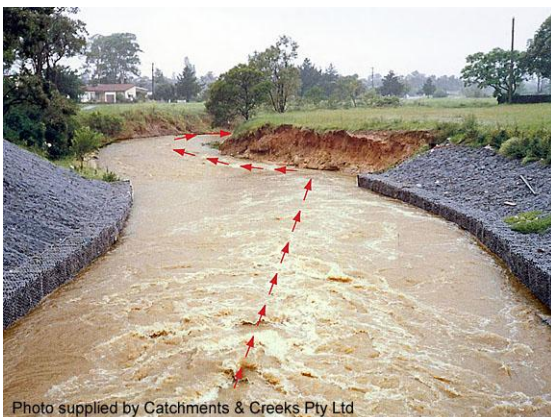
Bank erosion well-downstream of culvert
