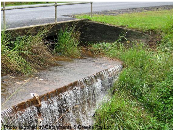
Culvert with apron but no cut-off wall
