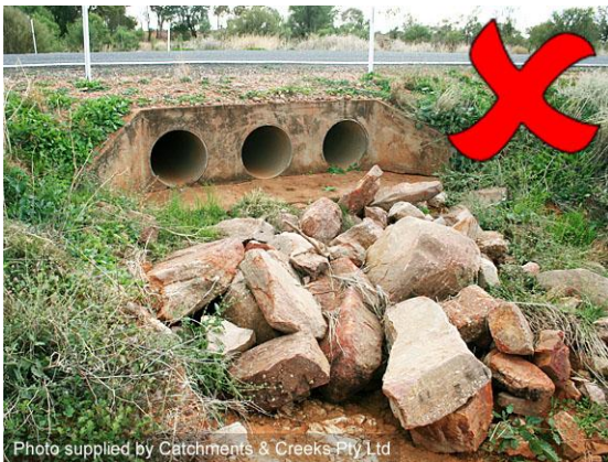
Inappropriate rock placement
