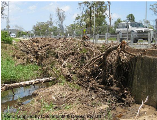
100% blockage of a road culvert (Qld)
