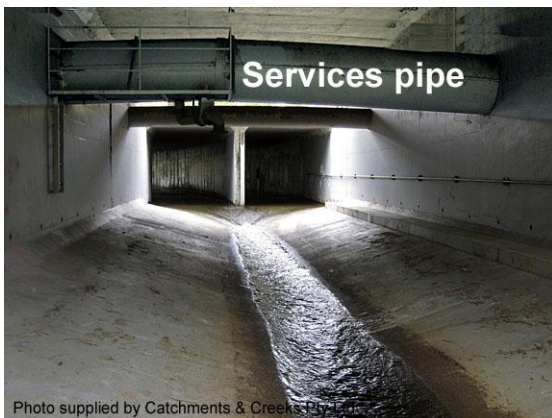
Culvert with exposed services (Qld)
