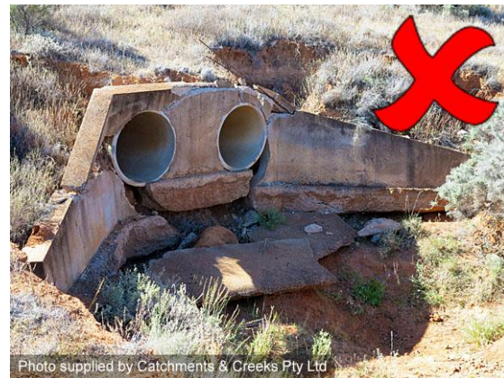
Same culvert outlet eight years later
