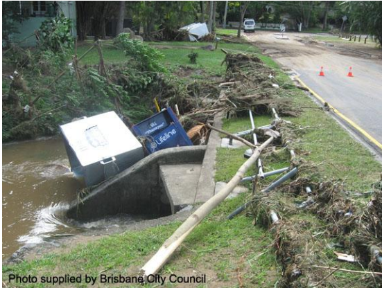
Culvert blocked by flood debris (Qld)
