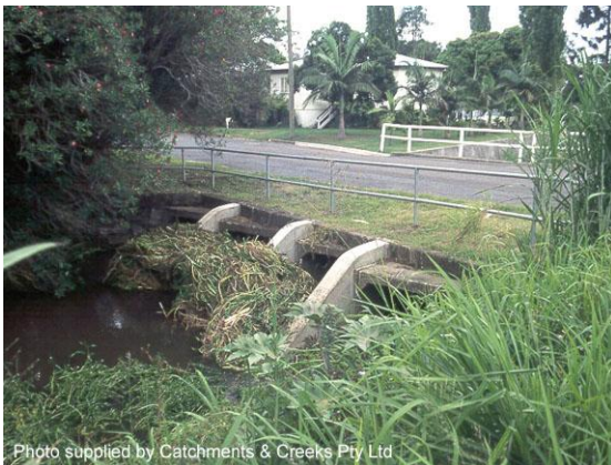
Post-flood condition, 1995 (Qld)
