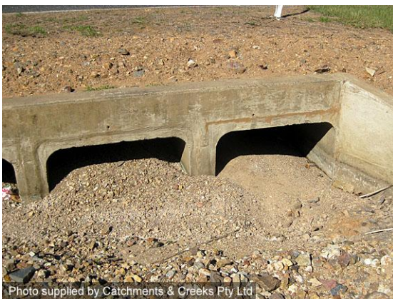
Partial sediment blockage of a culvert
