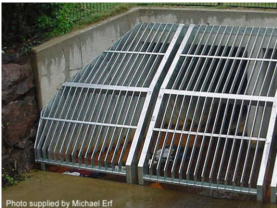
Parabolic inlet screen (Qld)
