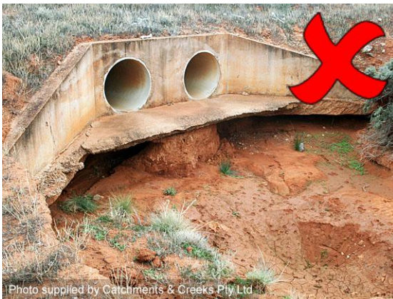
Undermining of culvert
