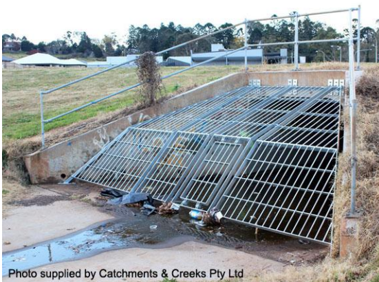
Parabolic inlet screen (Qld)
