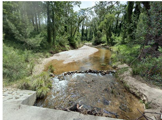
Inlet riffle washed away (2022)
