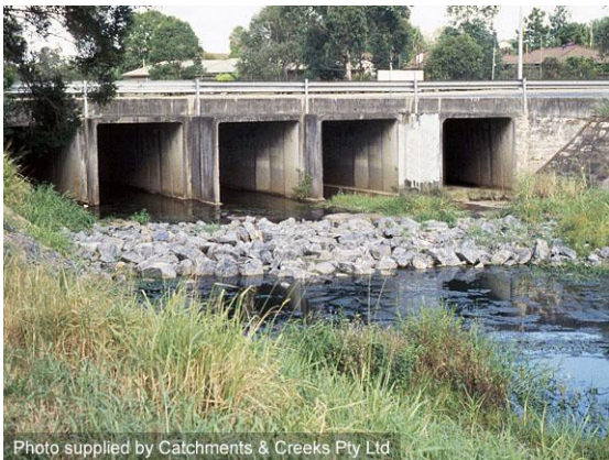
Rock pad outlet (Qld)
