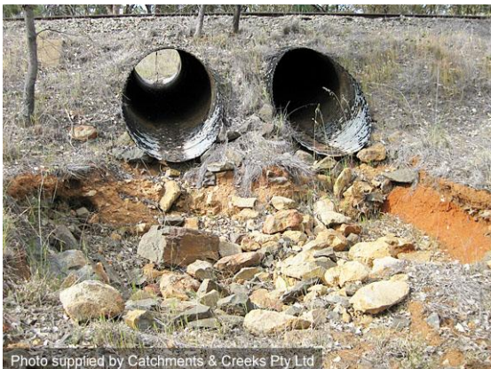
Outlet bed erosion (SA)
