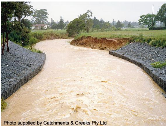
Outlet jetting during high tailwater (NSW)
