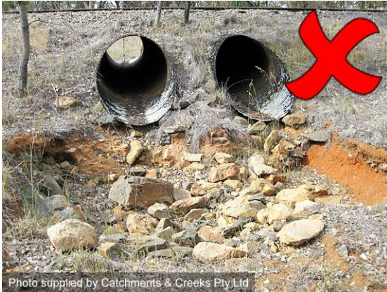
Displacement of rock pad
