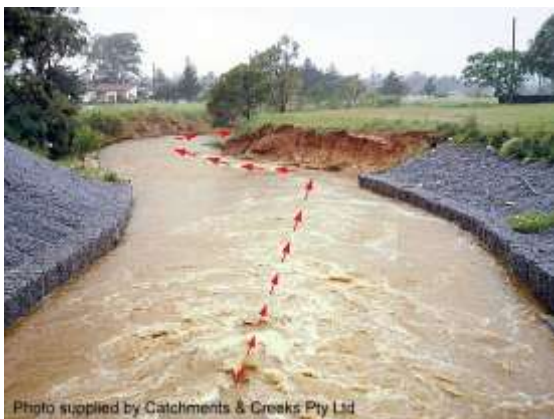
Bank erosion well-downstream of culvert
