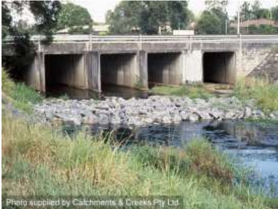
Rock pad outlet (Qld)
