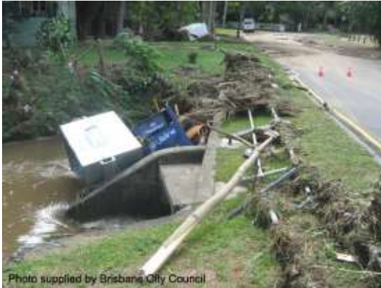
Culvert blocked by flood debris (Qld)
