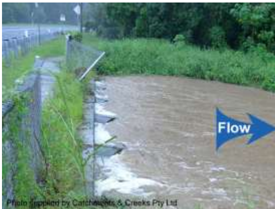
Drowned outlet conditions (full culvert)
