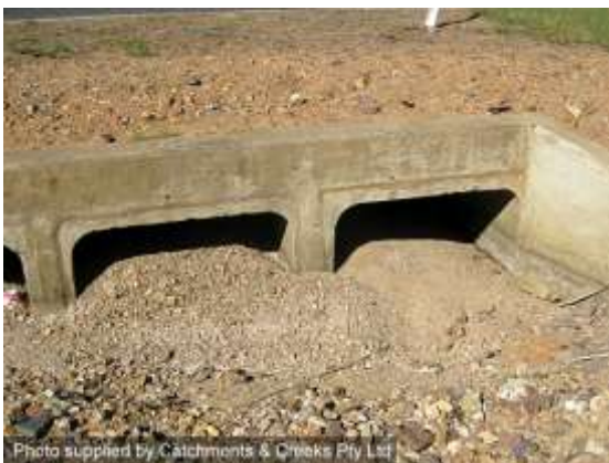
Partial sediment blockage of a culvert
