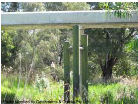
Debris impact pole (SA)
