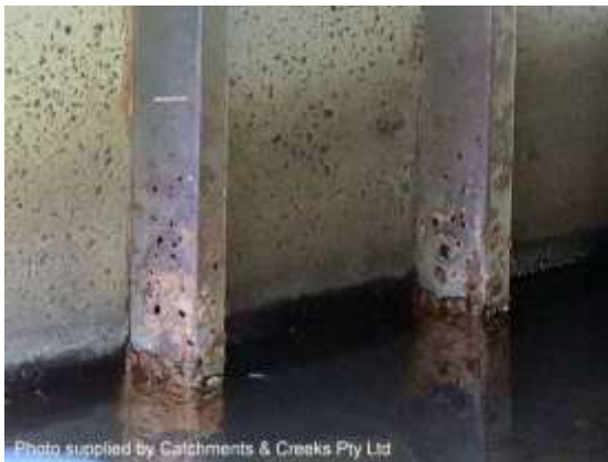
Rusted galvanised steel baffles (NSW)
