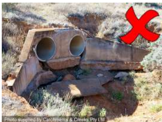
Same culvert outlet eight years later
