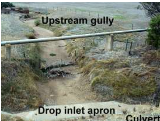
Gully erosion upstream of a drop inlet
