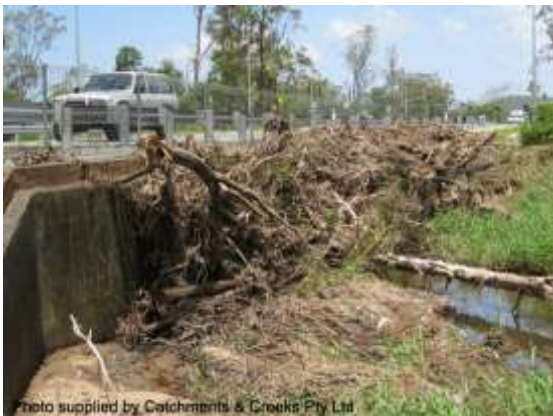
100% debris blockage (Qld)
