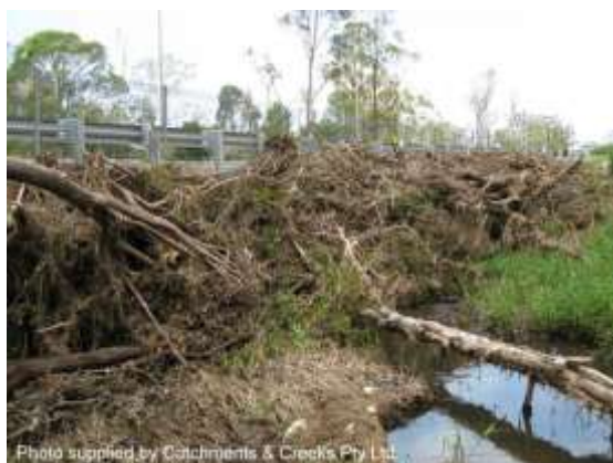
Culvert fully blocked by flood debris (Qld)
