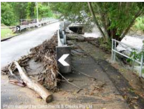
Debris blockage of traffic barrier (Qld)
