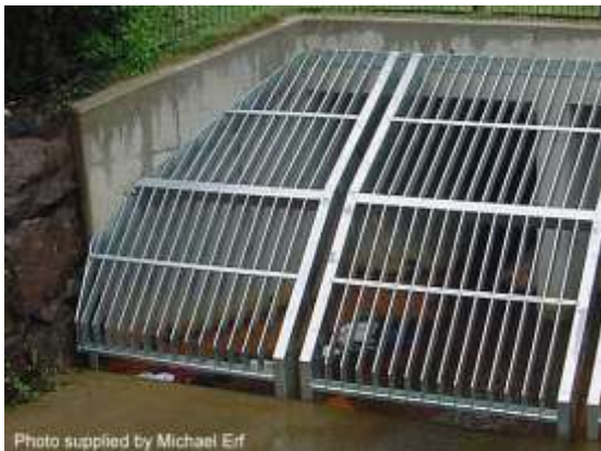
Parabolic inlet screen (Qld)
