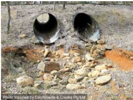
Outlet bed erosion (SA)
