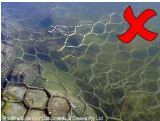
Damaged wire mesh
