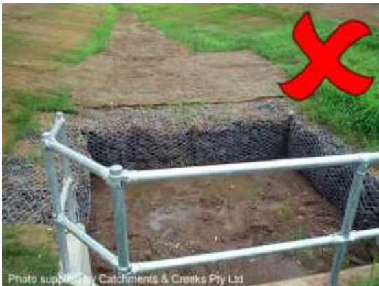
Drop inlet with no raised weir
