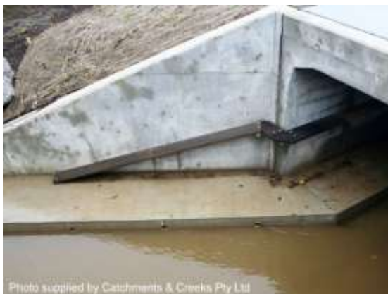
Box culvert with terrestrial pathways (Qld)
