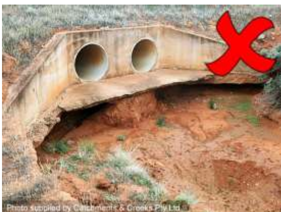
Undermining of culvert
