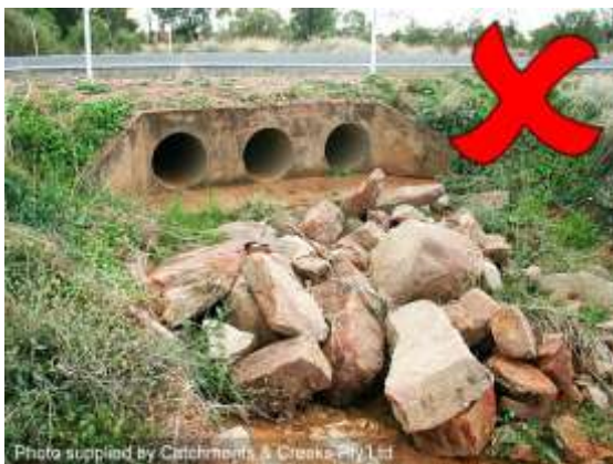
Inappropriate rock placement
