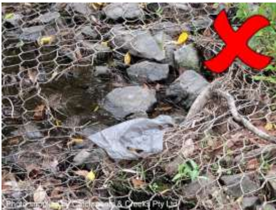
Wire mesh ripped open
