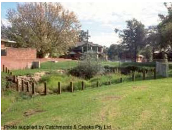
Safety poles (NSW)
