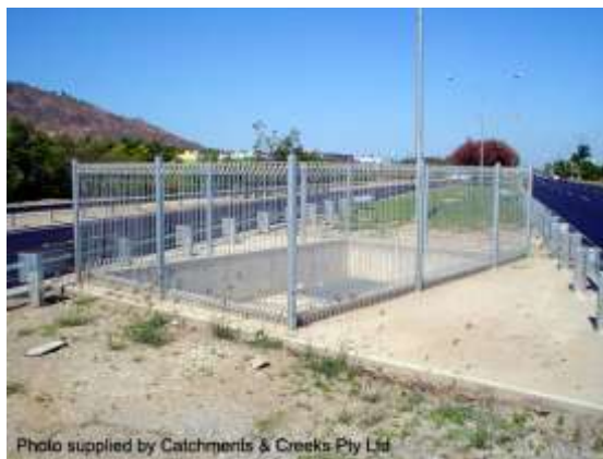
Skylights placed within the median (Qld)
