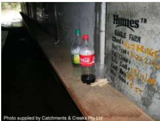
Evidence of human activity in the culvert
