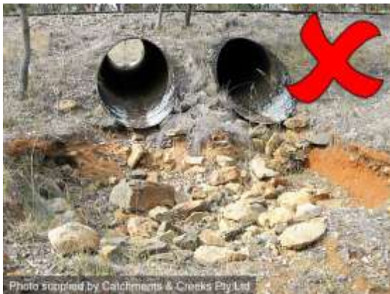
Displacement of rock pad
