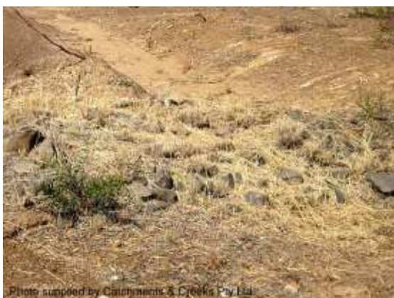
Recessed rock check dam (NT)
