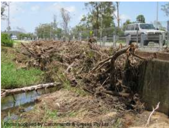
100% blockage of a road culvert (Qld)
