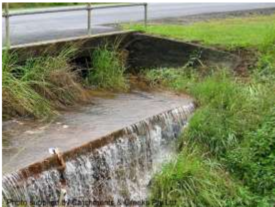
Culvert with apron but no cut-off wall
