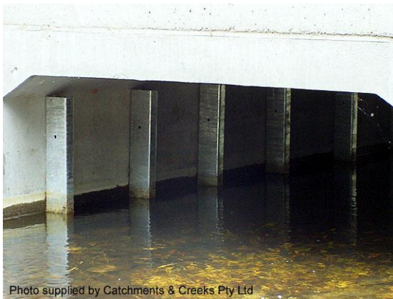
Channel-section baffles (NSW)
