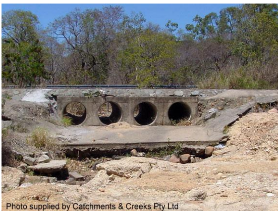
Bed level falling downstream of culvert
