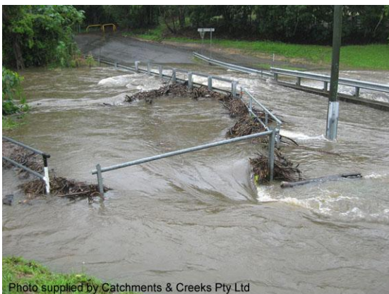
Overtopping flood event
