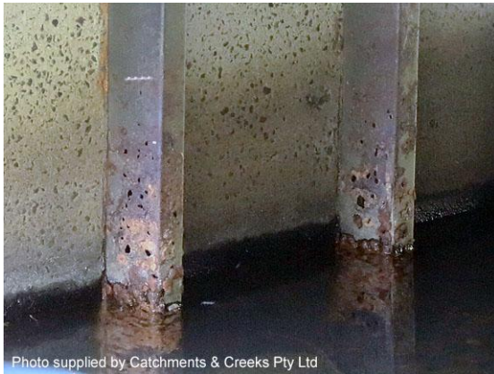
Galvanised steel (rusting)
