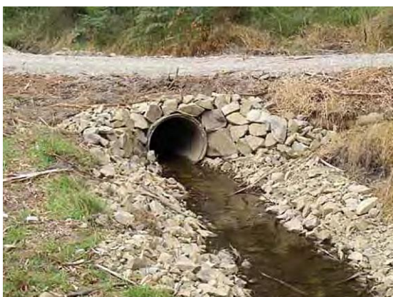
Stock crossing (Melbourne Water)
