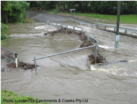
Drowned-out culvert structure
