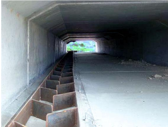
Floor baffle (Oodnadatta Track, SA)
