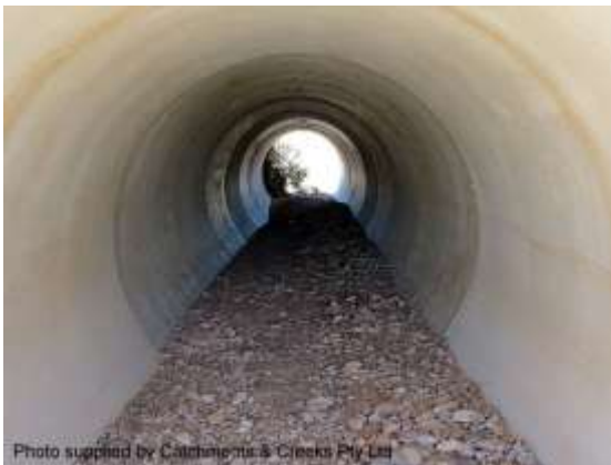
Deposition of sediments in a pipe culvert
