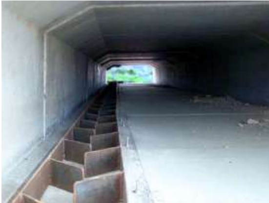
Floor baffle (Oodnadatta Track, SA)
