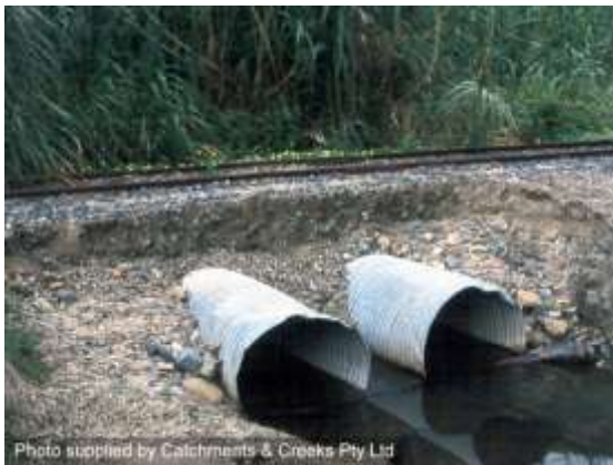
Erosion by overtopping flows
