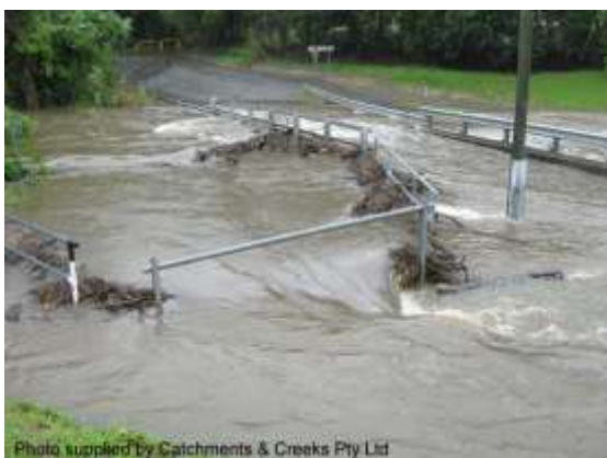
Drowned-out culvert structure
