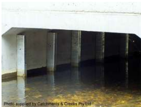
Channel-section baffles (NSW)
