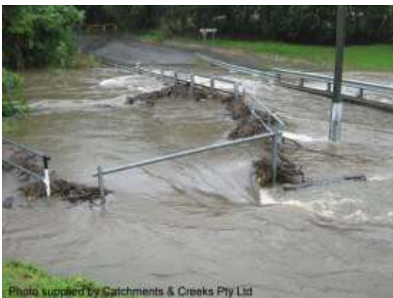
Overtopping flood event
