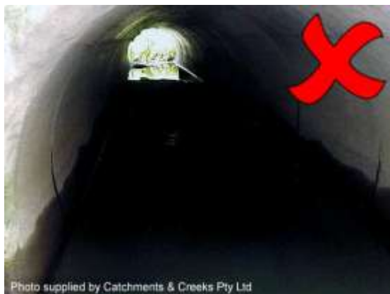
Poor lighting conditions
