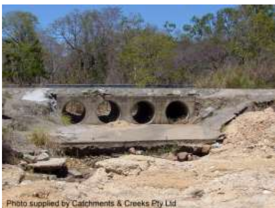
Bed level falling downstream of culvert
