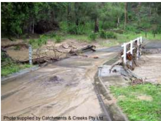
Flood damage to waterway crossing (Qld)
