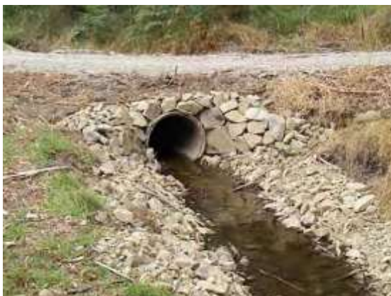
Stock crossing (Melbourne Water)
