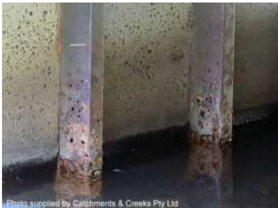
Rusted galvanised steel baffles (NSW)
