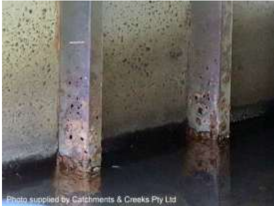
Galvanised steel (rusting)
